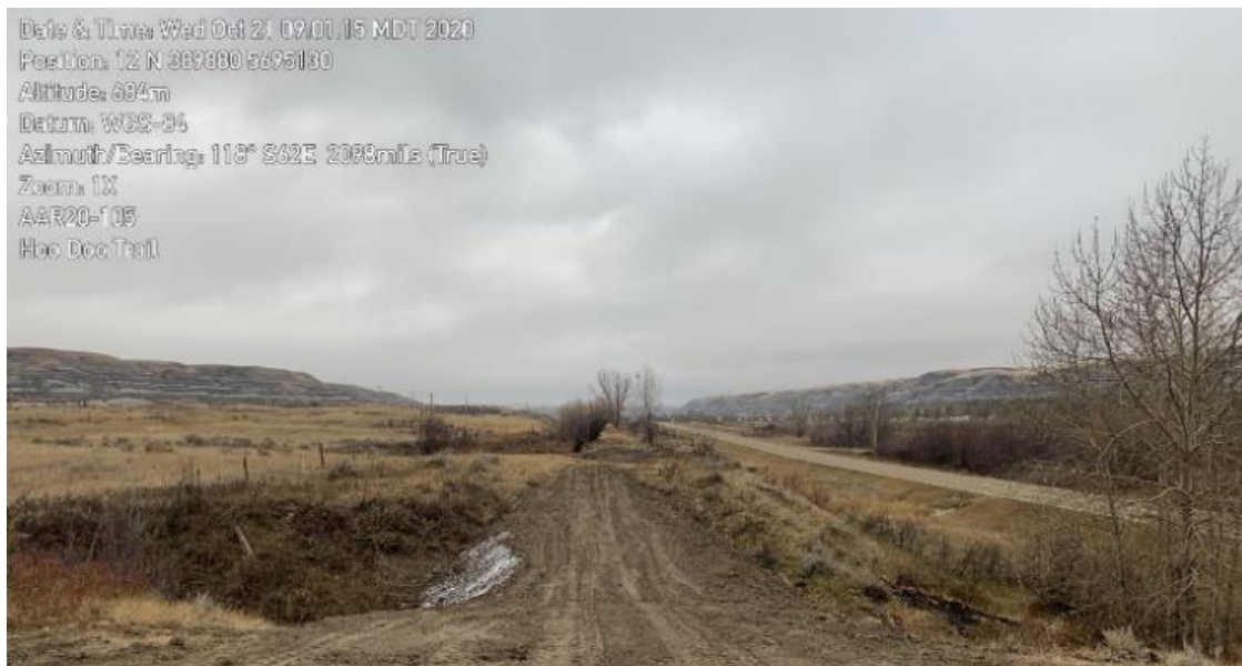
Plate 8. Hoodoos Trail. Recent vegetation clearing, stripping topsoil and culvert installation were recorded along the route (October 21, 2020).
