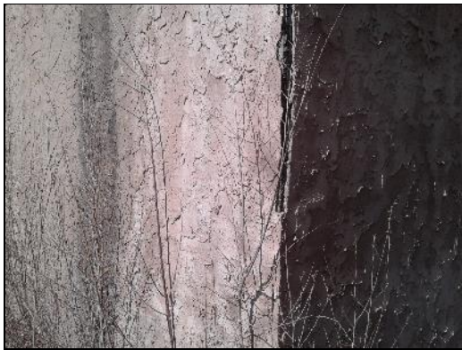
Non-lead based pink paint (sample L0001) on the stucco Exterior (location 1).
