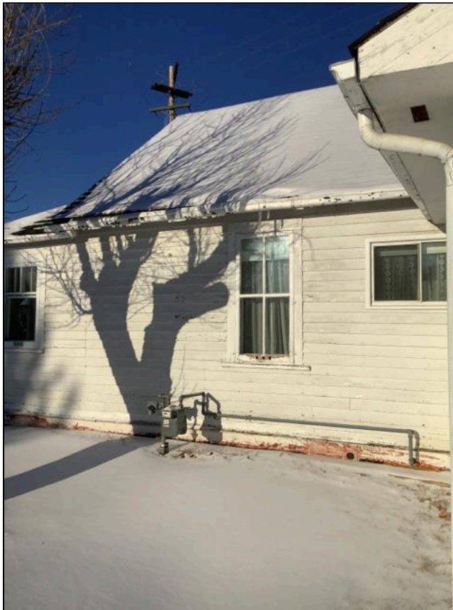
3.1 Item 3(Picture) Exterior - siding requires prep and paint
