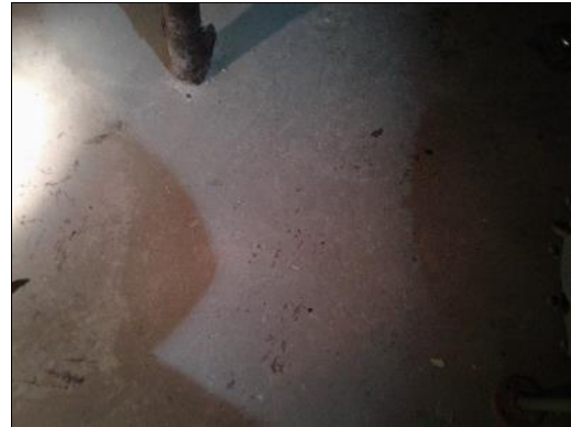
Lead-based grey paint (sample L0006) on the concrete floor in the Generator Room (location 25).
