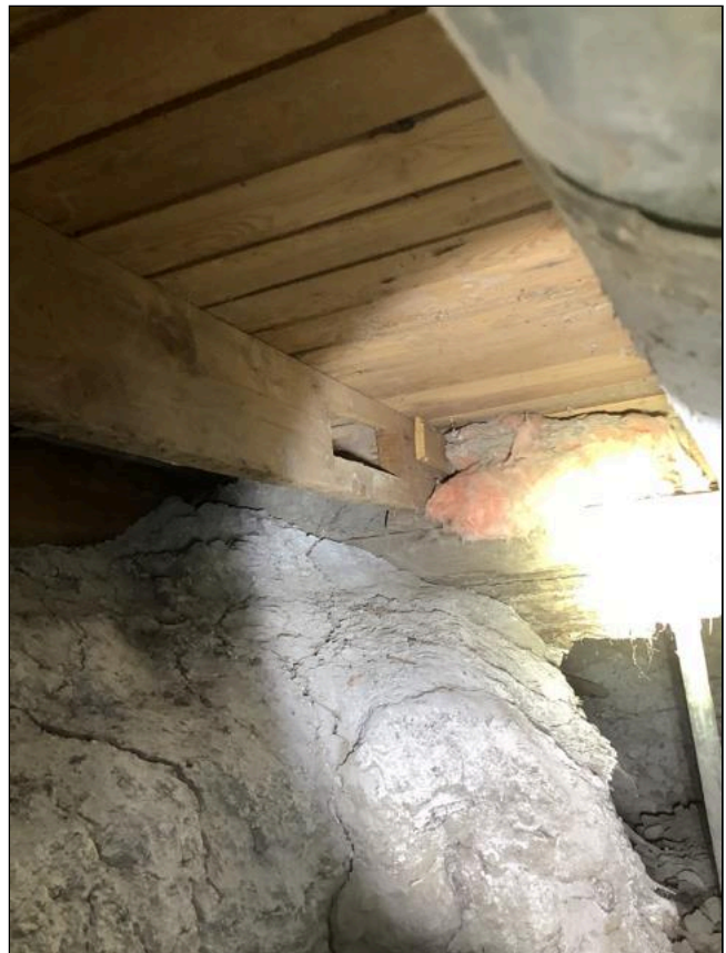
7.9 Item 6(Picture) Joists and Beams - notched out and split
