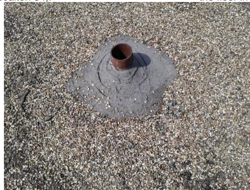
Non-asbestos black mastic (sample S0029) at a pipe penetration on the Roof (location 133).
