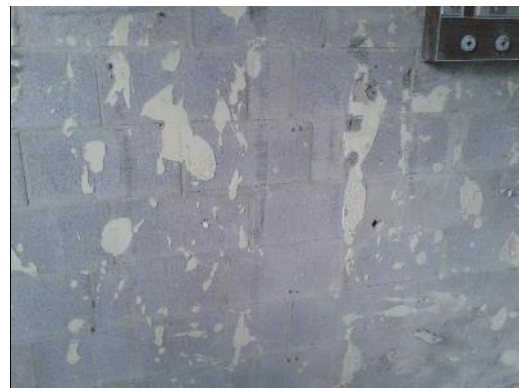
Asbestos-containing residual drywall joint compound pucks (sample S0018C) on the wall in Room 33 (location 60).
