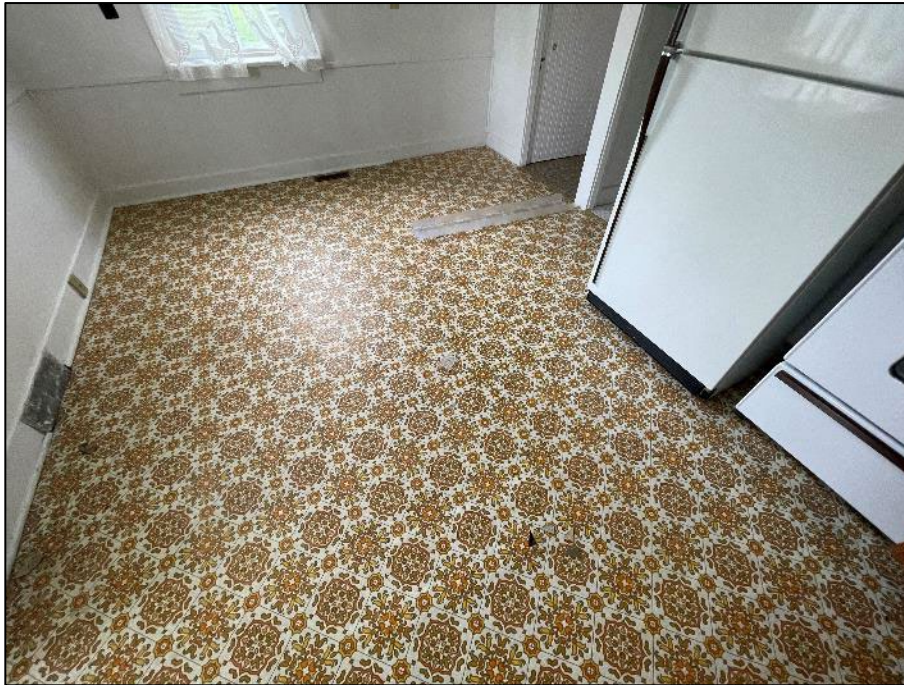
PHOTOGRAPH #5: Sheet Flooring (Brown) 3 Layers - Floor 1 Kitchen (20% Chrysotile)
