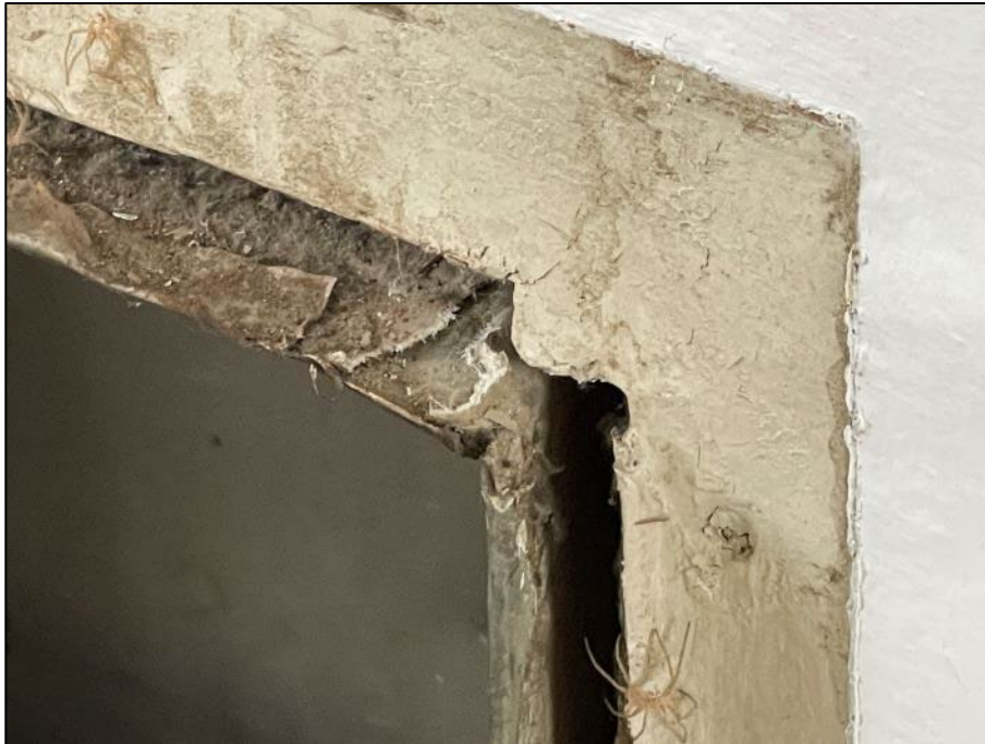
PHOTOGRAPH #11: Duct Wrap – Floor 1 Living Room (80% Chrysotile)
