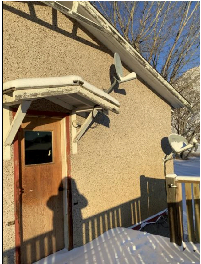
3.1 Item 2(Picture) Exterior - pebble dash may contain asbestos
