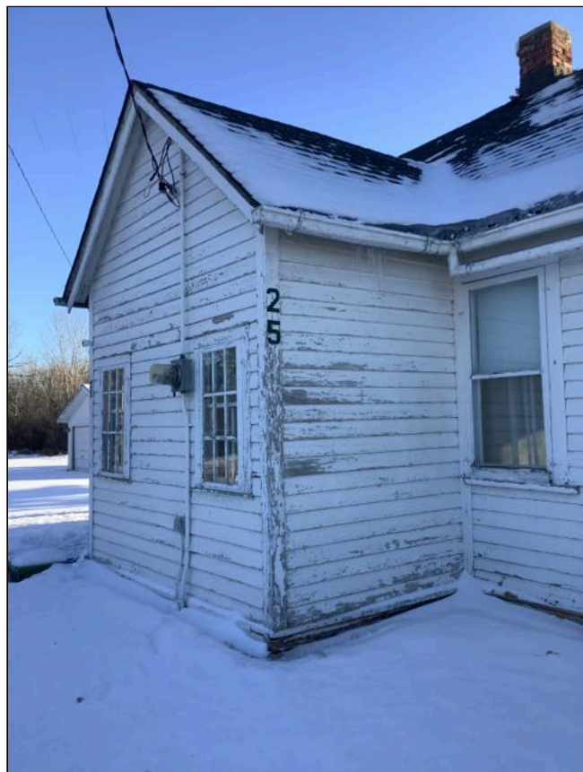
3.1 Item 7(Picture) Exterior - siding requires prep and paint
