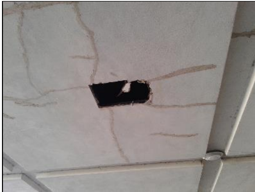
Non-asbestos plaster (sample S0004C) as a ceiling finish on the Exterior (location 1).
