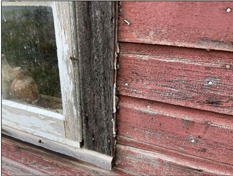
PHOTOGRAPH #23: Window Caulking - Large Shed Exterior (8% Chrysotile)
