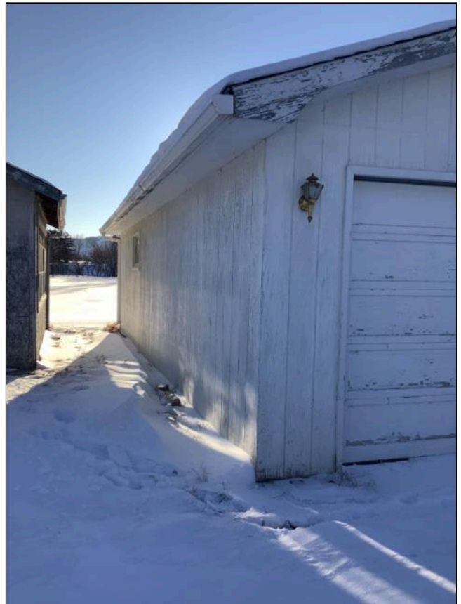
4.4 Item 4(Picture) Garage Exterior - siding requires prep and paint
