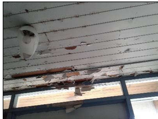
Lead-based white paint (sample L0009) on the wood ceiling in the Hallway (location 6).
