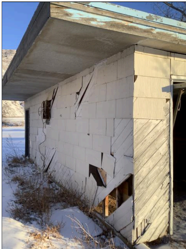
4.4 Item 2(Picture) Garage Exterior - damaged from flood, demo recommended
