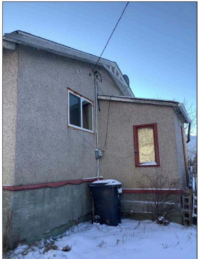
3.1 Item 4(Picture) Exterior - pebble dash may contain asbestos
