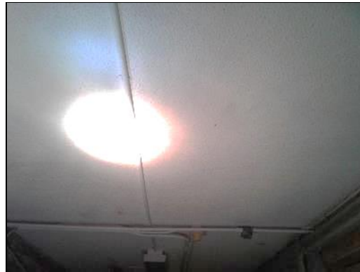
Asbestos-containing texture coat (sample S0017A) as a ceiling finish in the Hallway (location 43).
