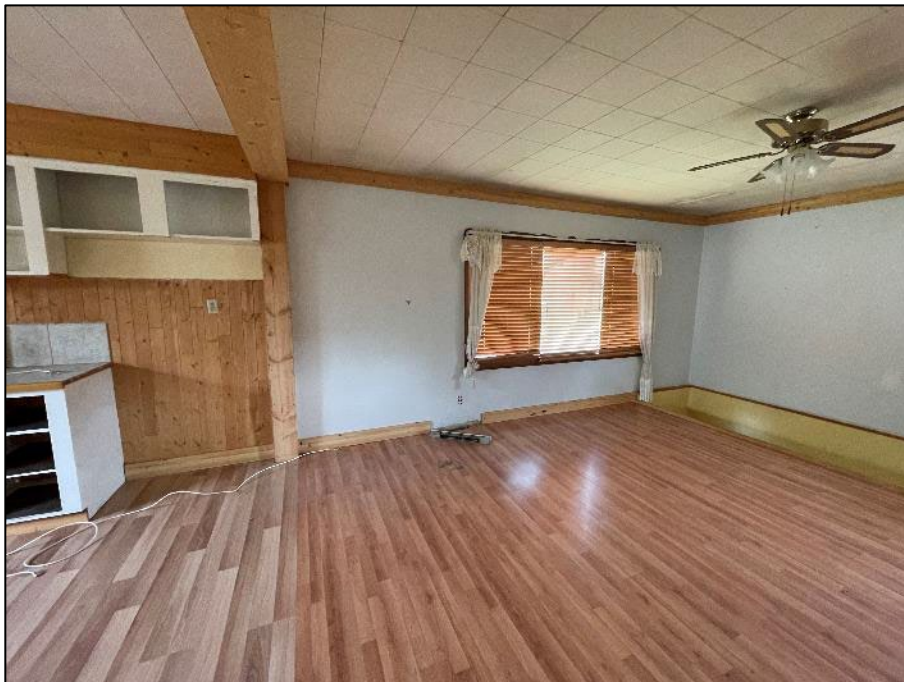
PHOTOGRAPH #2: Drywall Joint Compound - Level 1 Dining Area Exterior (2% Chrysotile)
