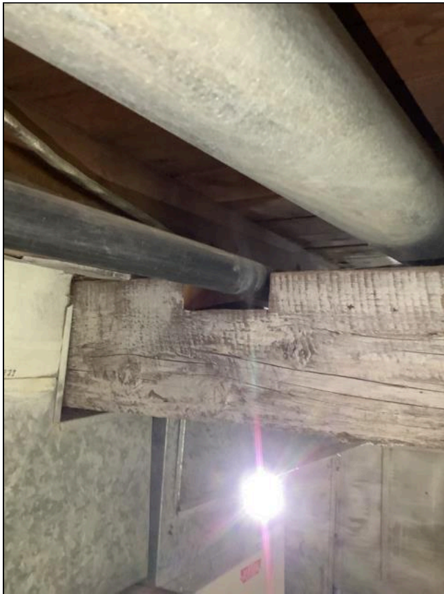
7.9 Item 3(Picture) Joists and Beams - notched out and split
