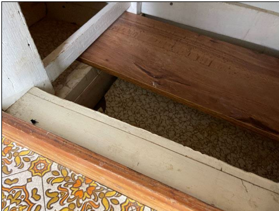
PHOTOGRAPH #6: Flooring (Beige/White) – Floor 1 Under Cabinets (25% Chrysotile)
