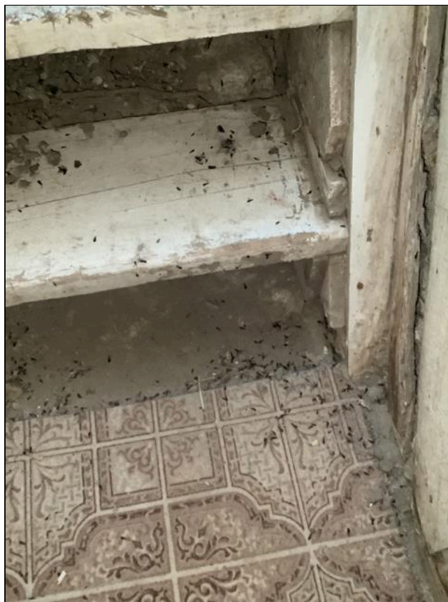
7.3 Item 1(Picture) Basement - signs of rodent droppings
