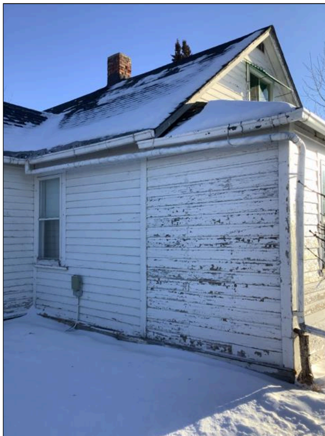
3.1 Item 6(Picture) Exterior - siding requires prep and paint
