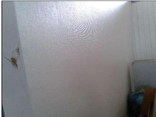
Lead-based white paint on drywall wall (sample L0006) in the Daycare (location 2).
