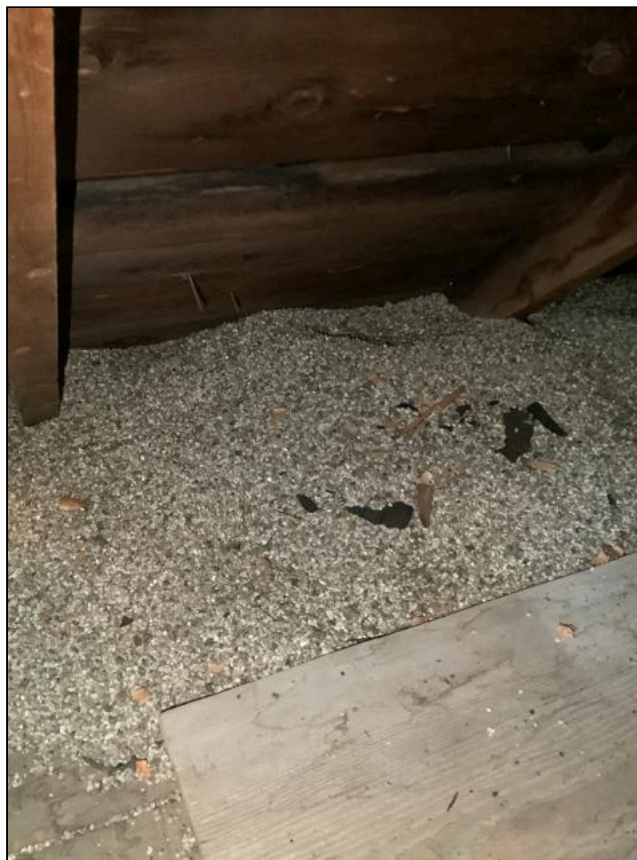
2.4 Item 1(Picture) Attic Insulation - vermiculite
