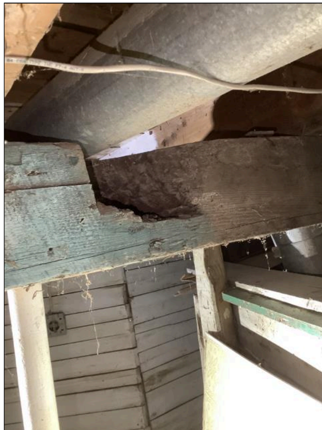
7.9 Item 2(Picture) Joists and Beams - notched out and split
