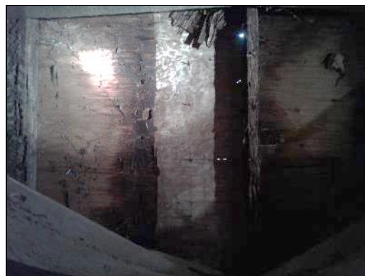
Mould growth on the wood wall in the Telephone Room (location 44).
