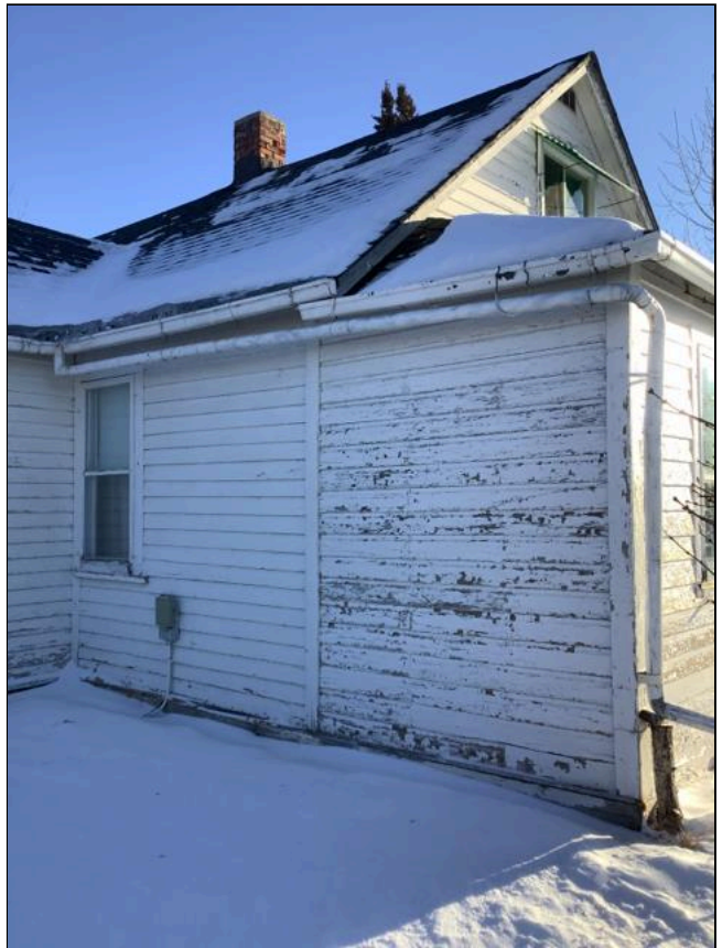
3.1 Item 6(Picture) Exterior - siding requires prep and paint
