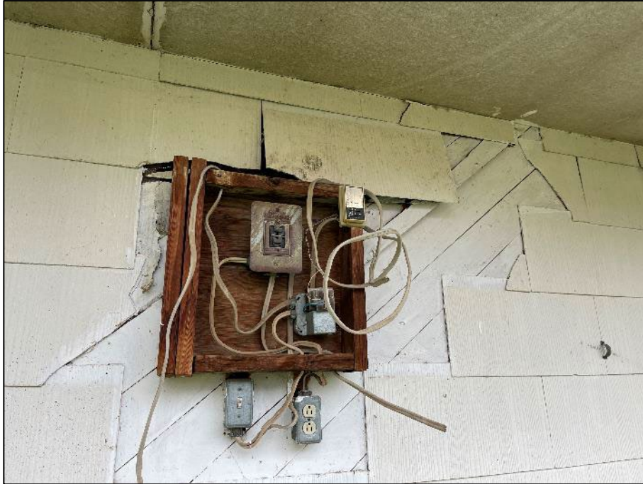
PHOTOGRAPH #35: Thermostat (Mercury)
