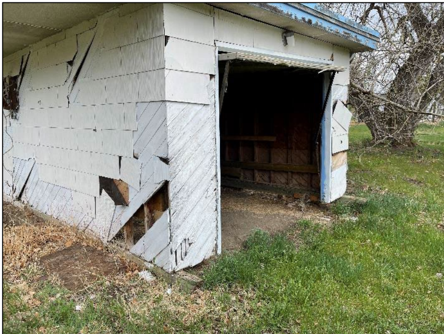
PHOTOGRAPH #30: Paint- Small White Shed (Lead Based)
