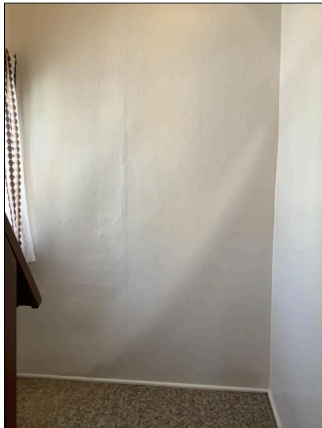
5.1 Item 7(Picture) Interior Walls - plaster wrinkling and cracked, may contain asbestos
