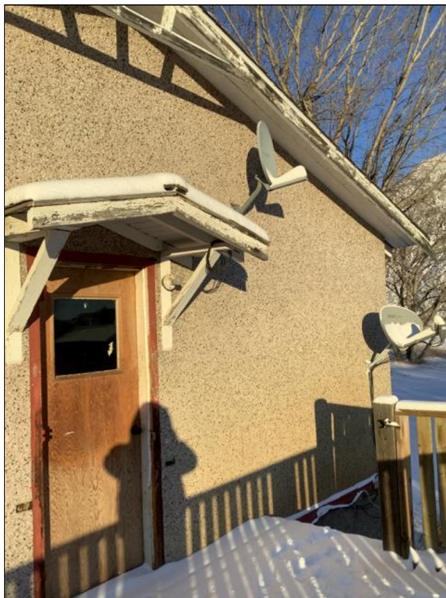
3.1 Item 2(Picture) Exterior - pebble dash may contain asbestos
