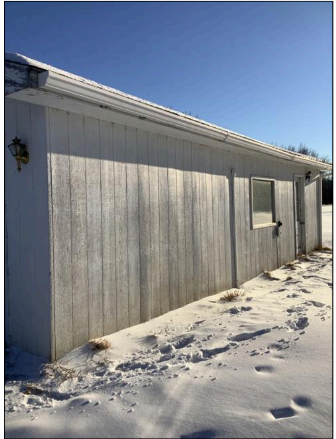
4.4 Item 2(Picture) Garage Exterior - siding requires prep and paint
