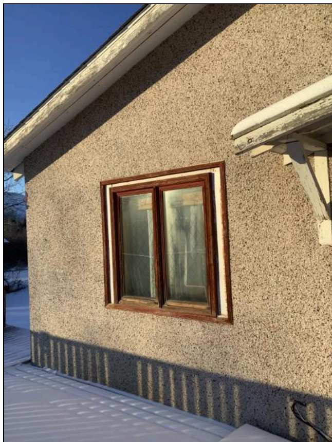
3.1 Item 1(Picture) Exterior - pebble dash may contain asbestos
