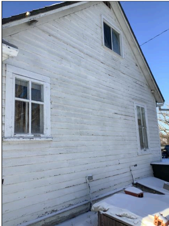
3.1 Item 1(Picture) Exterior - siding requires prep and paint
