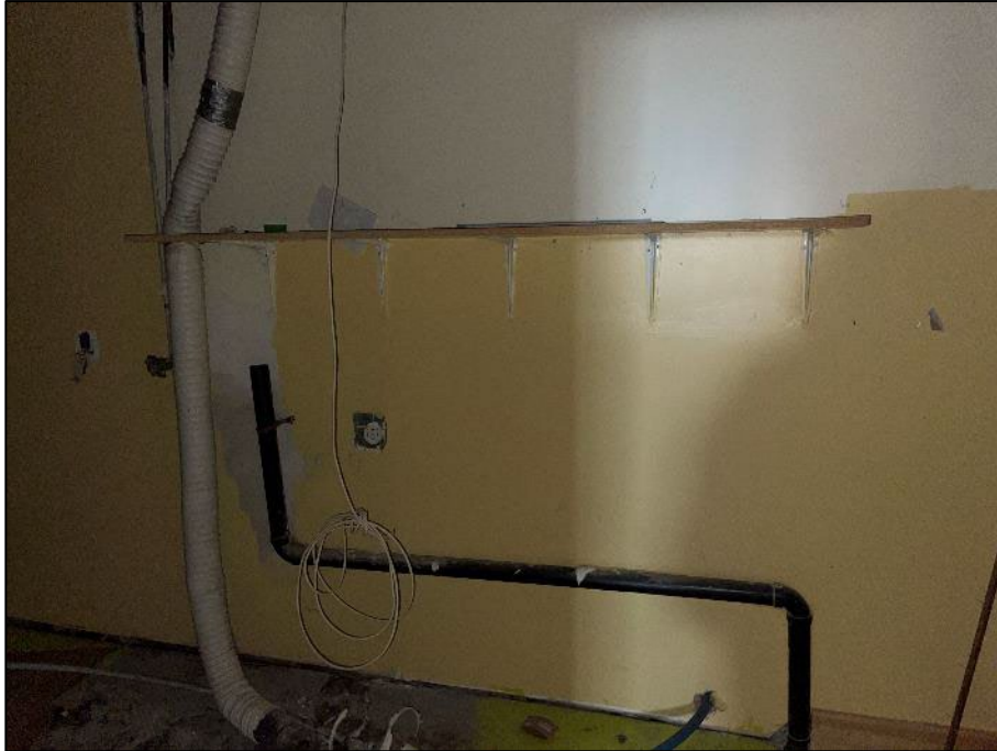
PHOTOGRAPH #5: Drywall Joint Compound - Basement Furnace Room Exterior (Assume Positive)
