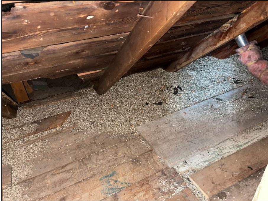
PHOTOGRAPH #21: Vermiculite in the Attic Space (<1% Actinolite)
