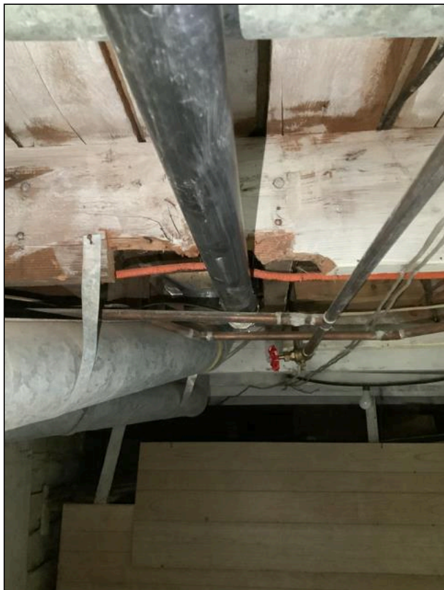
7.9 Item 1(Picture) Joists and Beams - notched out and split
