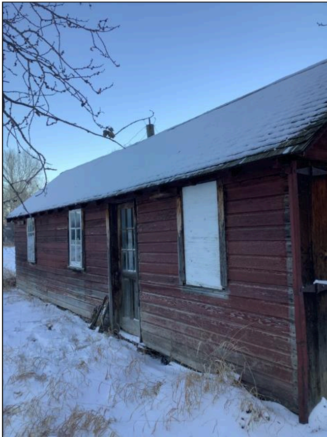
3.1 Item 13(Picture) Outbuilding - aged, structure demo recommended
