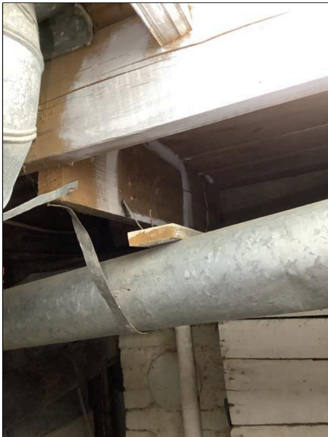
7.9 Item 5(Picture) Joists and Beams - notched out and split
