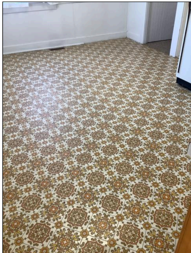
5.2 Item 3(Picture) Floor - heaved
