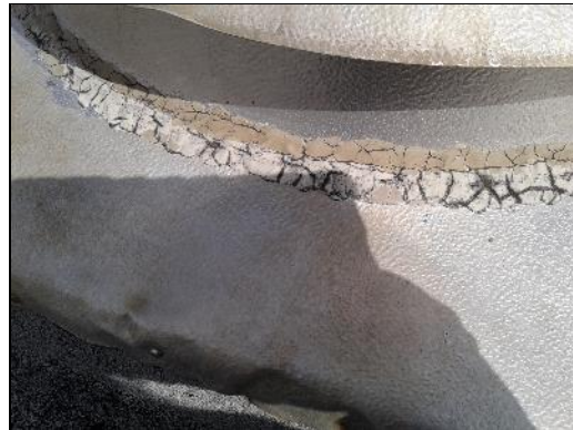
Non-asbestos white and black caulking (sample S0031) on piping on the Roof (location 133).
