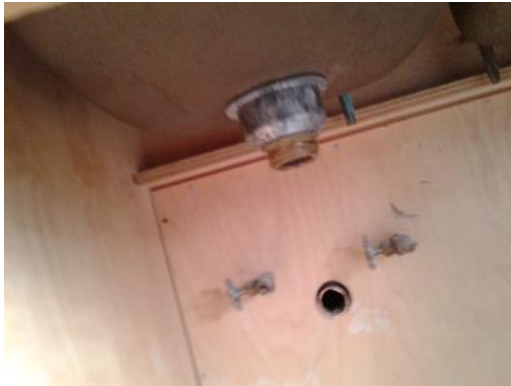
Asbestos-containing mastic below the sink (sample S0025) in the Nureses Room (location 84).
