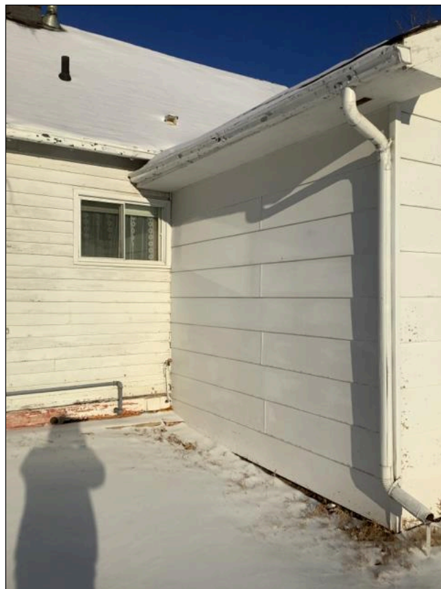
3.1 Item 4(Picture) Exterior - siding requires prep and paint
