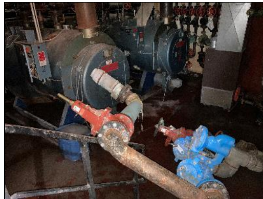
General view of mechanical equipment.
