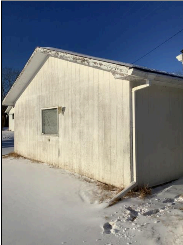
4.4 Item 1(Picture) Garage Exterior - siding requires prep and paint
