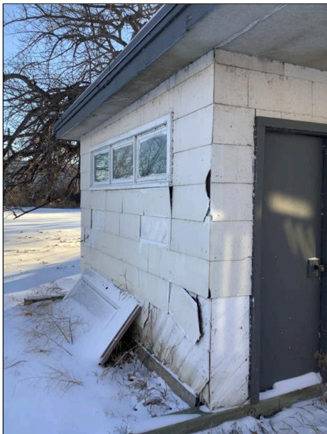
4.4 Item 3(Picture) Garage Exterior - damaged from flood, demo recommended
