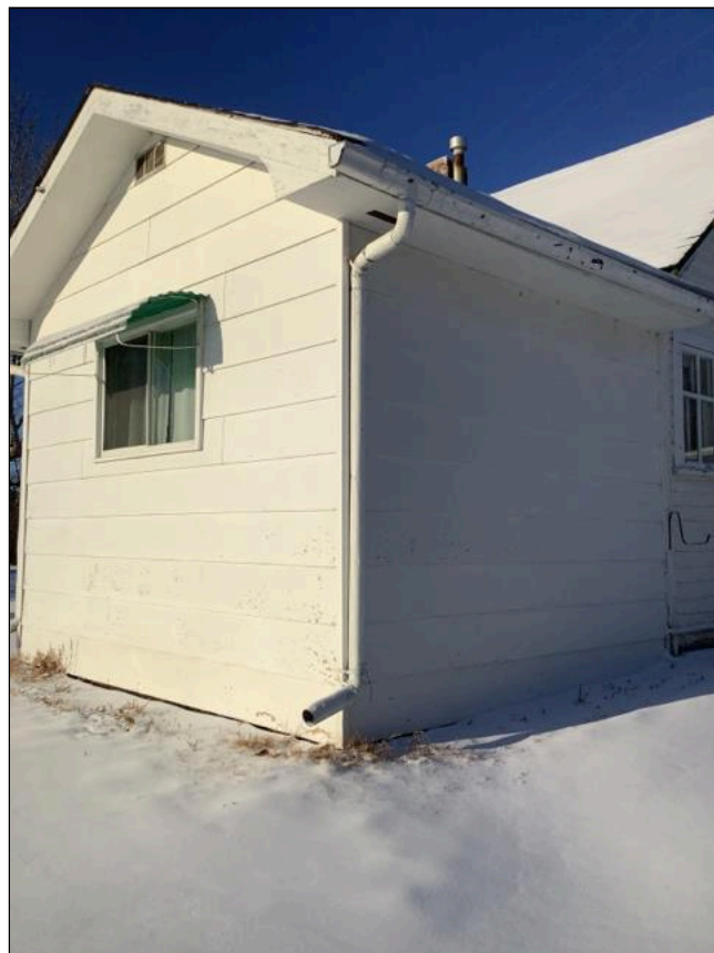
3.1 Item 2(Picture) Exterior - siding requires prep and paint
