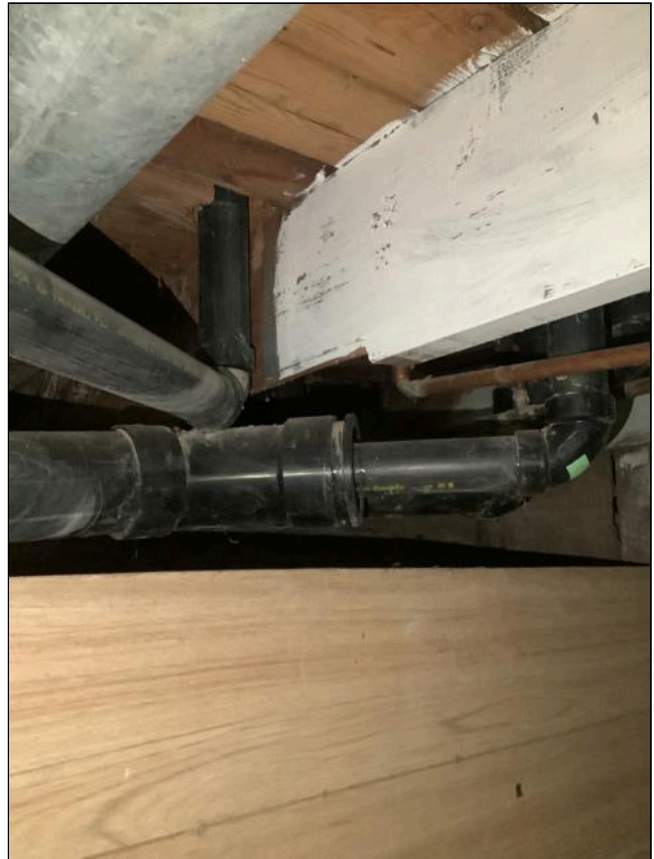
7.9 Item 4(Picture) Joists and Beams - notched out and split
