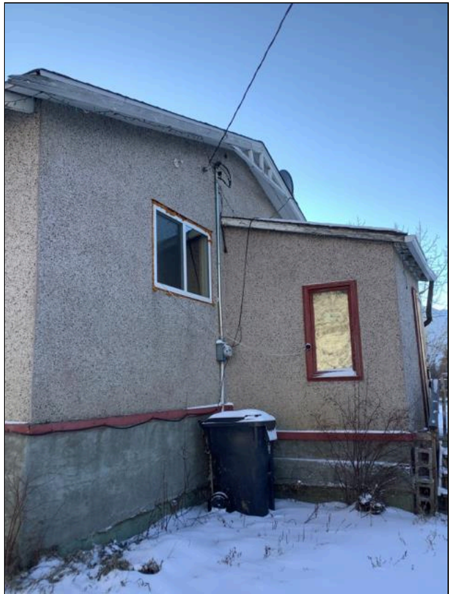
3.1 Item 4(Picture) Exterior - pebble dash may contain asbestos
