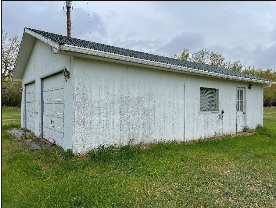
PHOTOGRAPH #17: Paint- White Exterior of Large Garage (Lead Based)
