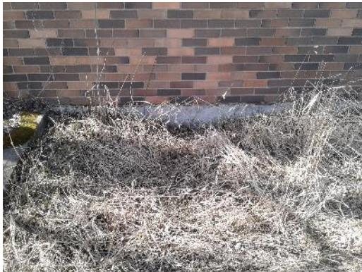
Non-asbestos brick mortar (sample S0001G) and non-asbestos paring cement over foundation (sample S0002G) on the Exterior (location 1).
