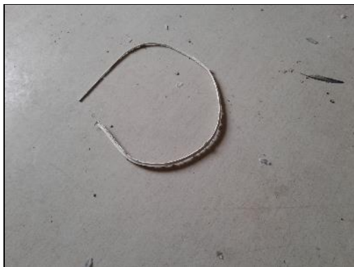
Non-asbestos white caulking debris (sample S0023) in Room 24 (location 79).
