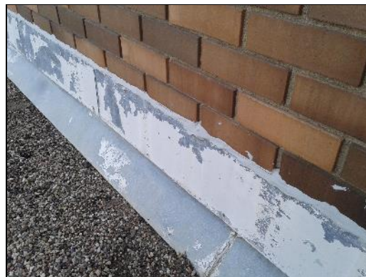
Lead-based white paint (sample L0010) on the metal trim on the Roof (location 133).
