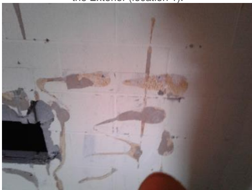
Non-asbestos adhesive (sample S0008) on the concrete block wall in the Administration Area (location 2).
