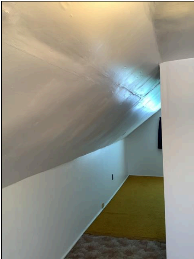
5.0 Item 3(Picture) Ceiling - plaster wrinkled and cracking, may contain asbestos
