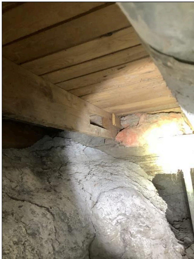
7.9 Item 6(Picture) Joists and Beams - notched out and split
