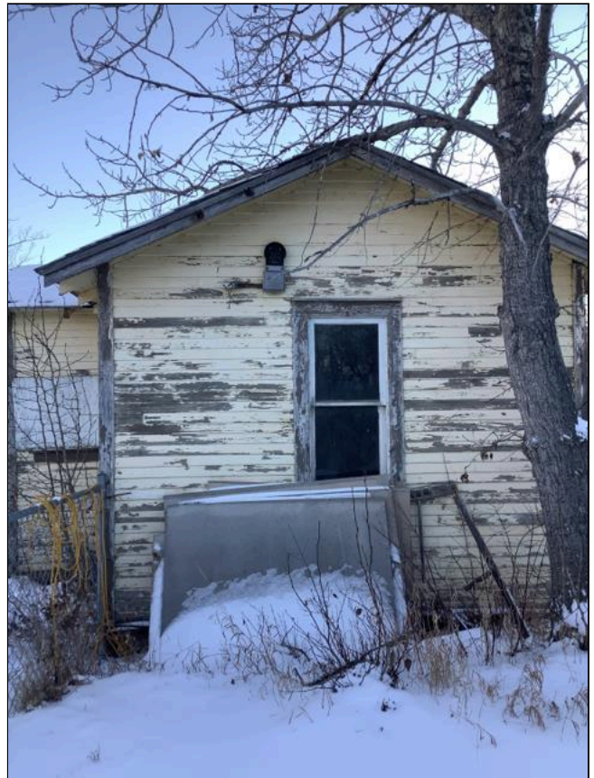
3.1 Item 8(Picture) Outbuilding - aged, structure demo recommended
