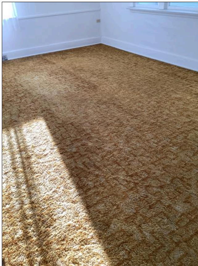
5.2 Item 2(Picture) Floor - heaved
