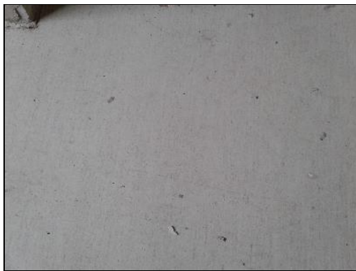
Non-asbestos grey streaks patterned vinyl sheet flooring (sample S0022) in Room 24 (location 79).
