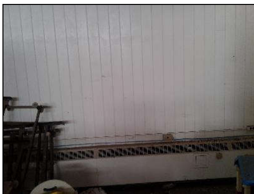
Lead-based white paint on the wood wall (sample L0004) in the Daycare (location 2).
