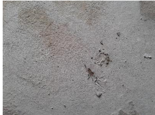
Non-asbestos unidentified cement product (sample S0026) on the floor in the Office (location 106).
