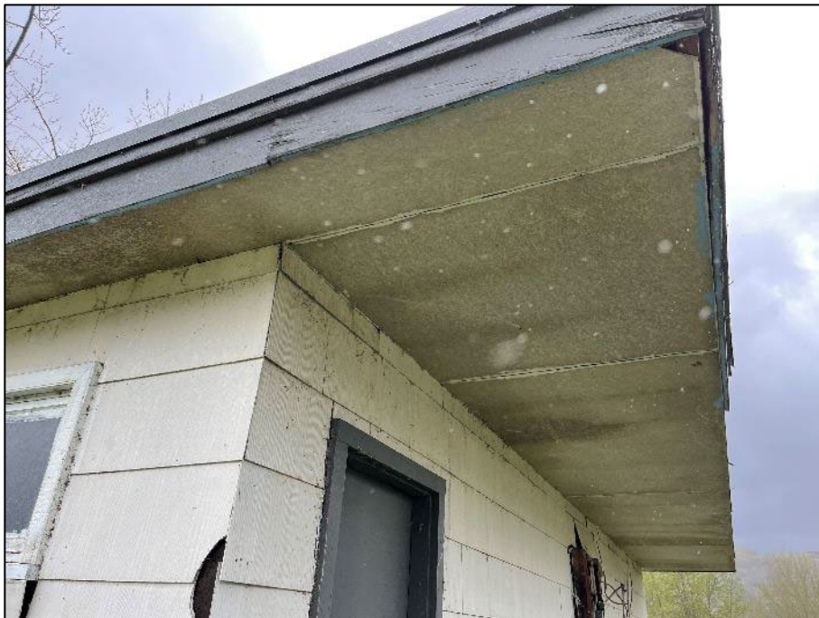
PHOTOGRAPH #20: Transite Soffit - Small Shed (15% Chrysotile)
