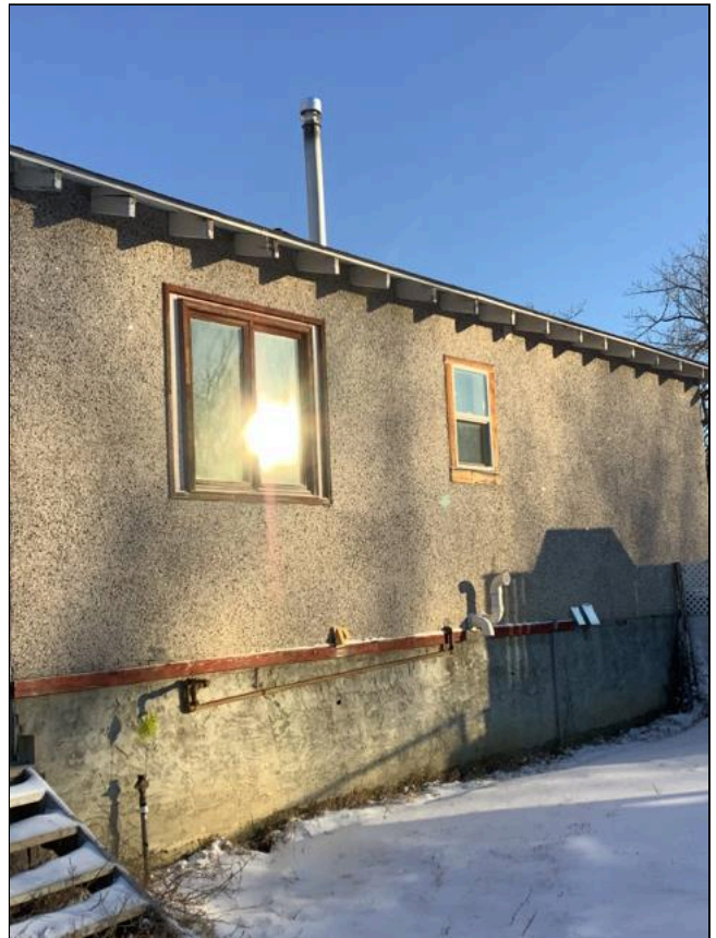
3.1 Item 6(Picture) Exterior - pebble dash may contain asbestos
