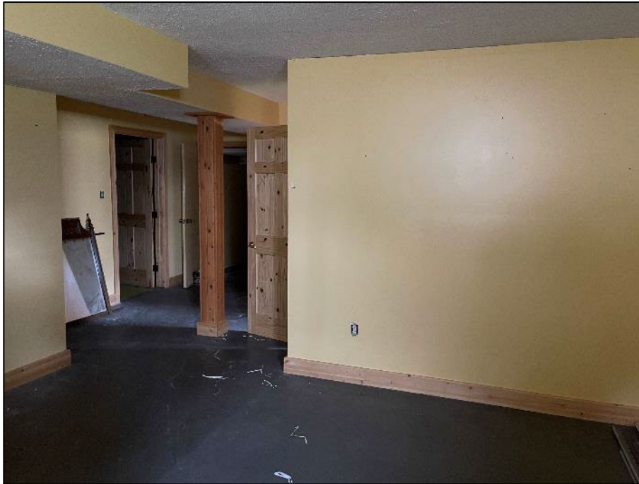
PHOTOGRAPH #7: Drywall Joint Compound - Basement Living Room Interior (Assume Positive)
