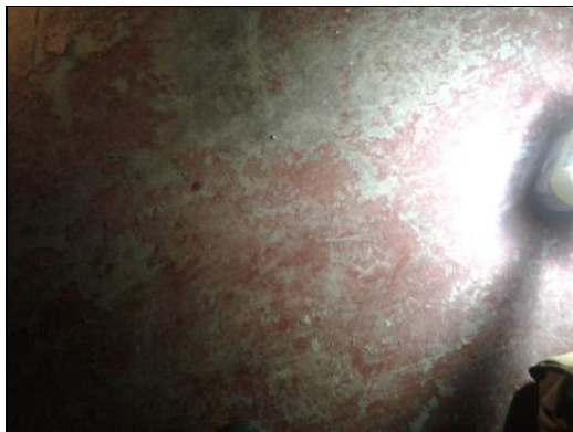
Lead-based red paint (sample L0007) on the concrete floor in the Mechanical Room (location 27).
