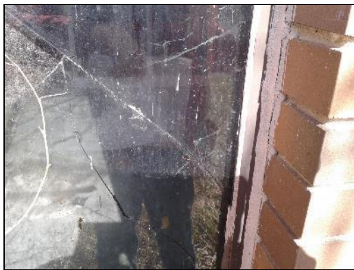
Non-asbestos grey caulking (sample S0003) on the window on the Exterior (location 1).
