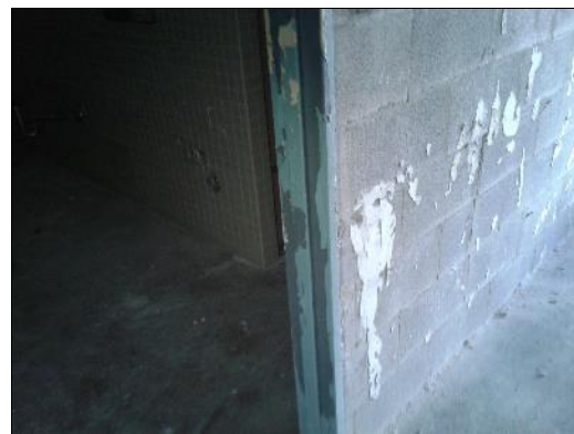
Lead-based blue paint (sample L0004) on the metal door frame in the Shower Room (location 16).
