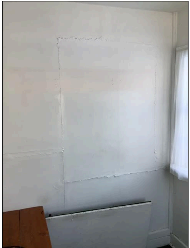
5.1 Item 6(Picture) Interior Walls - plaster wrinkling and cracked, may contain asbestos
