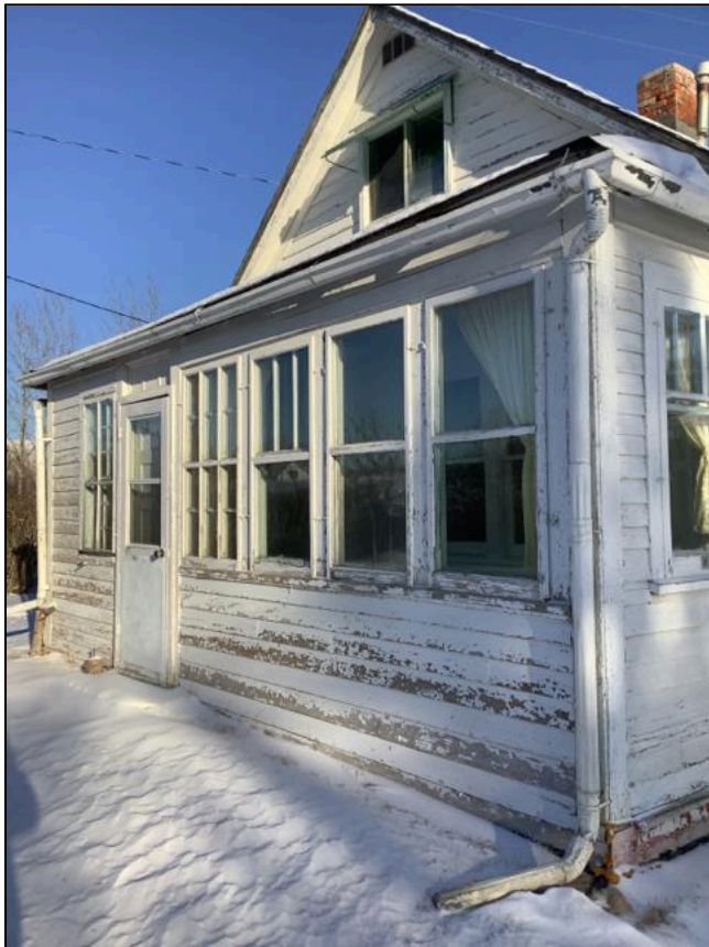
3.1 Item 5(Picture) Exterior - siding requires prep and paint
