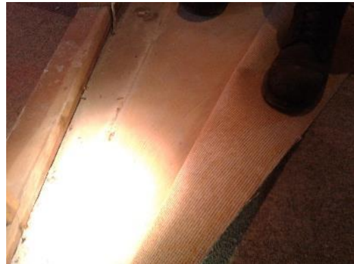
Asbestos-containing adhesive below carpet (sample S0007) in the Administration Area (location 2).
