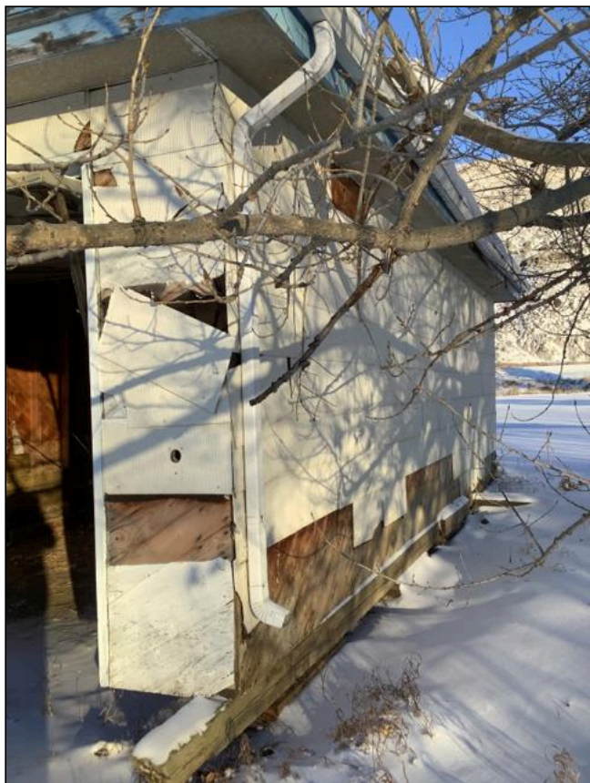
4.4 Item 1(Picture) Garage Exterior - damaged from flood, demo recommended
