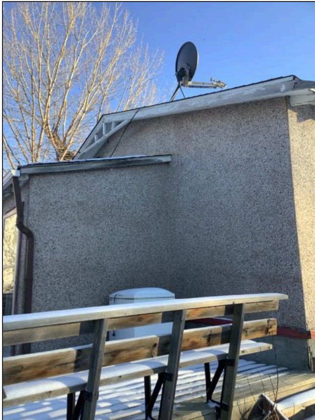
3.1 Item 5(Picture) Exterior - pebble dash may contain asbestos
