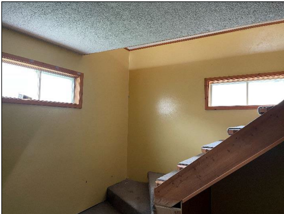
PHOTOGRAPH #6: Drywall Joint Compound - Basement Stairs Exterior (Assume Positive)
