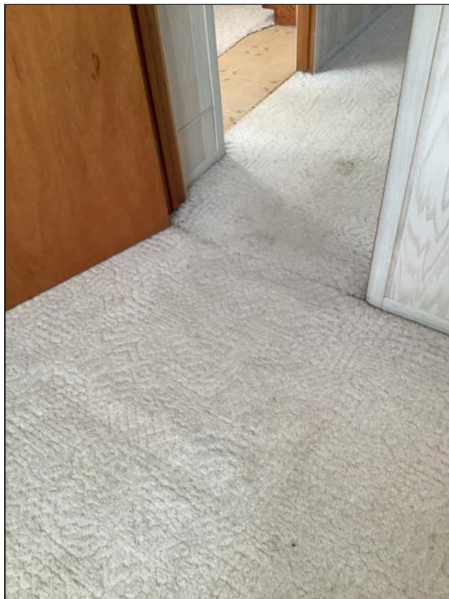
5.2 Item 1(Picture) Bedroom/Bathroom Floor - soft spot
