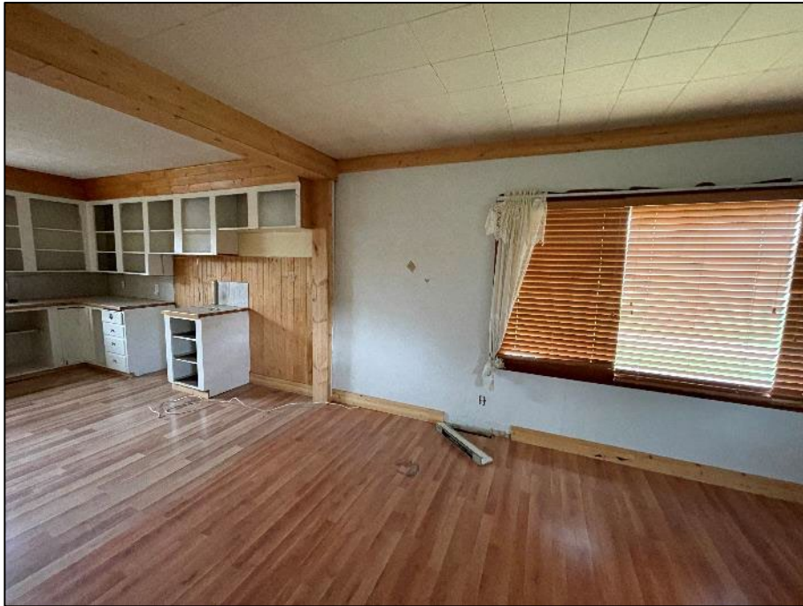
PHOTOGRAPH #27: Paint- White Interior Dining Room (Lead Based)
