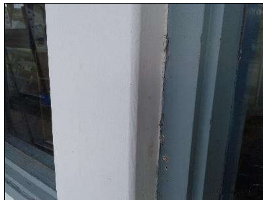
Non-asbestos grey caulking, covered in paint (sample S0001) on the window on the Exterior (location 1).
