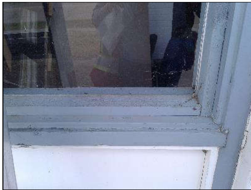
Lead-based white paint (sample L0001) on the wood wall and lead-based blue paint (sample L0002) on the wood window frame on the Exterior (location 1).
