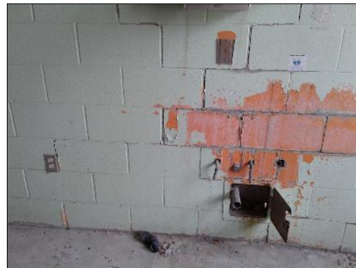
Lead-based green paint (sample L0008) and lead-based orange paint (sample L0009) on the masonry block wall in the Laundry Area (location 36).
