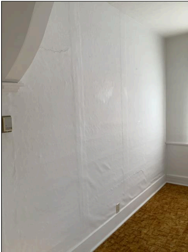
5.1 Item 3(Picture) Interior Walls - plaster wrinkling and cracked, may contain asbestos
