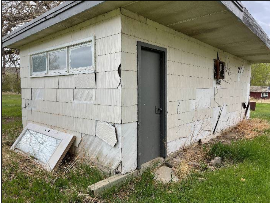
PHOTOGRAPH #21: Cement Shingle - Small Shed (10% Chrysotile)
