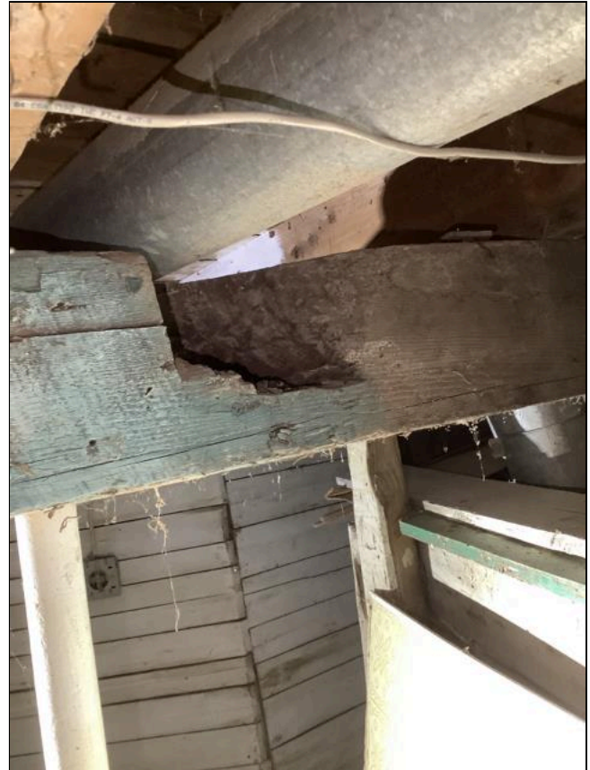
7.9 Item 2(Picture) Joists and Beams - notched out and split
