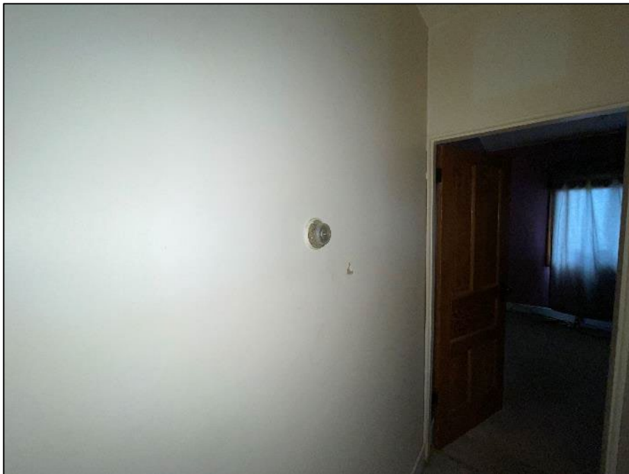
PHOTOGRAPH #36: Thermostat (Mercury)
