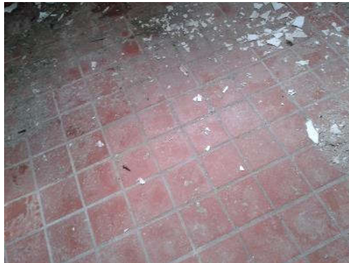
Ceramic tiles over non-asbestos thin set (sample S0006A) in the Men's Washroom (location 7).
