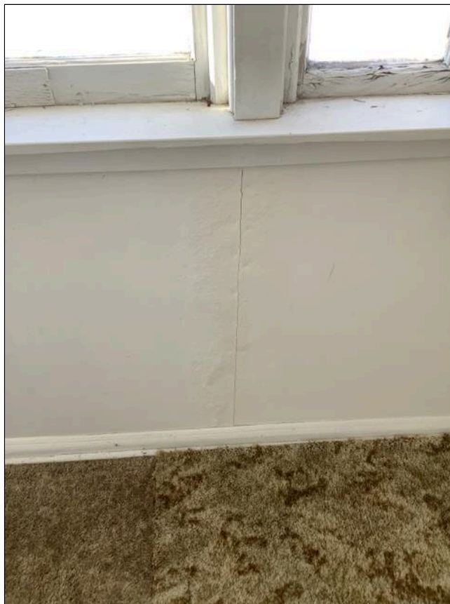
5.1 Item 2(Picture) Interior Walls - plaster wrinkling and cracked, may contain asbestos
