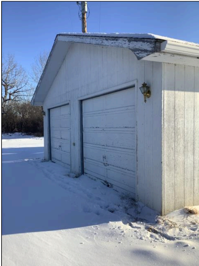
4.4 Item 3(Picture) Garage Exterior - siding requires prep and paint
