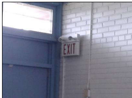
Lead-acid battery in the Daycare (location 2).
