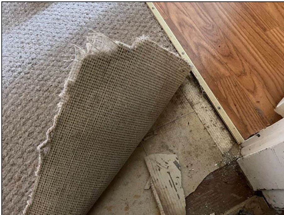
PHOTOGRAPH #14: Floor Tile - Level 1 Hallway (4% Chrysotile)
