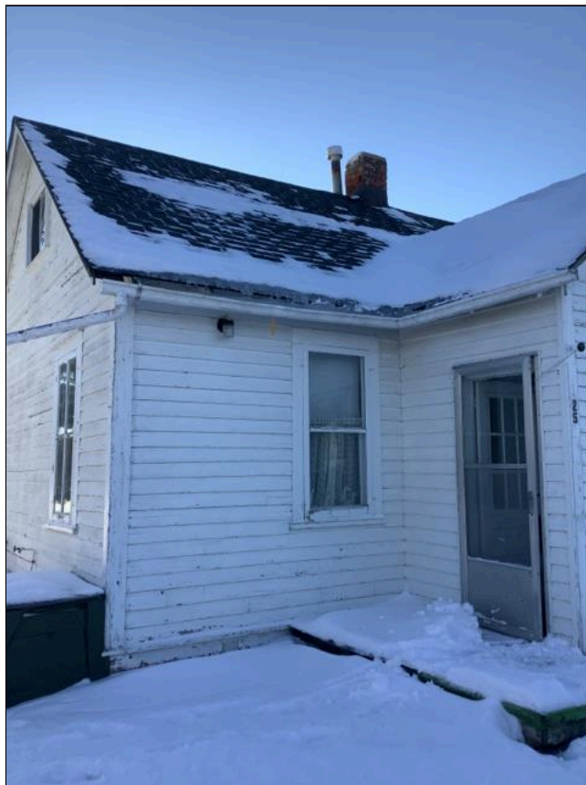
3.1 Item 8(Picture) Exterior - siding requires prep and paint
