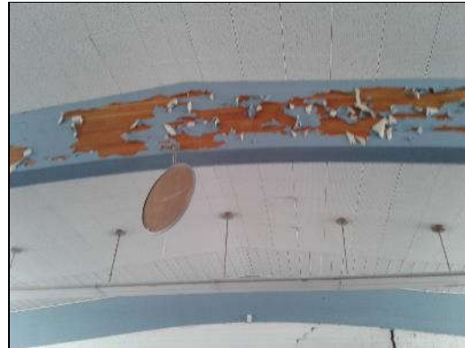
Lead-based blue paint (sample L0007) on wooden structural components in the Daycare (location 2).
