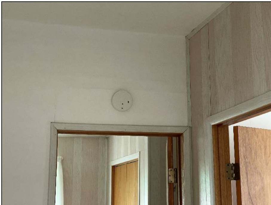
PHOTOGRAPH #18: Smoke Detector
