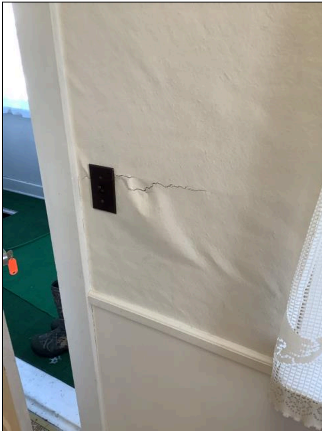
5.1 Item 5(Picture) Interior Walls - plaster wrinkling and cracked, may contain asbestos
