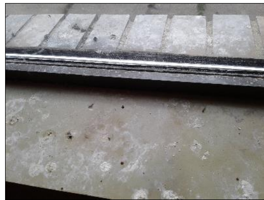
Asbestos-containing black caulking (sample S0021) on the window in Room 24 (location 47).
