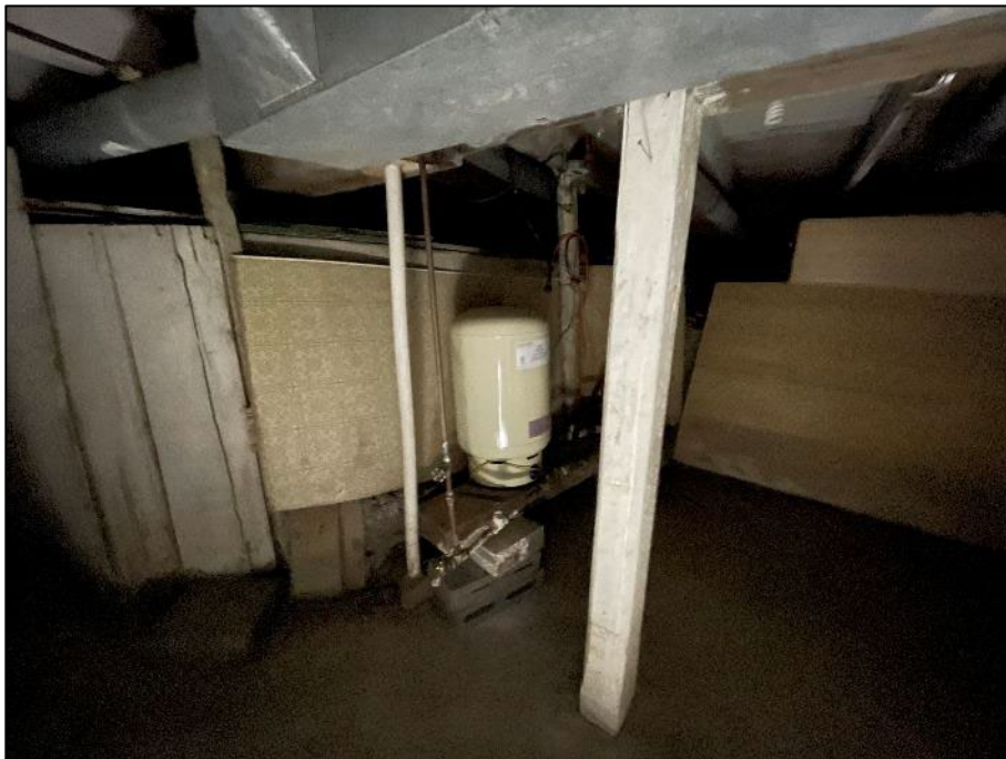
PHOTOGRAPH #22: Captive Air Tank in Basement
