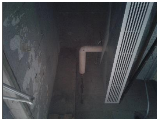
Asbestos-containing parging cement (sample S0012B) on pipe elbow in the Vestibule (location 17).
