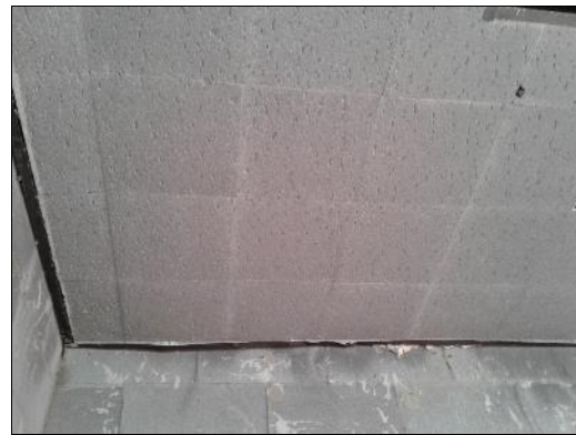
Non-asbestos 12"x12" fissures, mechanically fastened, acoustic ceiling tiles (sample S0028C) in the Conference Room (location 119).
