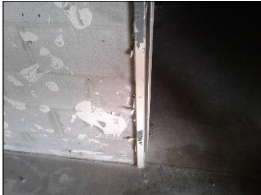
Lead-based white paint (sample L0005) on the metal door frame in the Vestibule (location 17).
