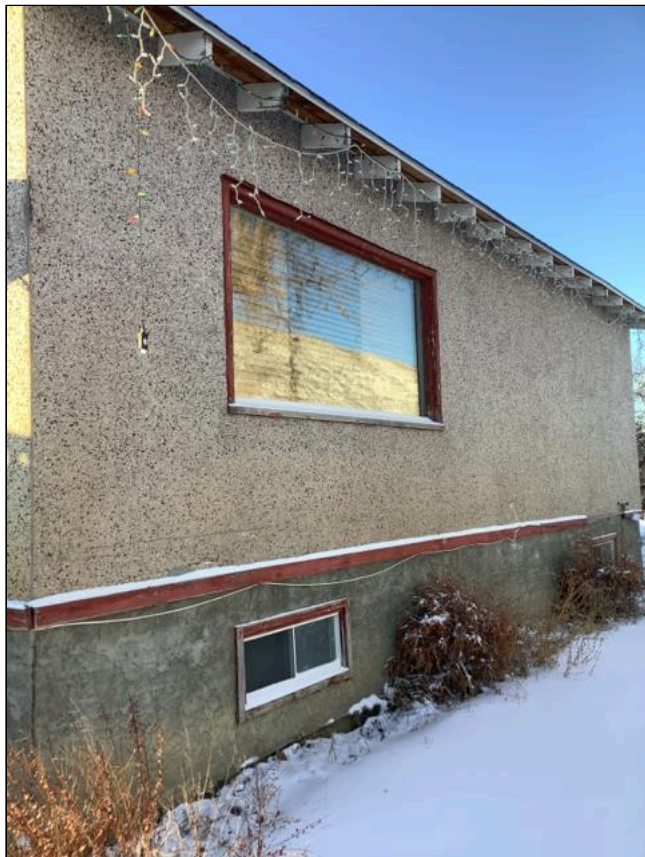
3.1 Item 3(Picture) Exterior - pebble dash may contain asbestos
