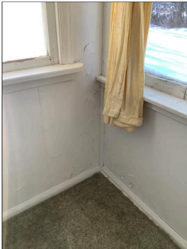
5.1 Item 1(Picture) Interior Walls - plaster wrinkling and cracked, may contain asbestos
