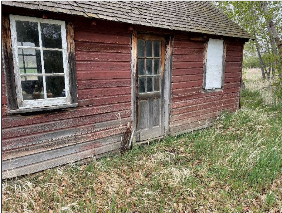
PHOTOGRAPH #31: Paint- Large Red Shed (Lead Based)
