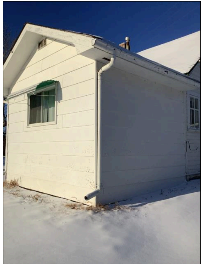
3.1 Item 2(Picture) Exterior - siding requires prep and paint
