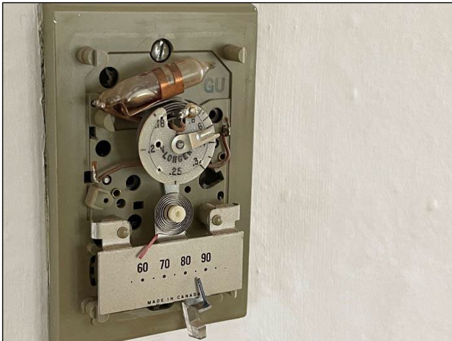
PHOTOGRAPH #20: Thermostat (Mercury)
