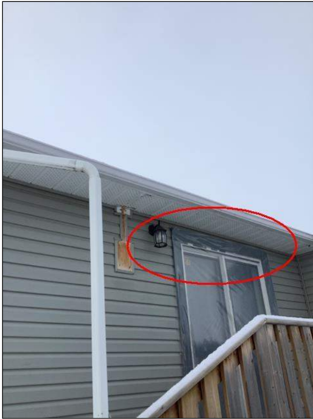
3.1 Item 9(Picture) Exterior Siding - bowed
