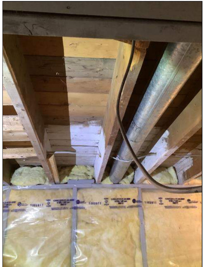
7.9 Item 10(Picture) Joists and Beams - slanted, crooked, notched out, bowed, split
