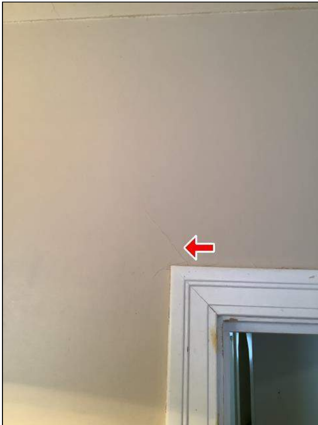
9.0 Item 3(Picture) Bathroom Wall - cracks from settling
