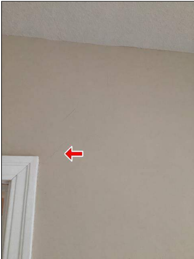
5.1 Item 5(Picture) Interior Walls - cracks from settling and shifting
