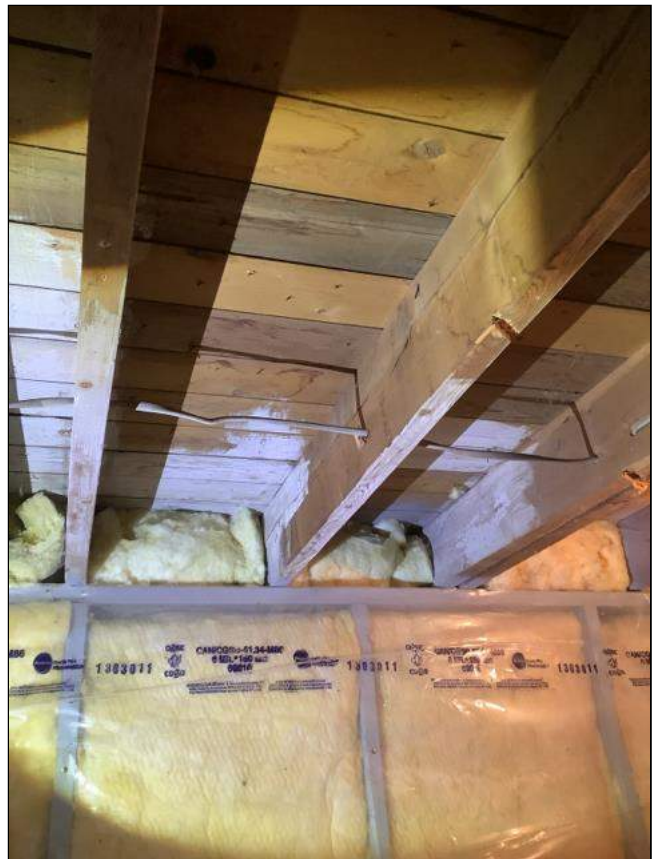
7.9 Item 8(Picture) Joists and Beams - slanted, crooked, notched out, bowed, split
