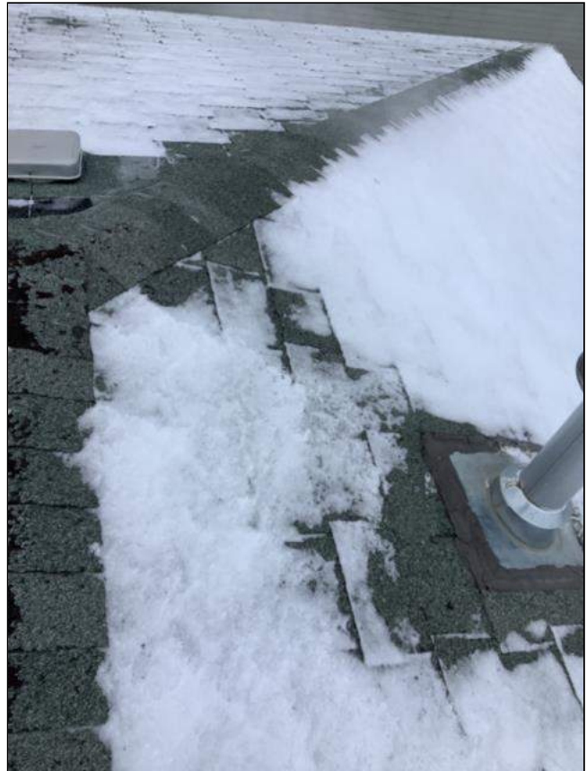
1.0 Item 2(Picture) Roof - shingles are aged and will require replacement
