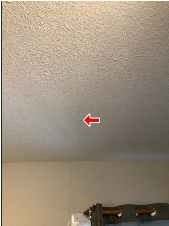
5.0 Item 3(Picture) Ceiling - common cracks from settling and shifting
