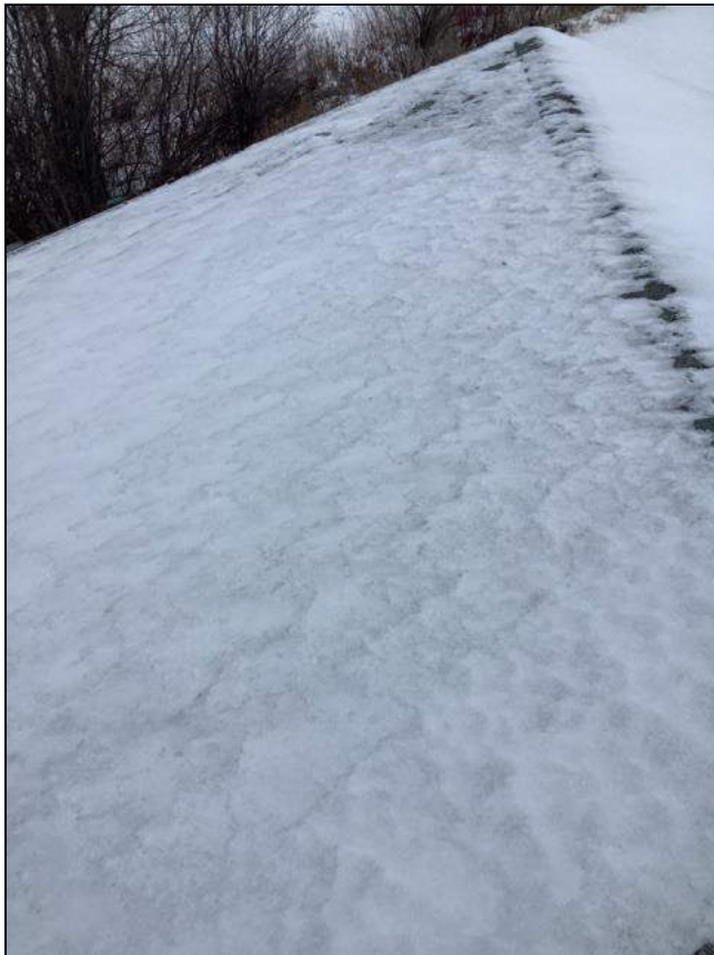
1.0 Item 5(Picture) Roof - shingles are aged and will require replacement
