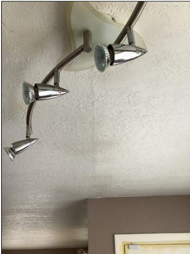
5.0 Item 5(Picture) Ceiling - signs of moisture damage, patching, stressed seams
