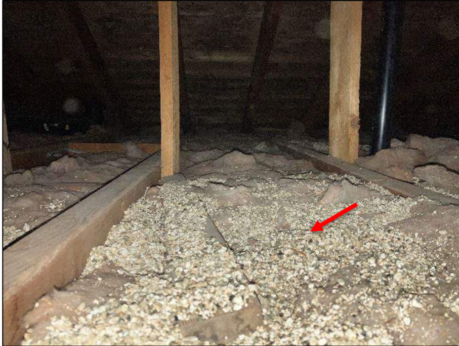
PHOTOGRAPH #21: Vermiculite in the Attic Space (<1% Tremolite)
