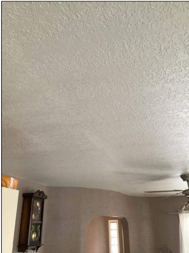
5.0 Item 7(Picture) Ceiling - signs of moisture damage, patching, stressed seams
