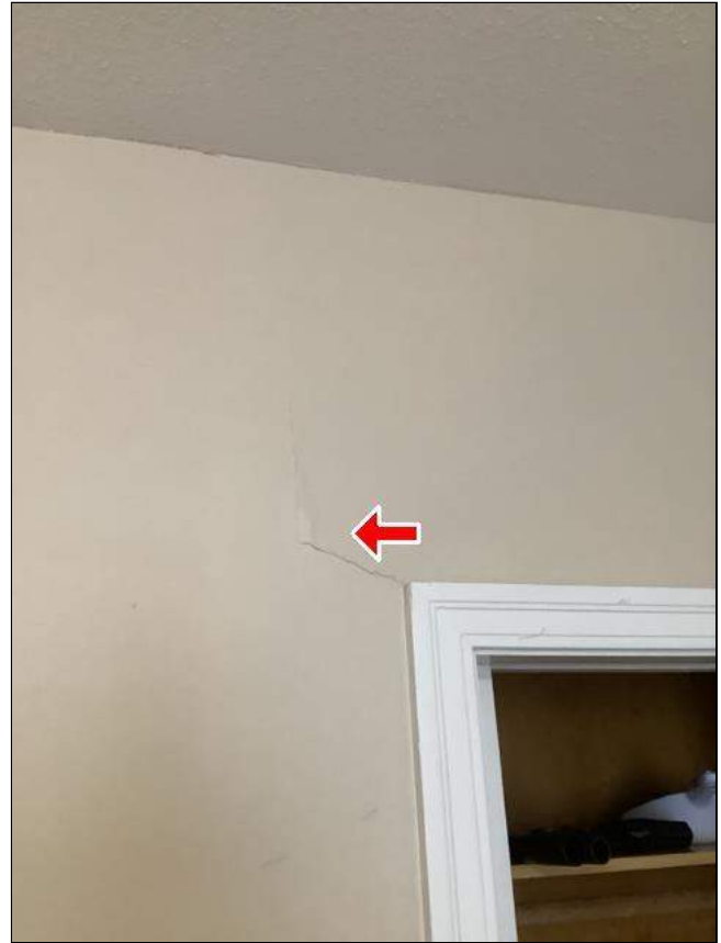
5.1 Item 2(Picture) Interior Walls - cracks from settling and shifting
