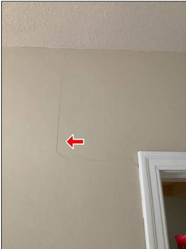
5.1 Item 3(Picture) Interior Walls - cracks from settling and shifting
