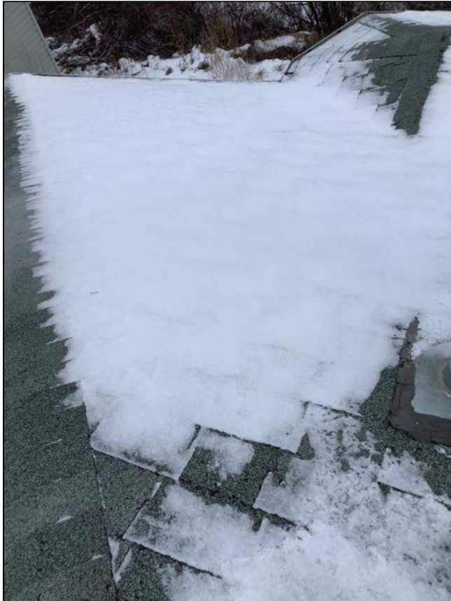
1.0 Item 3(Picture) Roof - shingles are aged and will require replacement
