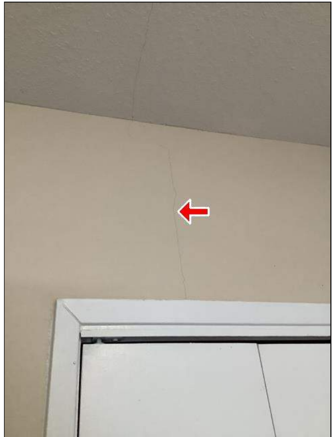
5.1 Item 6(Picture) Interior Walls - cracks from settling and shifting
