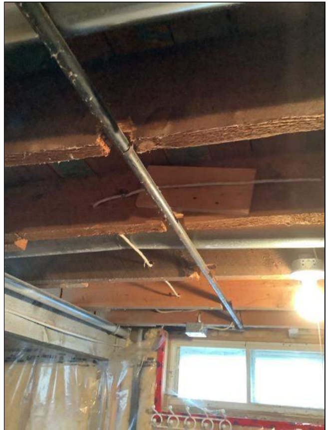
7.9 Item 22(Picture) Joists and Beams - slanted, crooked, notched out, bowed, split
