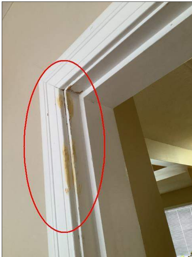
5.4 Item 2(Picture) Door - signs of rubbing
