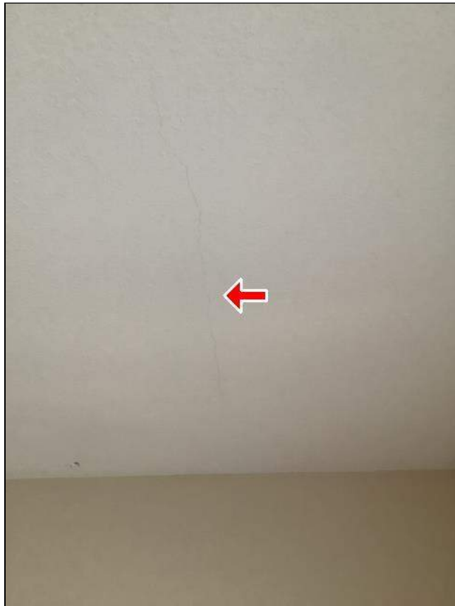
5.0 Item 1(Picture) Ceiling - common cracks from settling and shifting
