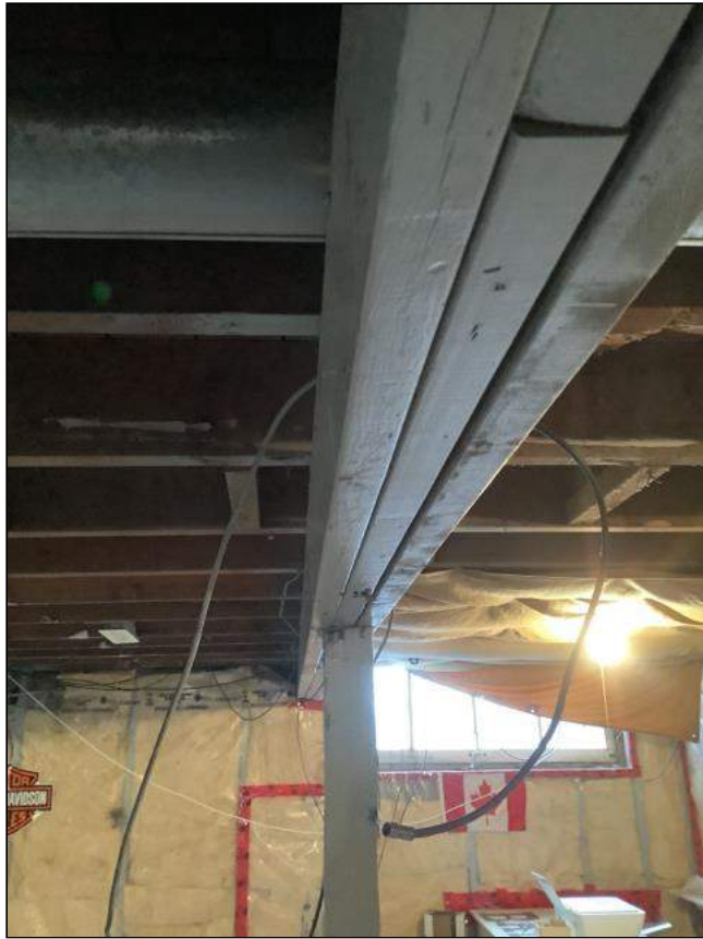
7.9 Item 1(Picture) Joists and Beams - slanted, crooked, notched out, bowed, split
