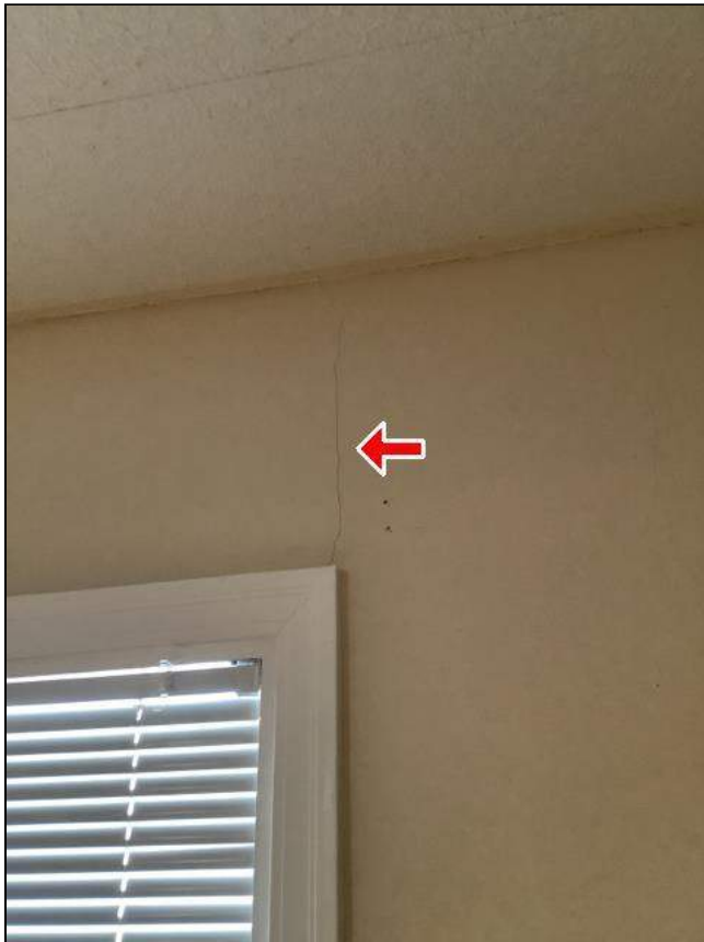
5.1 Item 7(Picture) Interior Walls - cracks from settling and shifting
