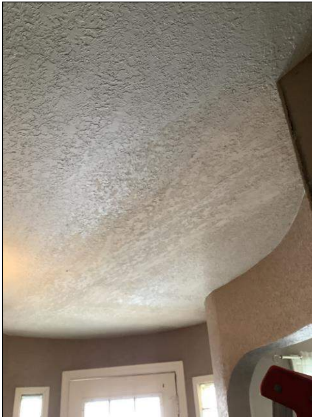
5.0 Item 3(Picture) Ceiling - signs of moisture damage, patching, stressed seams
