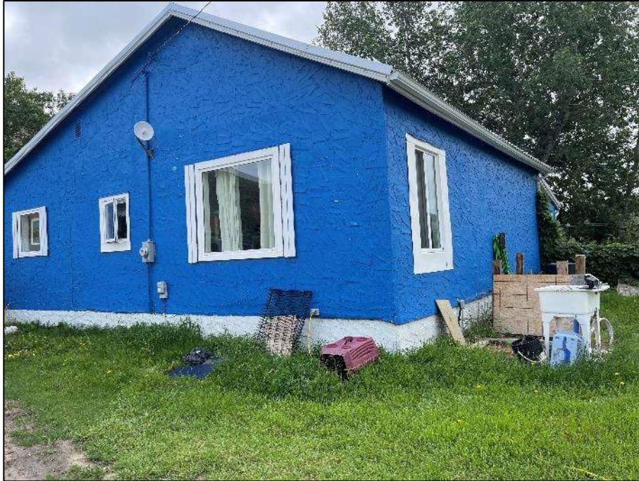
PHOTOGRAPH #15: Stucco - Exterior NW Corner (2% Chrysotile)
