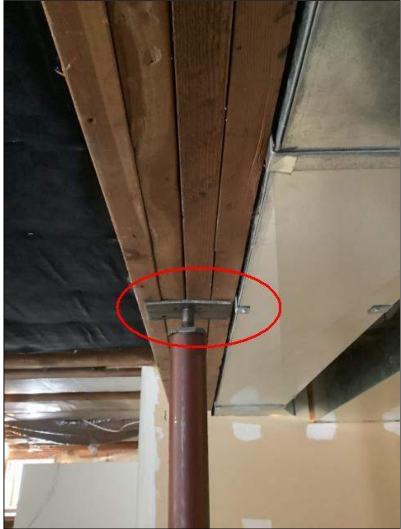
7.6 Item 1(Picture) Plate - bowed
