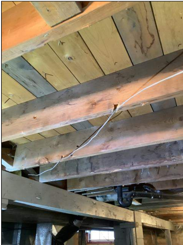
7.9 Item 17(Picture) Joists and Beams - slanted, crooked, notched out, bowed, split
