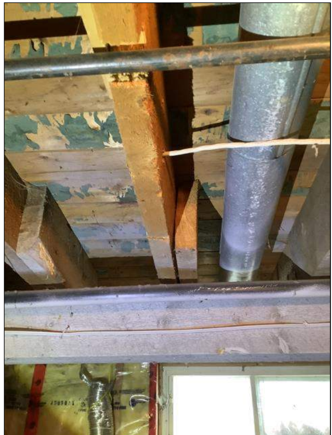
7.9 Item 28(Picture) Joists and Beams - slanted, crooked, notched out, bowed, split
