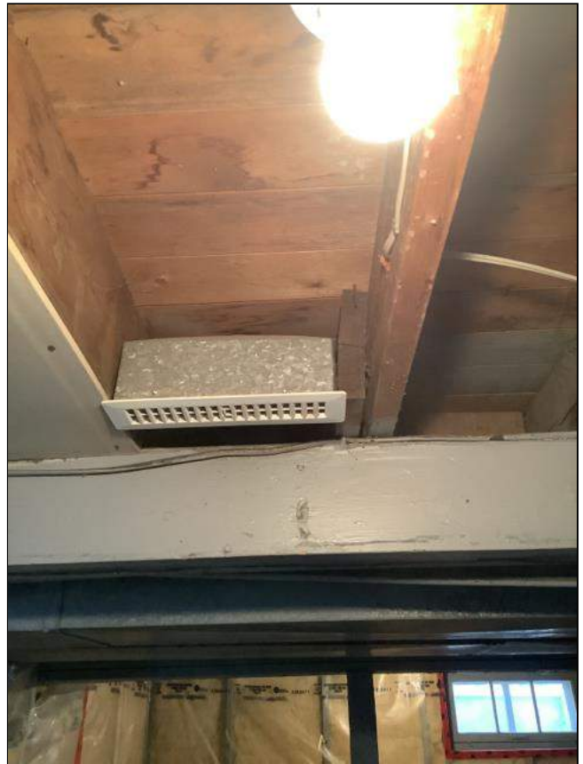
7.9 Item 6(Picture) Joists and Beams - slanted, crooked, notched out, bowed, split
