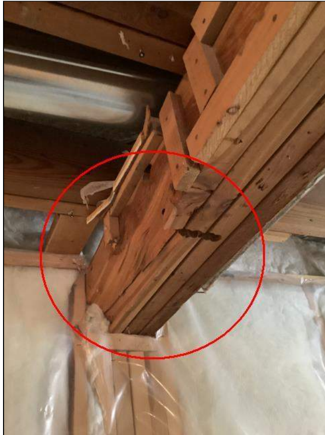
7.9 Item 1(Picture) Beam - end is broken
