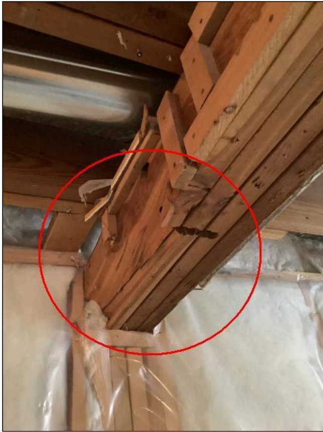
7.9 Item 1(Picture) Beam - end is broken
