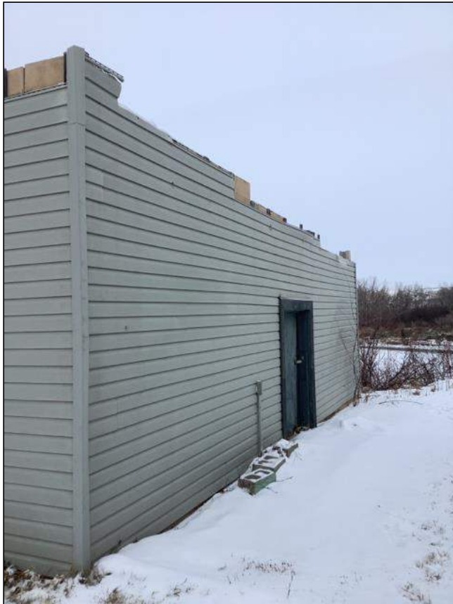
4.4 Item 1(Picture) Back of Garage - heavily bowed
