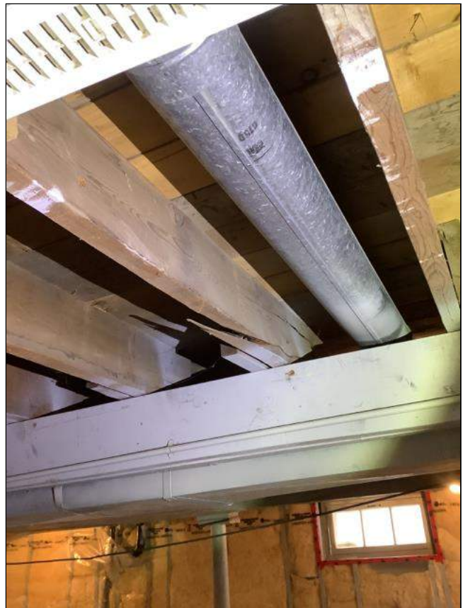
7.9 Item 12(Picture) Joists and Beams - slanted, crooked, notched out, bowed, split
