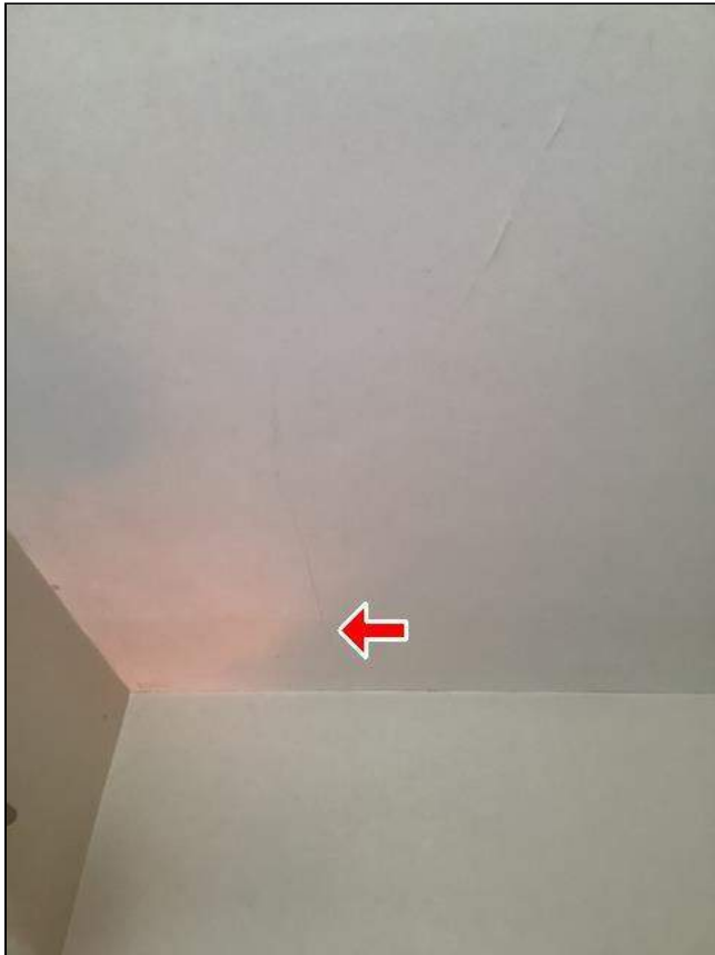
9.0 Item 1(Picture) Bathroom Ceiling - cracks from settling
