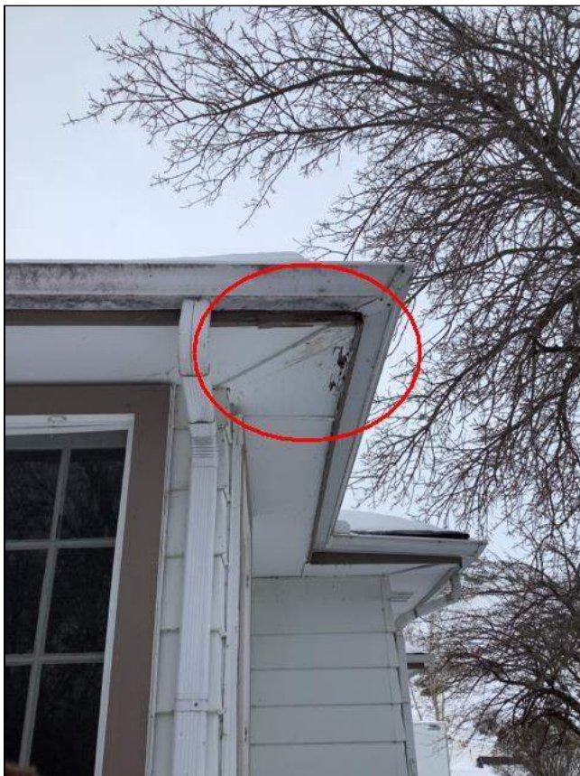
3.1 Item 1(Picture) Exterior - signs of moisture damage
