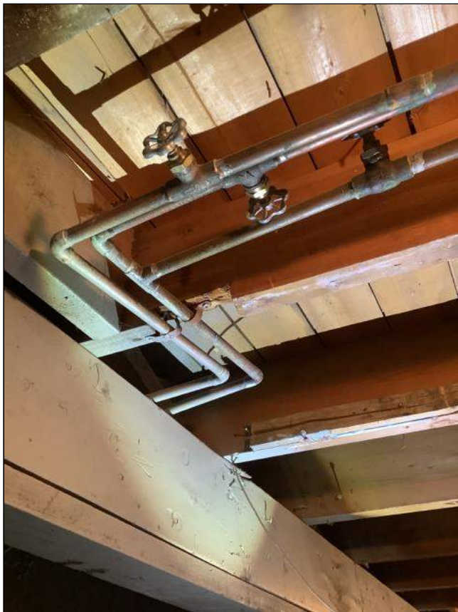
7.9 Item 19(Picture) Joists and Beams - slanted, crooked, notched out, bowed, split
