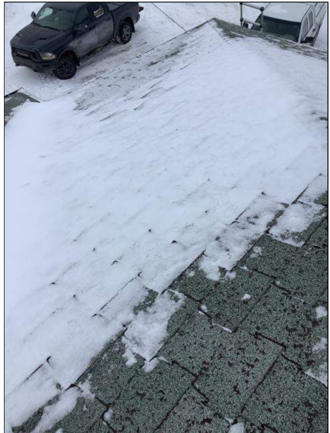
1.0 Item 10(Picture) Roof - shingles are aged and will require replacement
