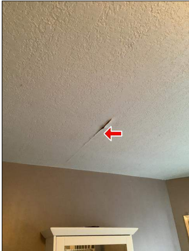
9.0 Item 1(Picture) Bathroom Ceiling - seam splitting
