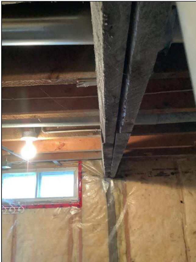
7.9 Item 21(Picture) Joists and Beams - slanted, crooked, notched out, bowed, split
