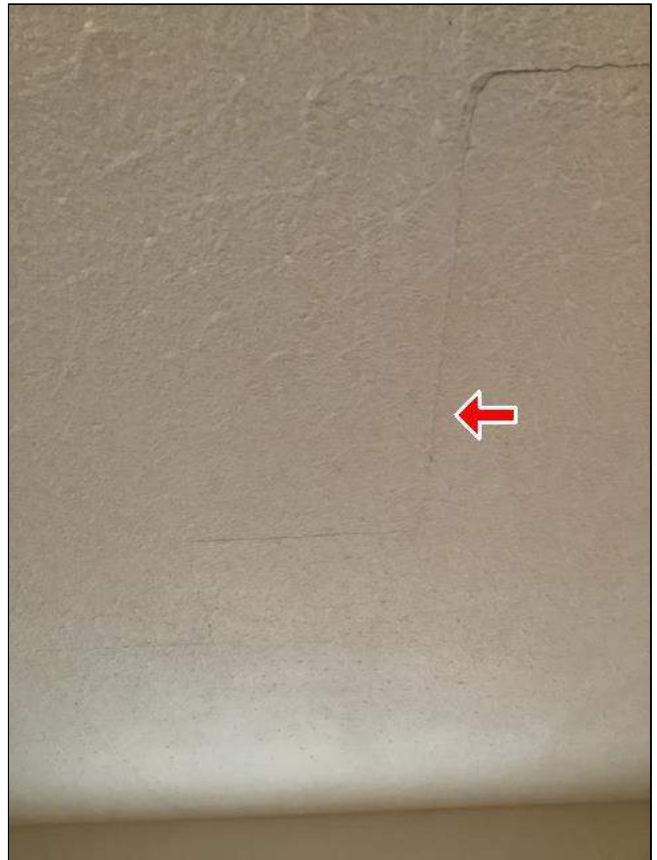
5.0 Item 6(Picture) Ceiling - common cracks from settling and shifting
