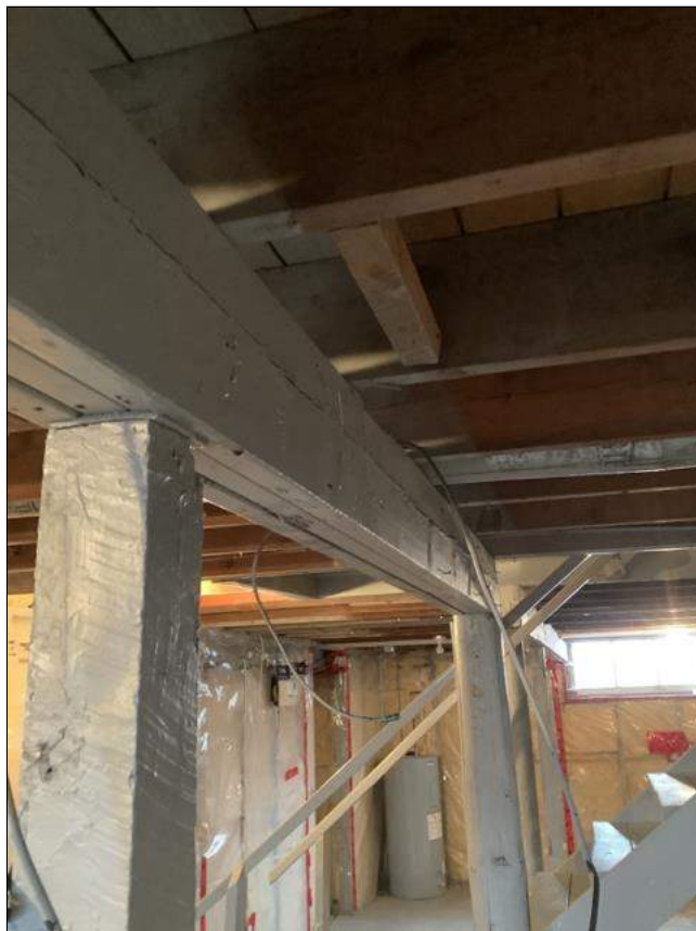
7.9 Item 2(Picture) Joists and Beams - slanted, crooked, notched out, bowed, split
