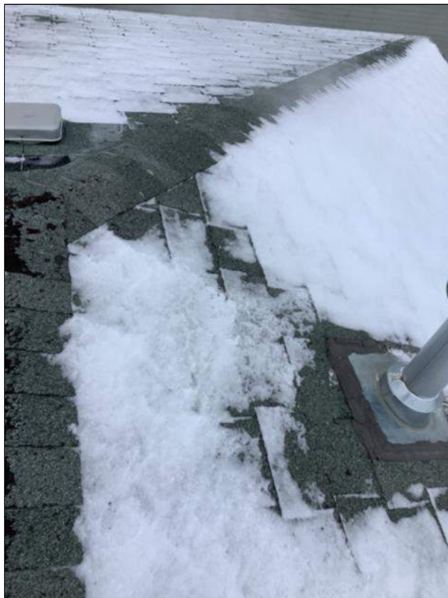
1.0 Item 2(Picture) Roof - shingles are aged and will require replacement
