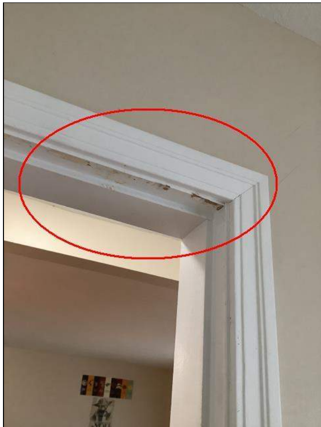
5.4 Item 1(Picture) Door - signs of rubbing
