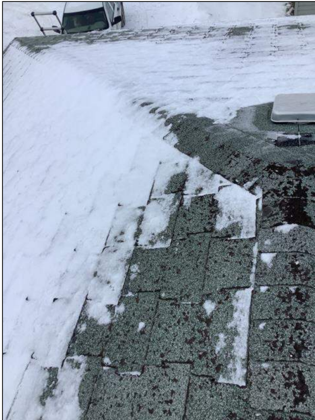
1.0 Item 1(Picture) Roof - shingles are aged and will require replacement
