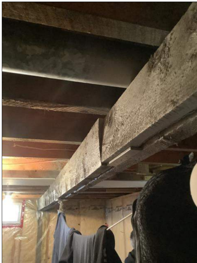
7.9 Item 24(Picture) Joists and Beams - slanted, crooked, notched out, bowed, split
