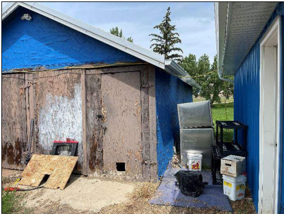
PHOTOGRAPH #16: Stucco - Shed SE Corner (2% Chrysotile)
