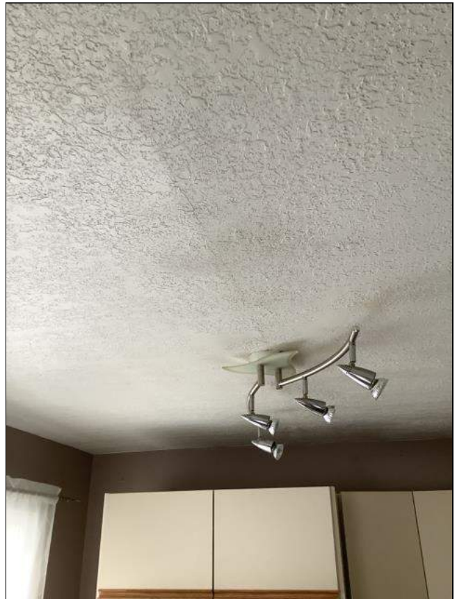
5.0 Item 6(Picture) Ceiling - signs of moisture damage, patching, stressed seams
