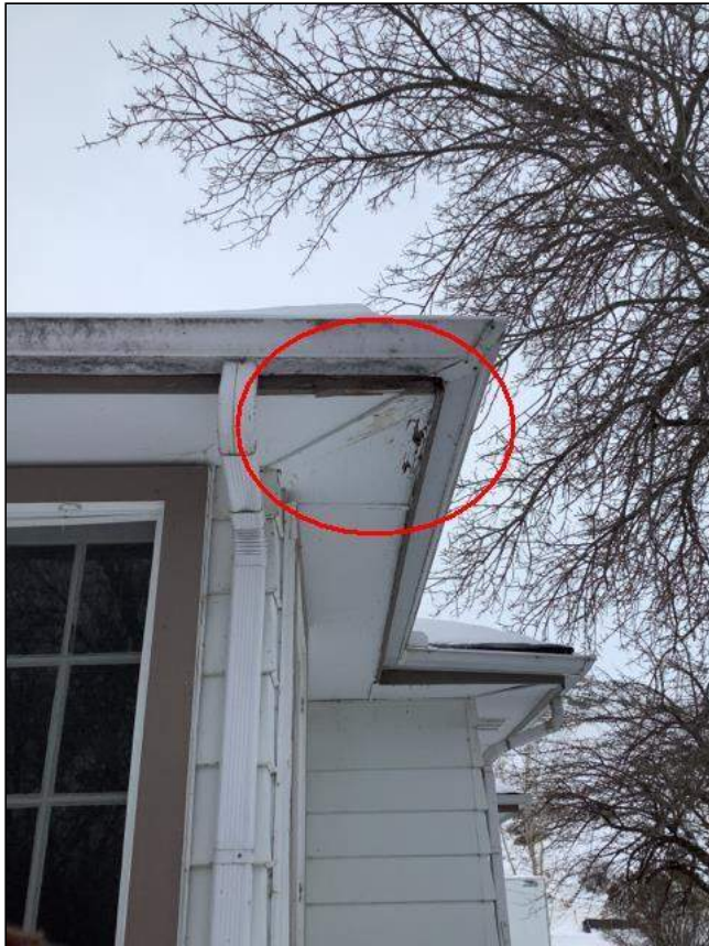
3.1 Item 1(Picture) Exterior - signs of moisture damage
