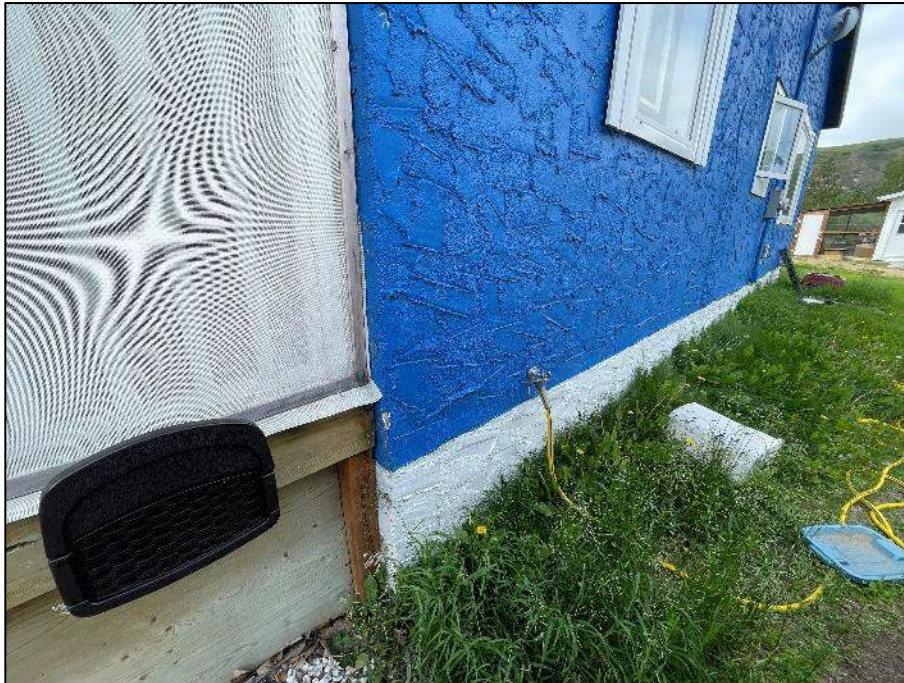
PHOTOGRAPH #13: Stucco - Exterior NE Corner (Assume Positive)
