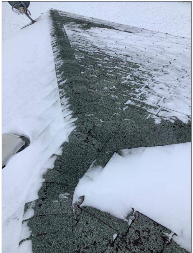
1.0 Item 8(Picture) Roof - shingles are aged and will require replacement
