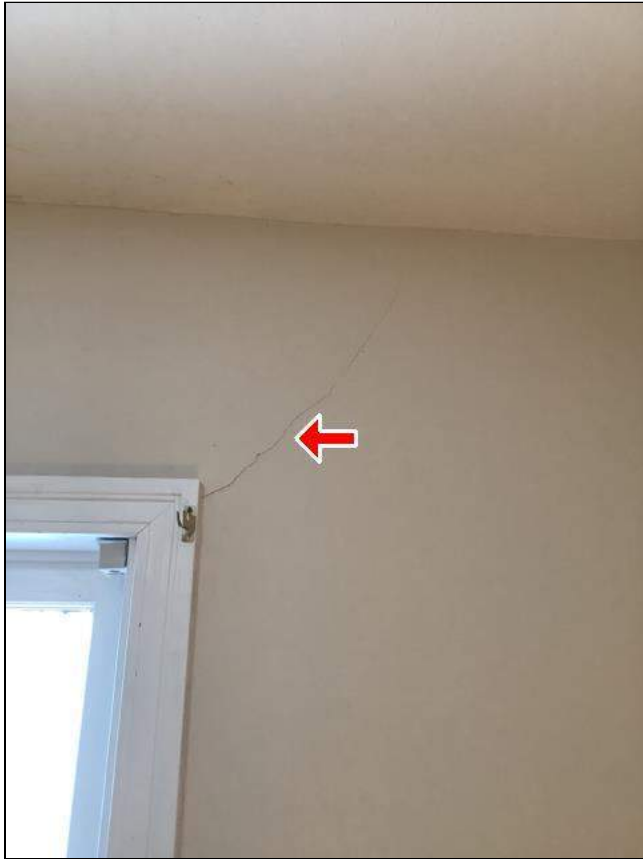
5.1 Item 1(Picture) Interior Walls - cracks from settling and shifting
