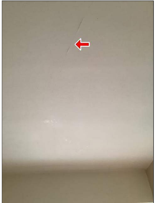
9.0 Item 2(Picture) Bathroom Ceiling - cracks from settling
