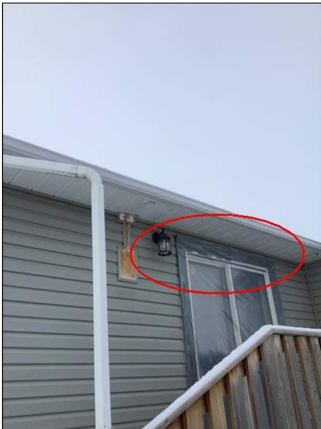
3.1 Item 9(Picture) Exterior Siding - bowed
