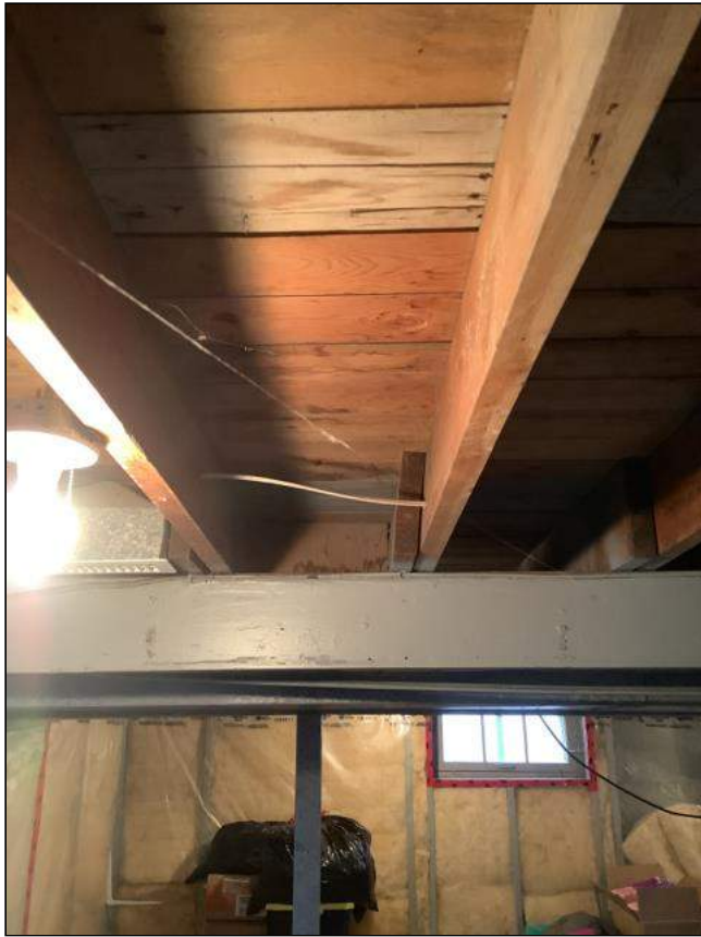
7.9 Item 5(Picture) Joists and Beams - slanted, crooked, notched out, bowed, split
