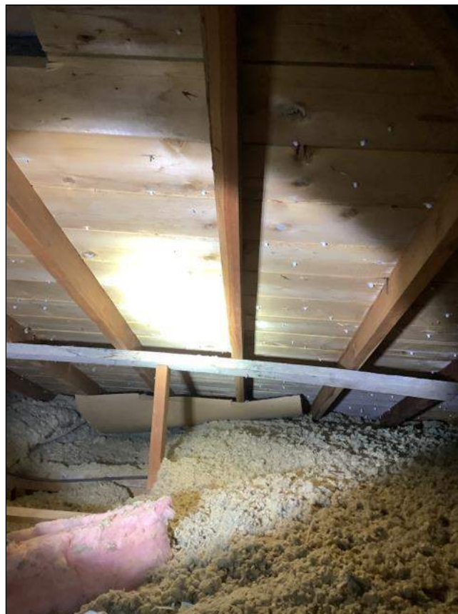
2.3 Item 2(Picture) Rafter - split, cross support bowed
