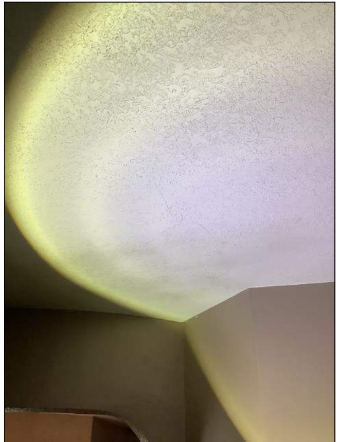
5.0 Item 8(Picture) Ceiling - signs of moisture damage, patching, stressed seams
