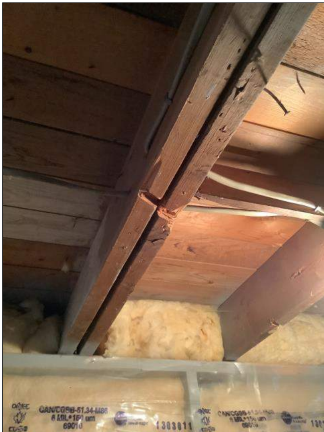
7.9 Item 15(Picture) Joists and Beams - slanted, crooked, notched out, bowed, split
