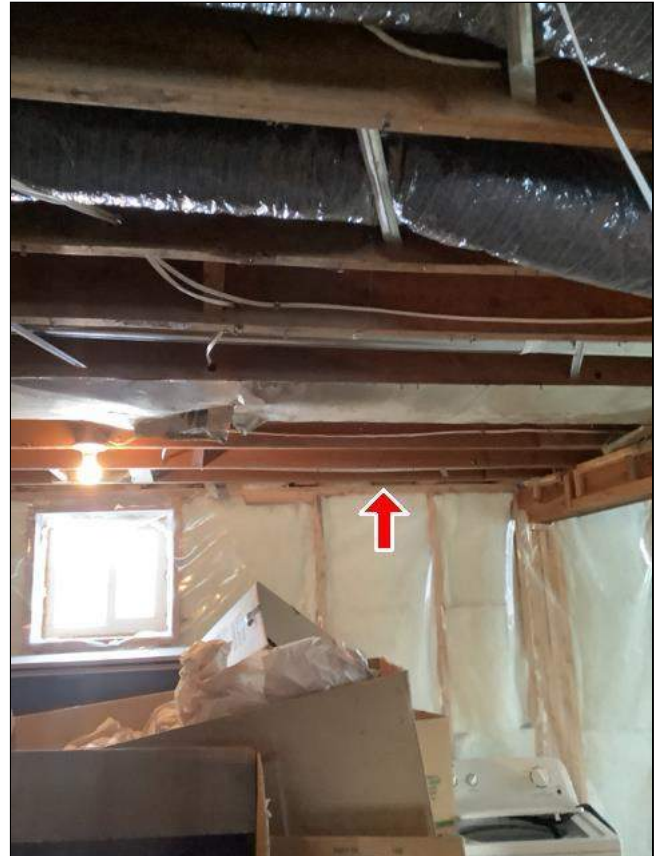
7.9 Item 2(Picture) Joist - sagging
