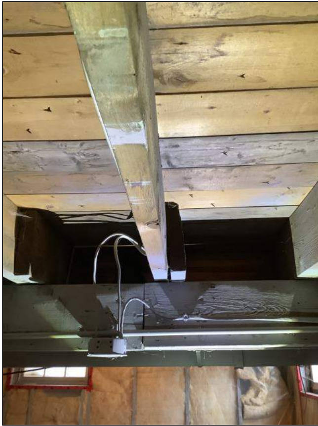
7.9 Item 13(Picture) Joists and Beams - slanted, crooked, notched out, bowed, split
