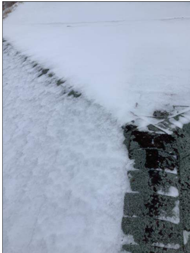
1.0 Item 6(Picture) Roof - shingles are aged and will require replacement
