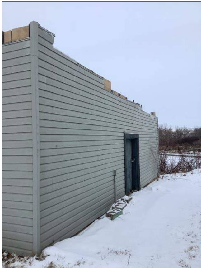
4.4 Item 1(Picture) Back of Garage - heavily bowed
