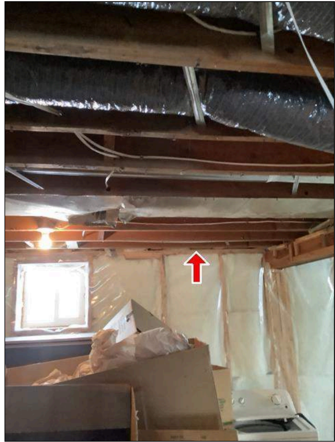
7.9 Item 2(Picture) Joist - sagging
