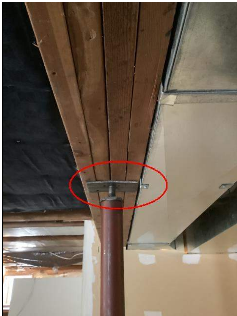
7.6 Item 1(Picture) Plate - bowed
