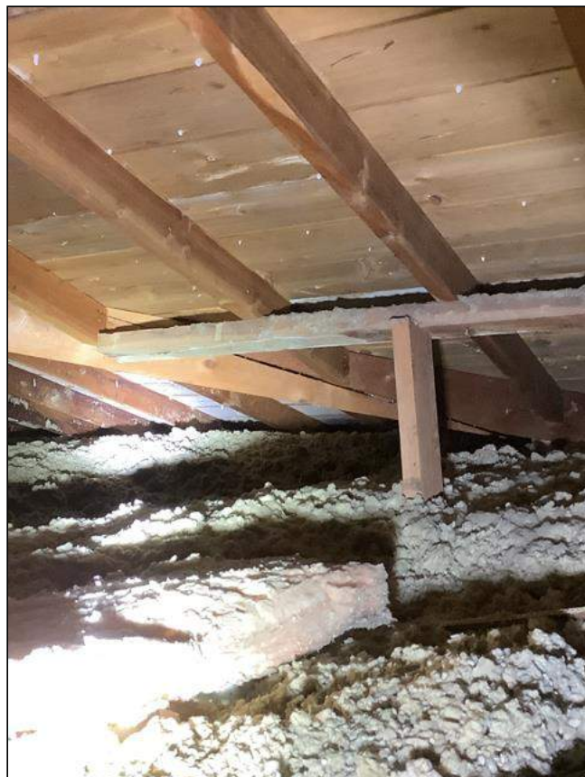
2.3 Item 1(Picture) Rafter - split, cross support bowed
