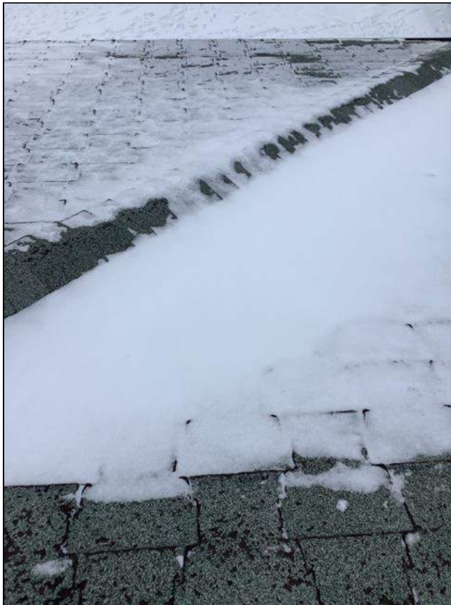
1.0 Item 9(Picture) Roof - shingles are aged and will require replacement
