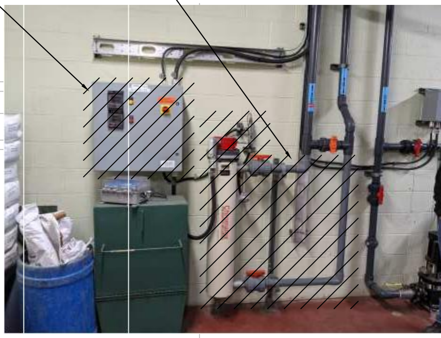
PICTURE #1 - HOT WATER EQUIPMENT
