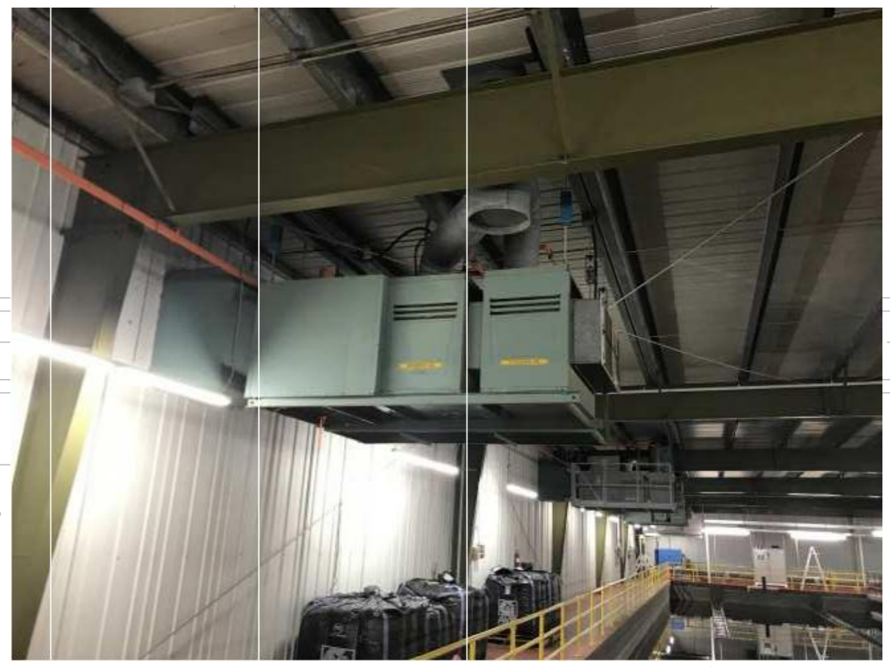
PICTURE #2 TYPICAL EXISTING MAKE UP AIR UNIT (7)- UPPER
