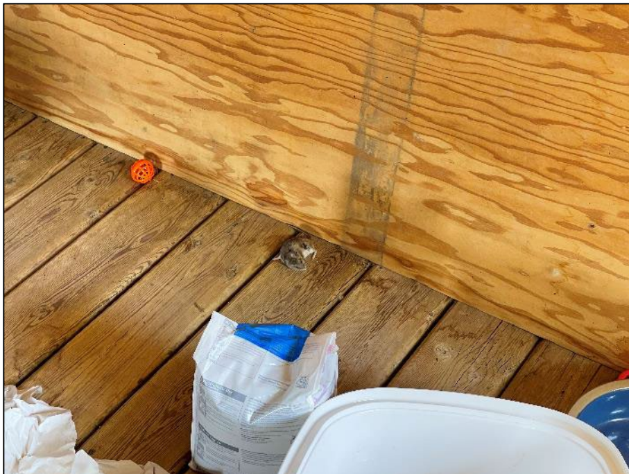
PHOTOGRAPH #24: Animal Carcass on Front Porch (Biological Hazard)
