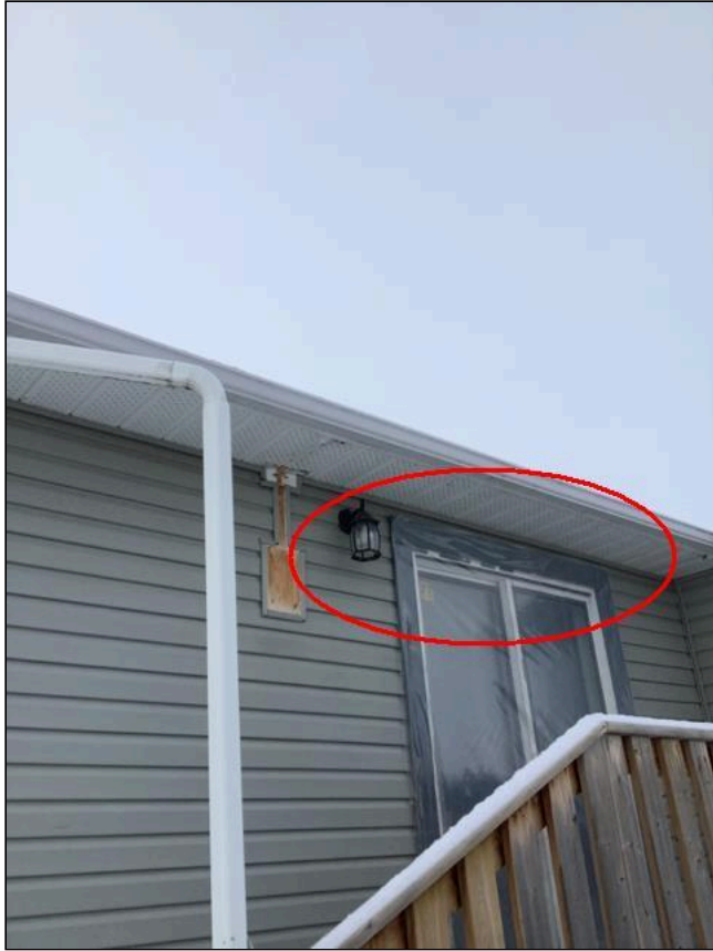
3.1 Item 9(Picture) Exterior Siding - bowed
