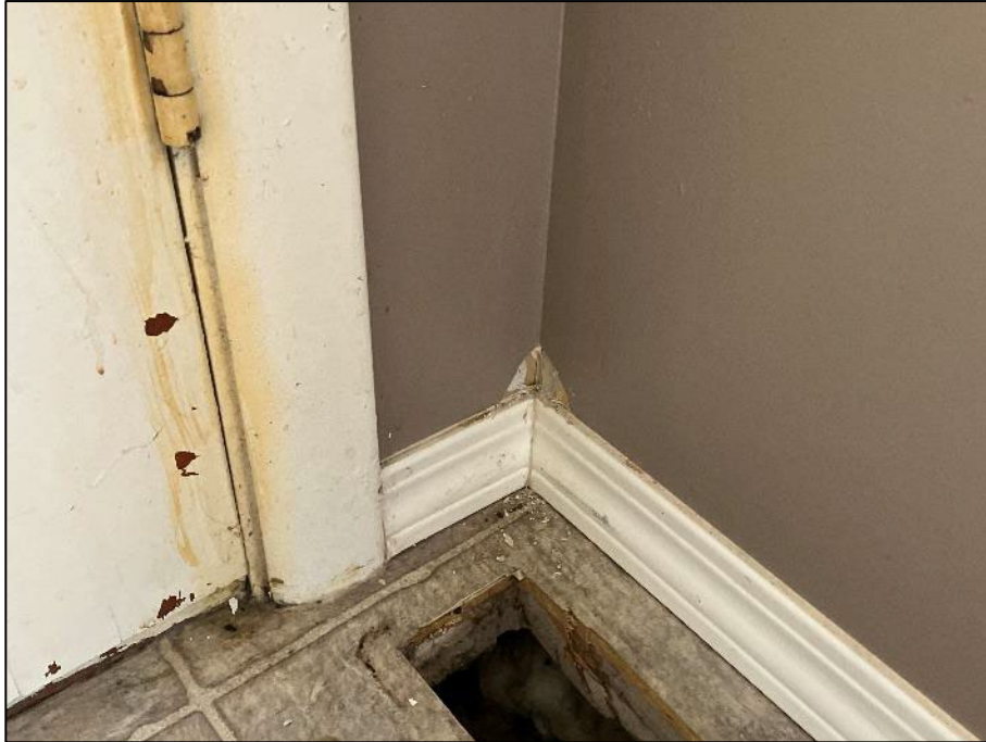
PHOTOGRAPH #3: Drywall Joint Compound – Floor 1 Ext Kitchen (2% Chrysotile)
