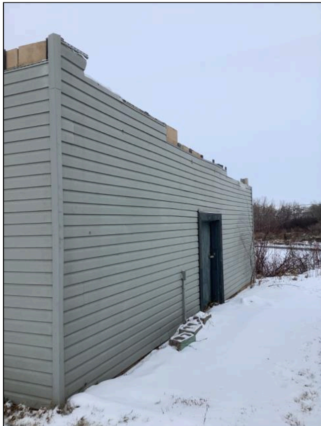
4.4 Item 1(Picture) Back of Garage - heavily bowed
