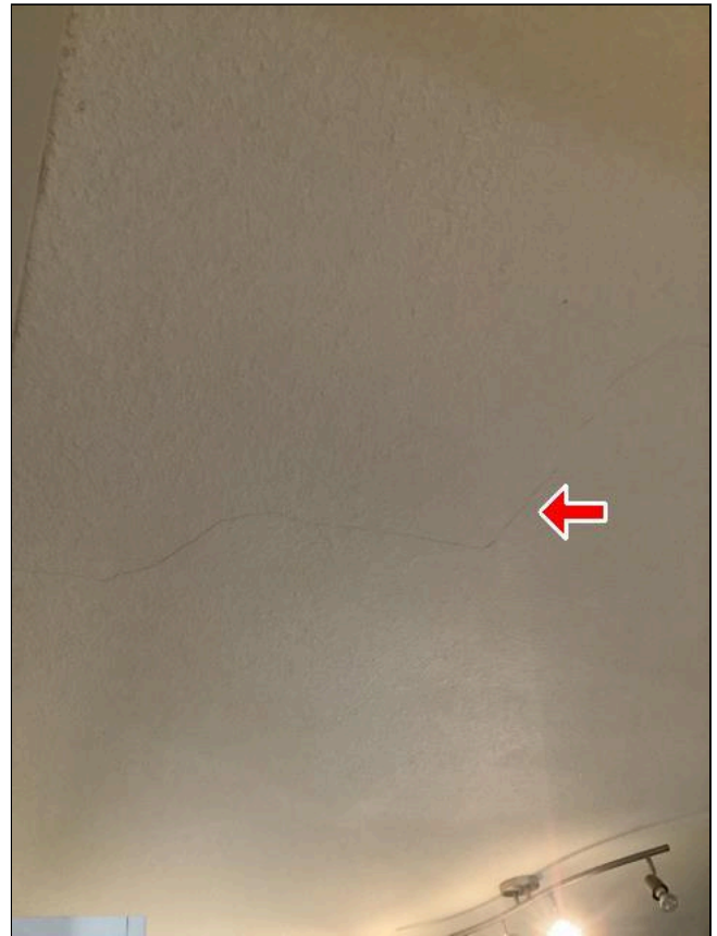
5.0 Item 8(Picture) Ceiling - common cracks from settling and shifting
