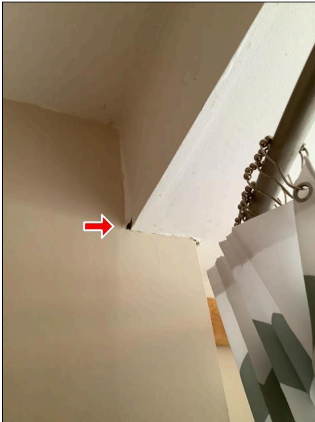
5.1 Item 9(Picture) Interior Walls - cracks from settling and shifting
