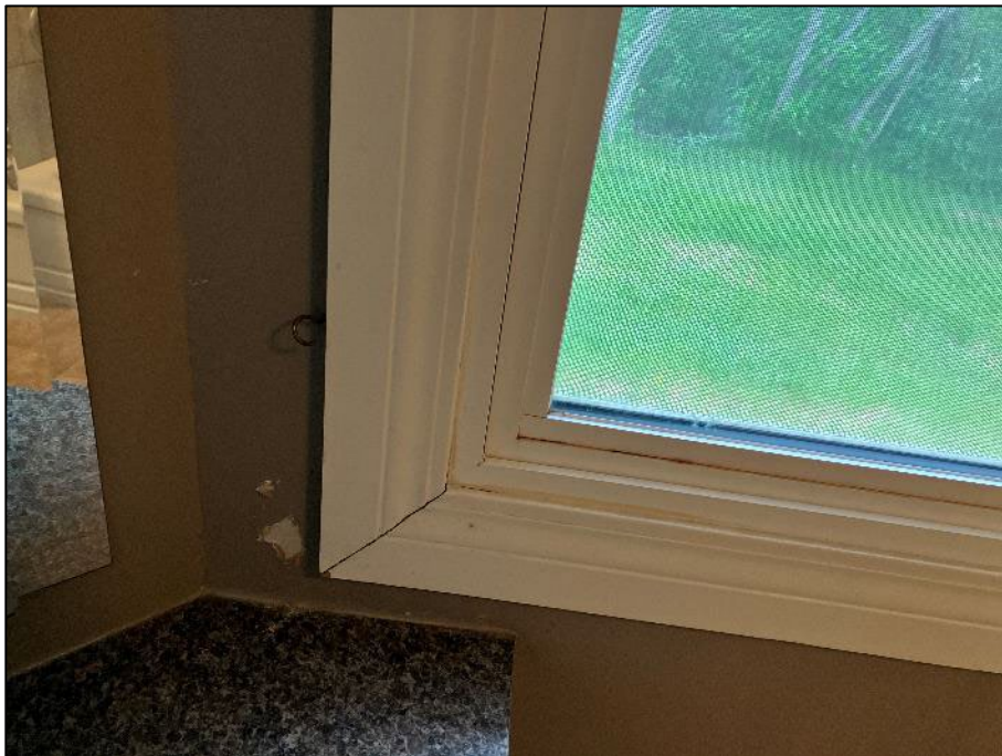
PHOTOGRAPH #6: Drywall Joint Compound – Floor 1 Ext Bathroom (Assume Positive)
