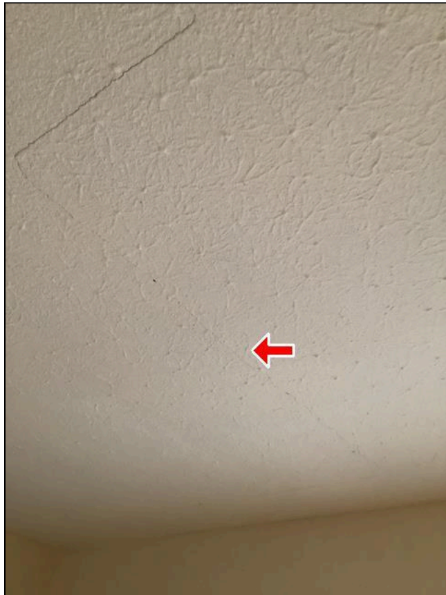
5.0 Item 7(Picture) Ceiling - common cracks from settling and shifting
