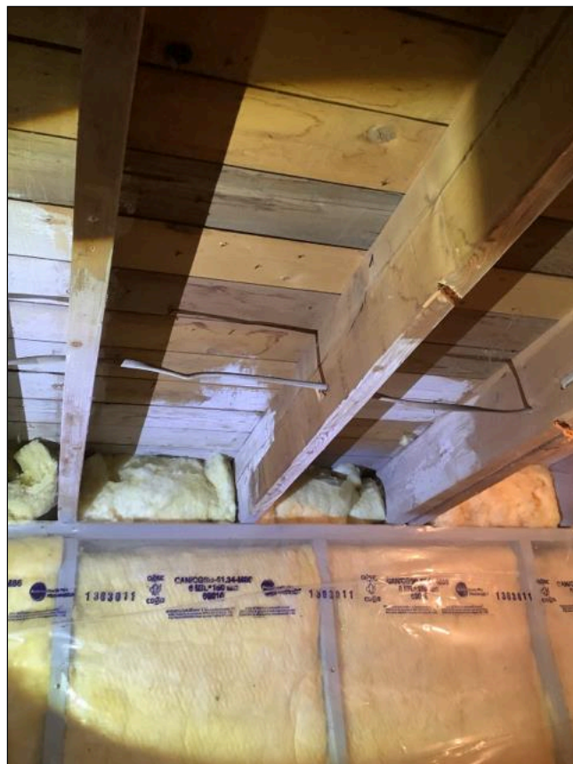
7.9 Item 8(Picture) Joists and Beams - slanted, crooked, notched out, bowed, split
