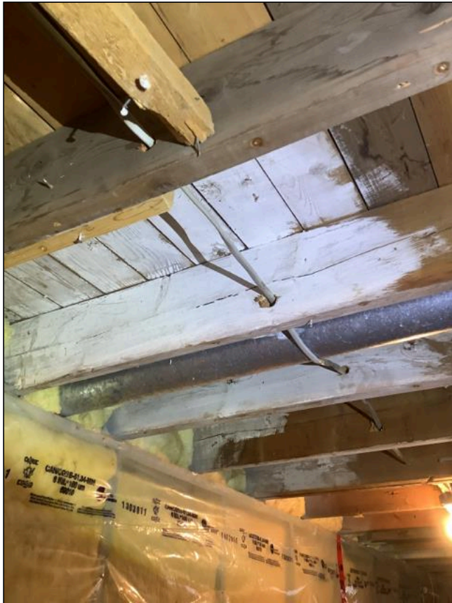
7.9 Item 9(Picture) Joists and Beams - slanted, crooked, notched out, bowed, split
