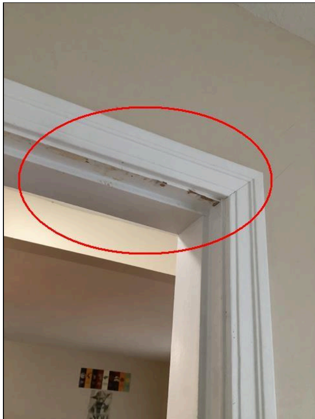
5.4 Item 1(Picture) Door - signs of rubbing
