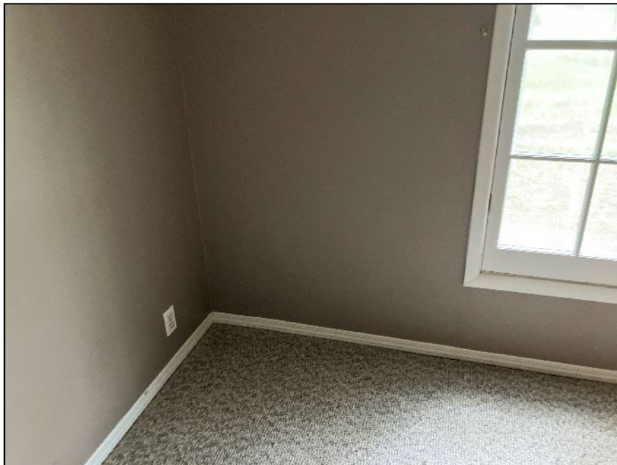
PHOTOGRAPH #8: Drywall Joint Compound – Floor 1 Ext NE Bedroom (2% Chrysotile)
