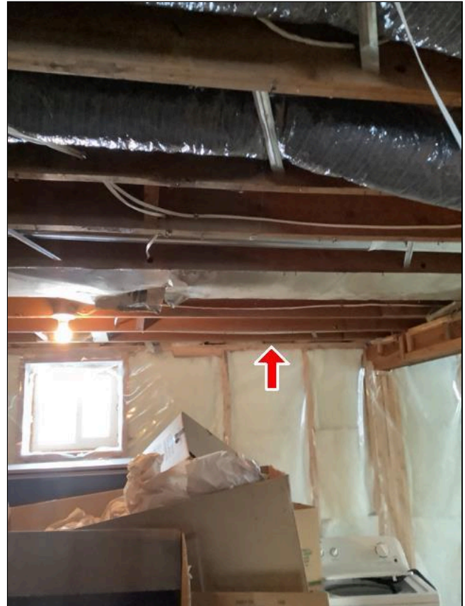
7.9 Item 2(Picture) Joist - sagging
