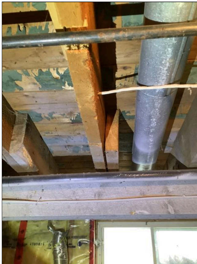
7.9 Item 28(Picture) Joists and Beams - slanted, crooked, notched out, bowed, split
