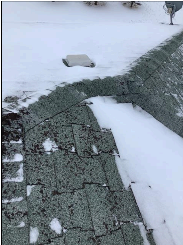
1.0 Item 7(Picture) Roof - shingles are aged and will require replacement
