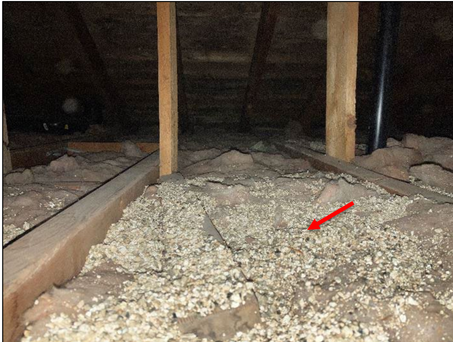
PHOTOGRAPH #21: Vermiculite in the Attic Space (<1% Tremolite)
