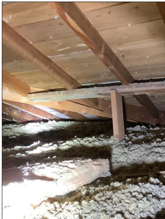
2.3 Item 1(Picture) Rafter - split, cross support bowed
