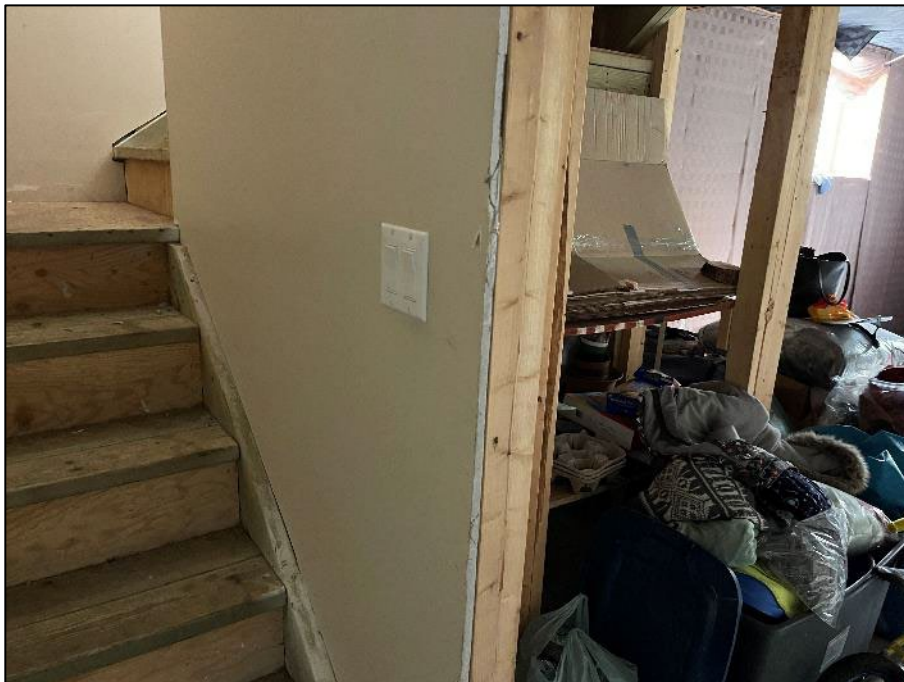
PHOTOGRAPH #16: Drywall Joint Compound - Basement Stairs (Non-Asbestos)
