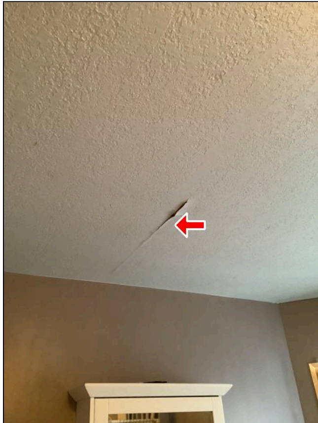
9.0 Item 1(Picture) Bathroom Ceiling - seam splitting
