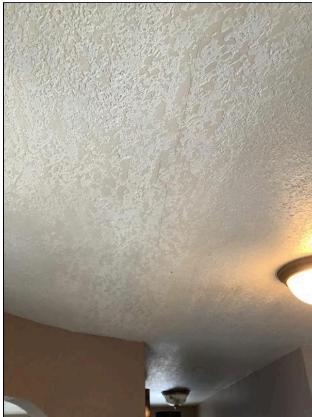
5.0 Item 1(Picture) Ceiling - signs of moisture damage, patching, stressed seams
