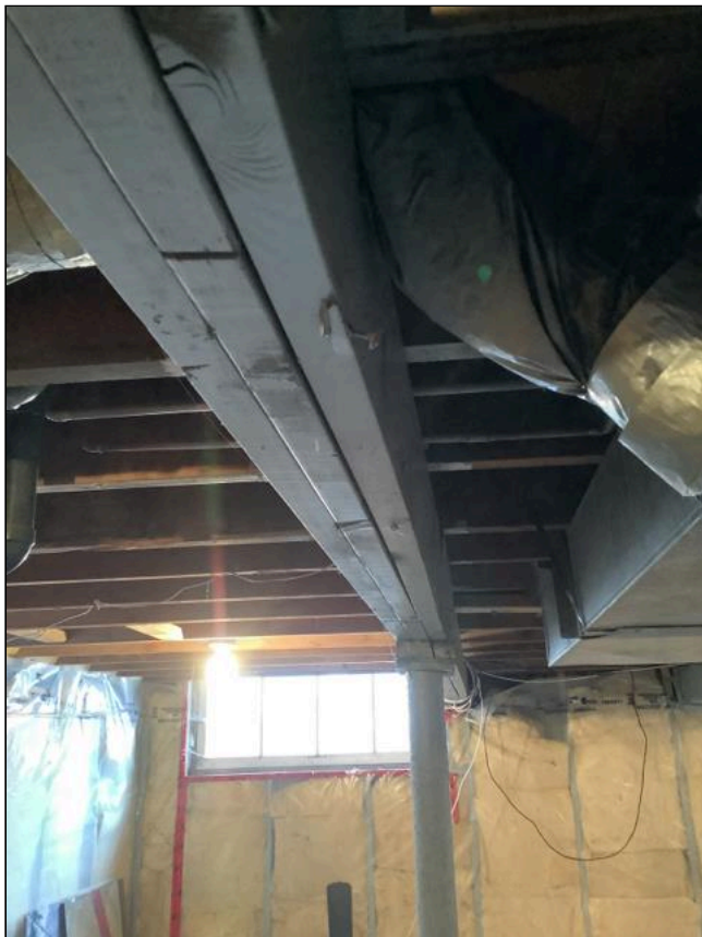
7.9 Item 3(Picture) Joists and Beams - slanted, crooked, notched out, bowed, split
