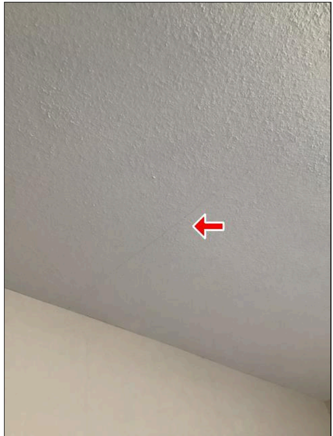
5.0 Item 2(Picture) Ceiling - common cracks from settling and shifting
