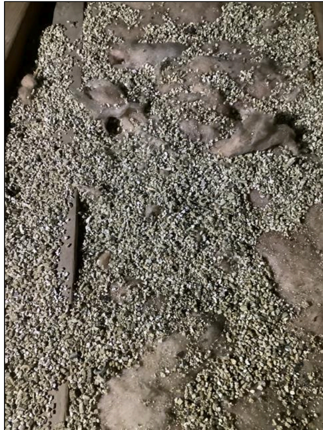
2.4 Item 1(Picture) Attic Insulation - vermiculite
