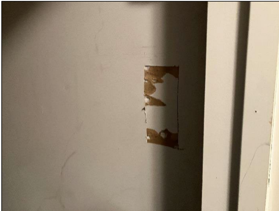
PHOTOGRAPH #23: Paint – White Stairs (Non-Lead Based)
