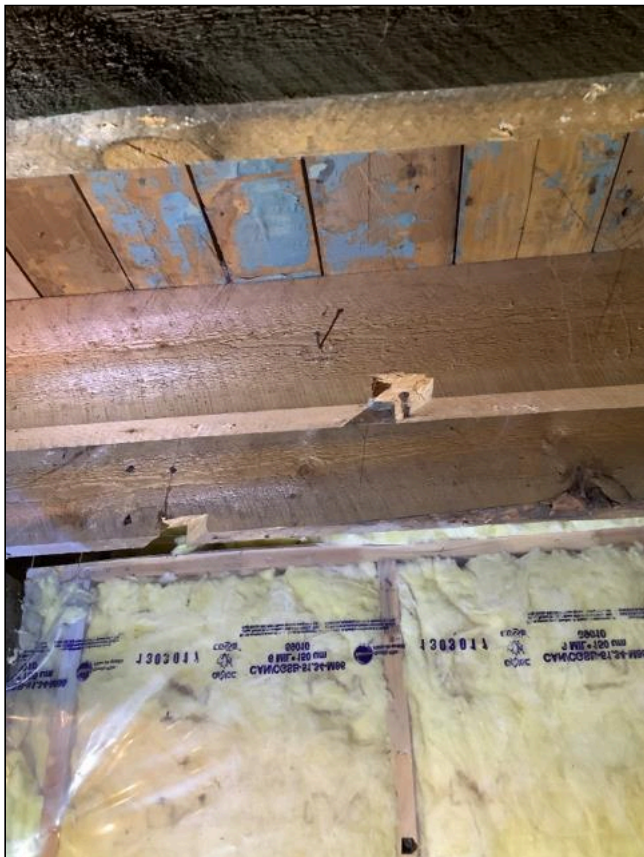
7.9 Item 27(Picture) Joists and Beams - slanted, crooked, notched out, bowed, split
