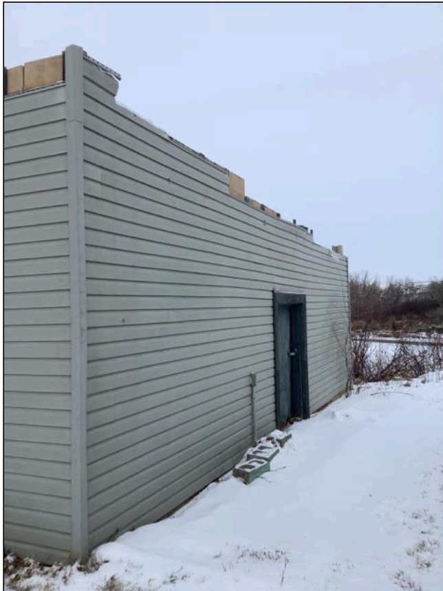
4.4 Item 1(Picture) Back of Garage - heavily bowed
