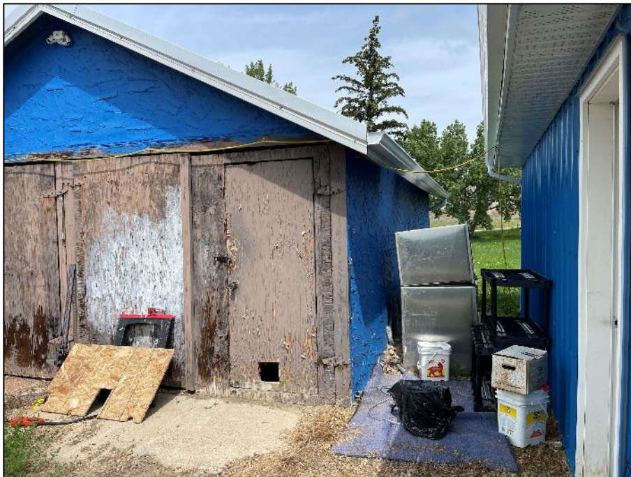
PHOTOGRAPH #16: Stucco - Shed SE Corner (2% Chrysotile)
