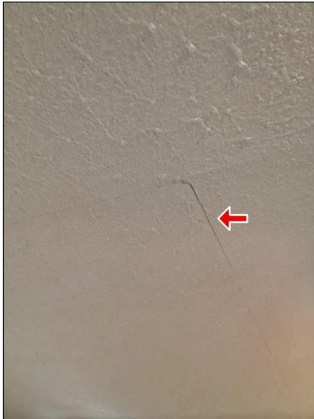
5.0 Item 5(Picture) Ceiling - common cracks from settling and shifting
