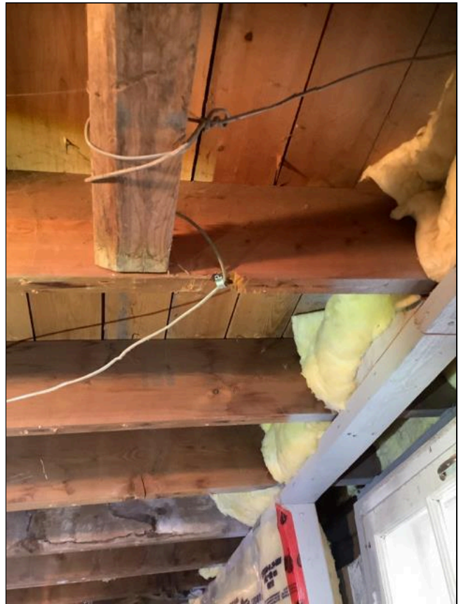
7.9 Item 18(Picture) Joists and Beams - slanted, crooked, notched out, bowed, split
