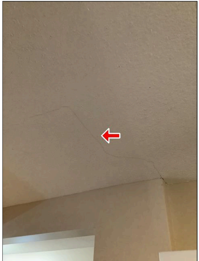
5.0 Item 4(Picture) Ceiling - common cracks from settling and shifting
