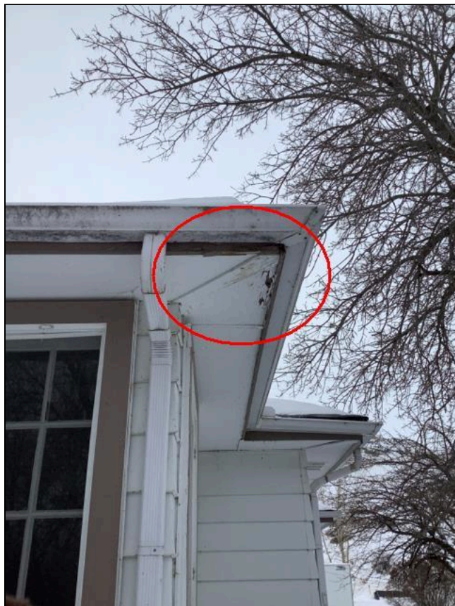
3.1 Item 1(Picture) Exterior - signs of moisture damage
