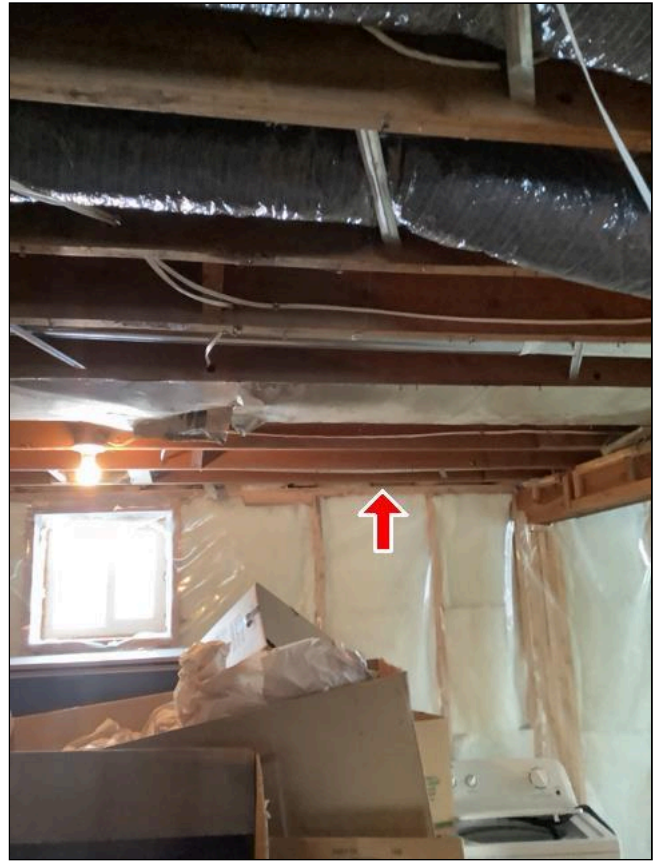
7.9 Item 2(Picture) Joist - sagging
