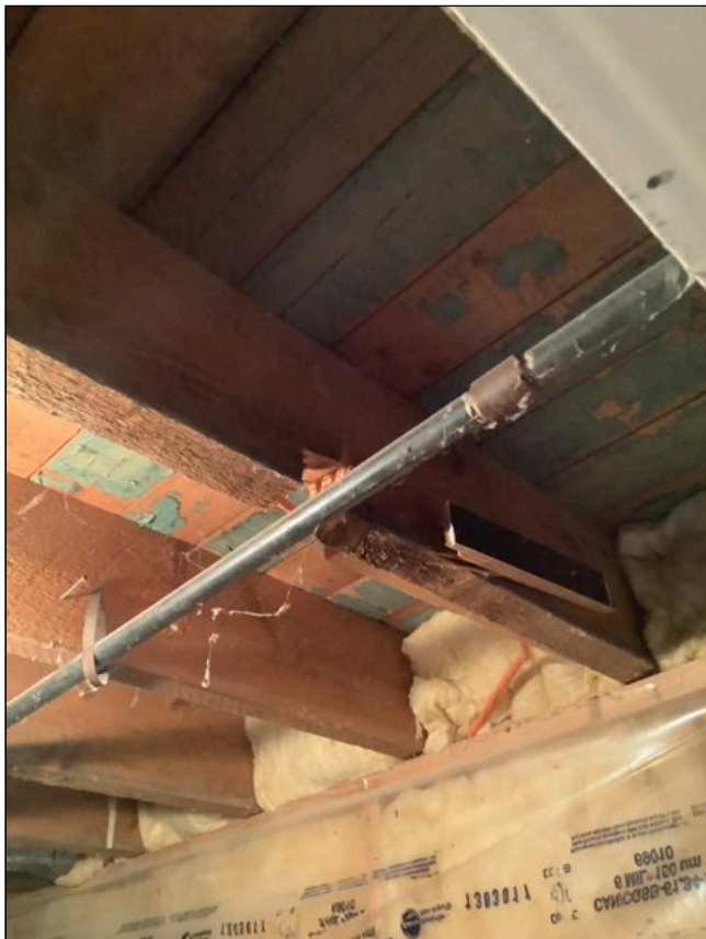
7.9 Item 23(Picture) Joists and Beams - slanted, crooked, notched out, bowed, split
