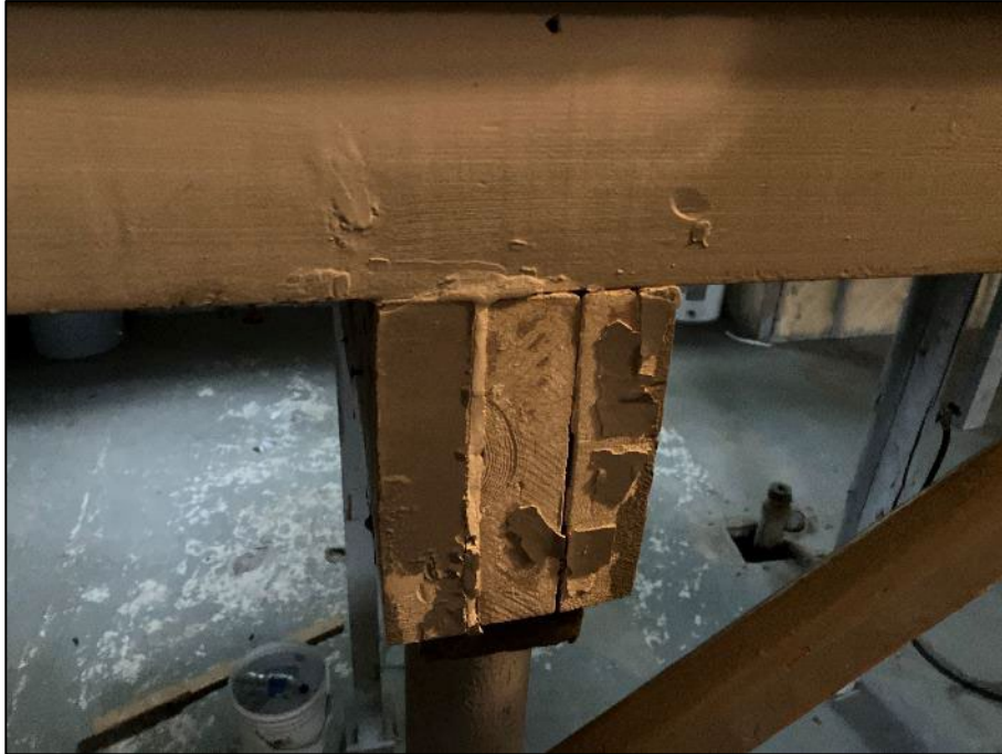
PHOTOGRAPH #7: Drywall Joint Compound – Basement Int Stairs (Assume Positive)
