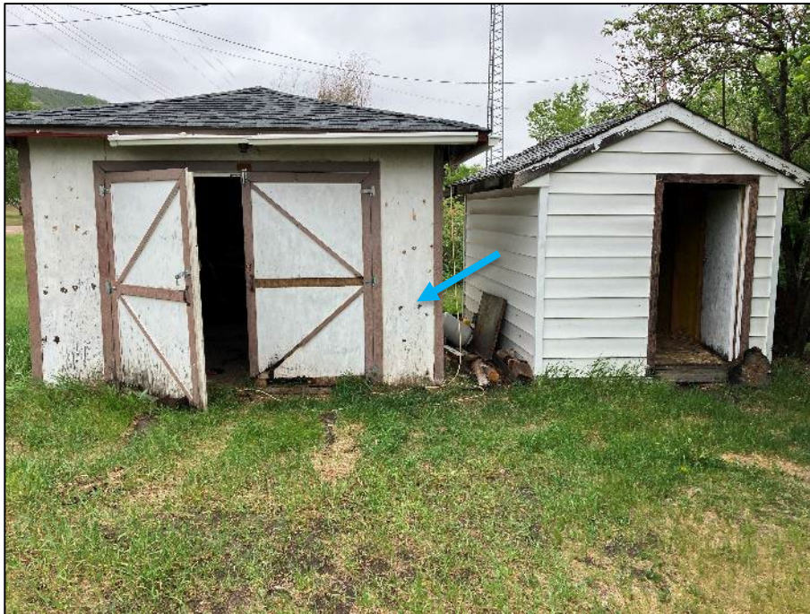
PHOTOGRAPH #27: Paint – White Shed (Non-Lead Based)
