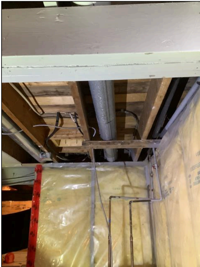
7.9 Item 7(Picture) Joists and Beams - slanted, crooked, notched out, bowed, split
