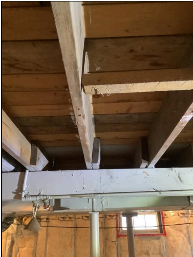
7.9 Item 11(Picture) Joists and Beams - slanted, crooked, notched out, bowed, split
