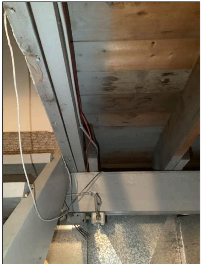
7.9 Item 16(Picture) Joists and Beams - slanted, crooked, notched out, bowed, split
