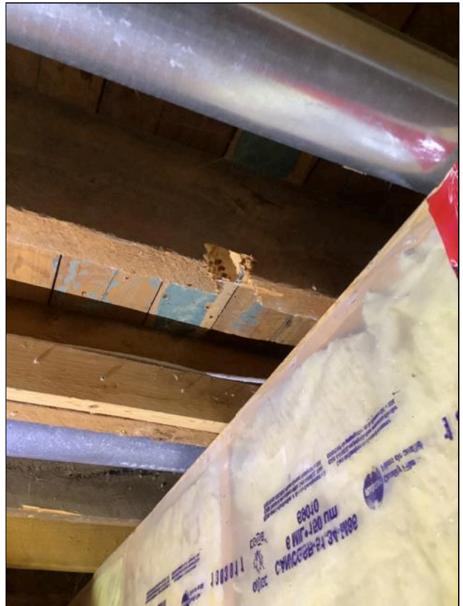
7.9 Item 26(Picture) Joists and Beams - slanted, crooked, notched out, bowed, split
