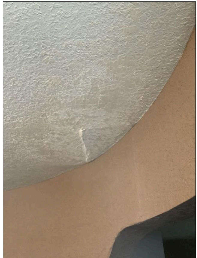
5.0 Item 2(Picture) Ceiling - signs of moisture damage, patching, stressed seams
