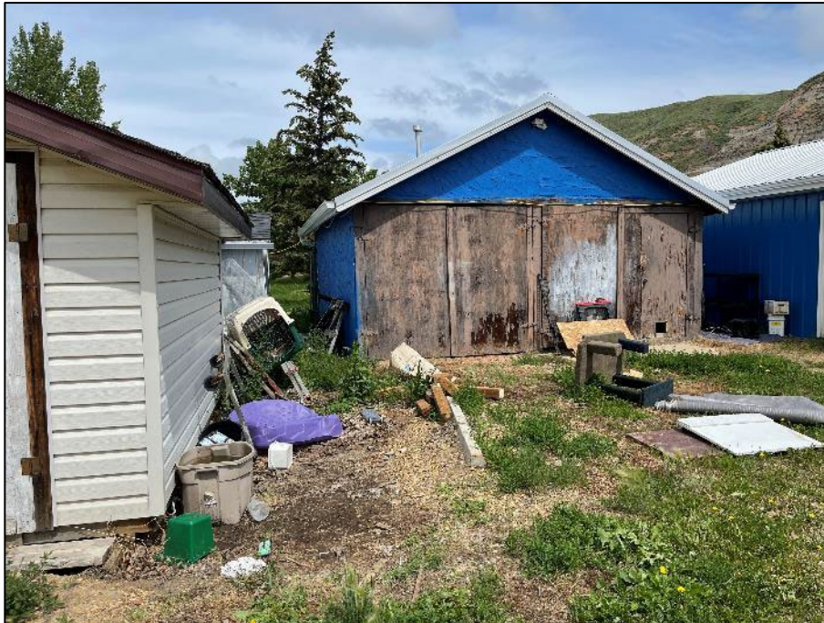
PHOTOGRAPH #17: Stucco - Shed SW Corner (2% Chrysotile)
