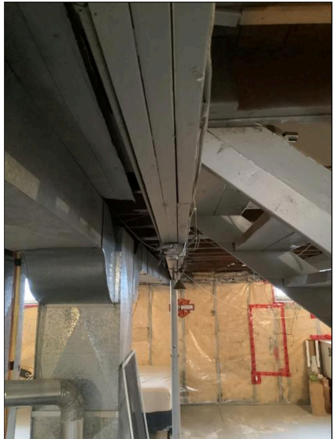
7.9 Item 4(Picture) Joists and Beams - slanted, crooked, notched out, bowed, split
