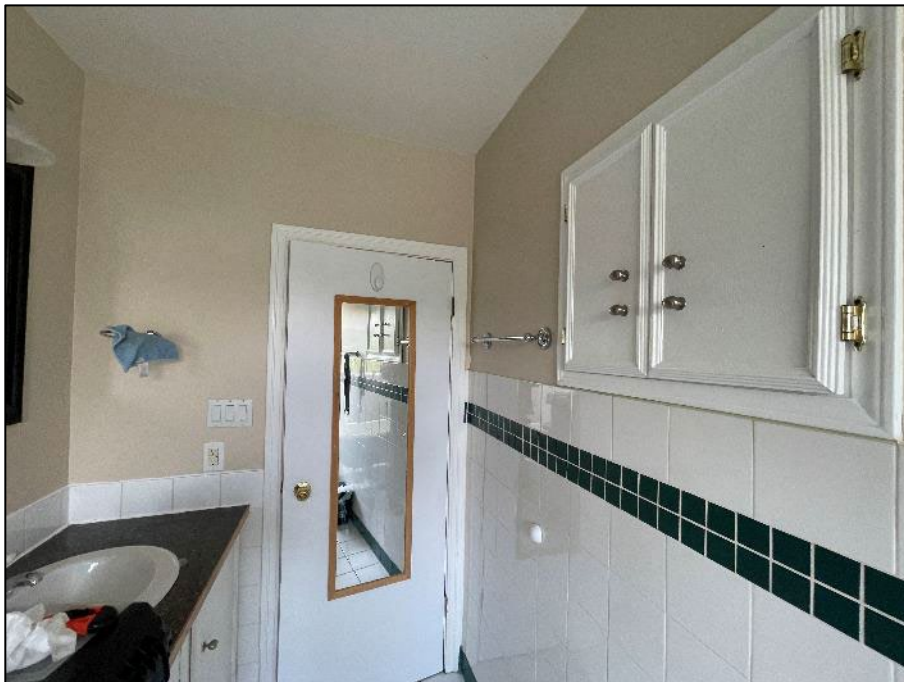
PHOTOGRAPH #6: Plaster - Level 1 Bathroom Interior (<1% Actinolite)
