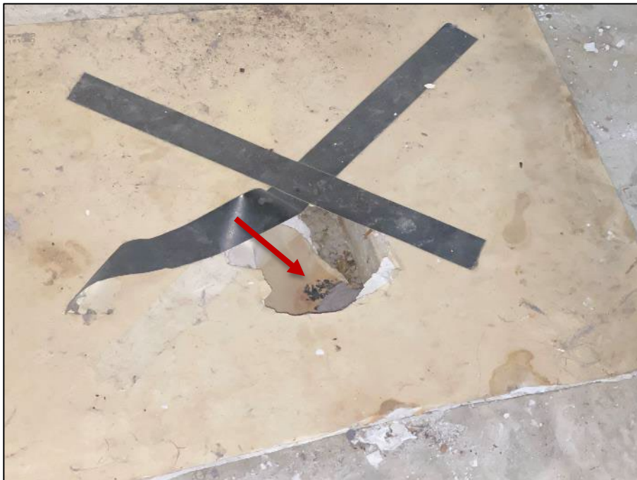
PHOTOGRAPH #26: Visible Mould Contamination - Basement Laundry Room (Biological Hazard)
