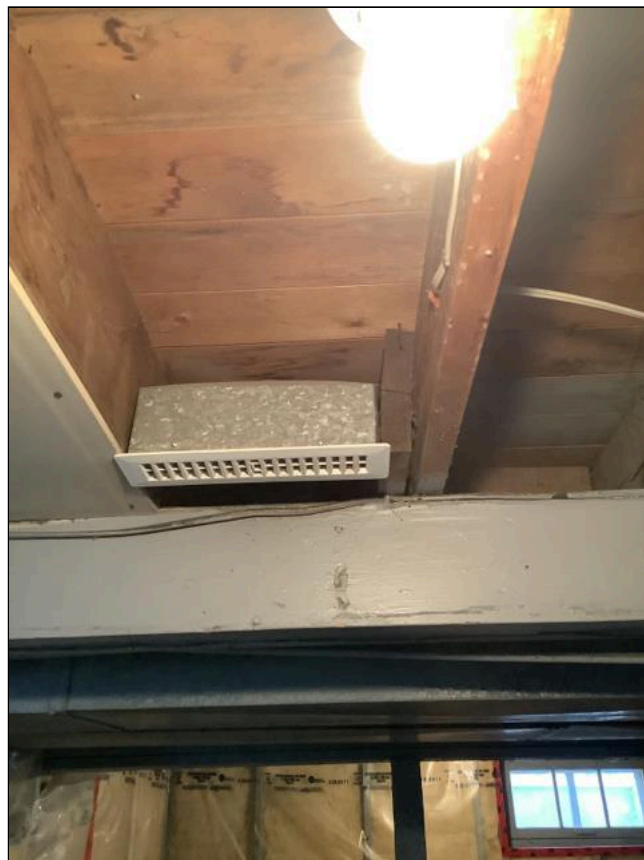
7.9 Item 6(Picture) Joists and Beams - slanted, crooked, notched out, bowed, split
