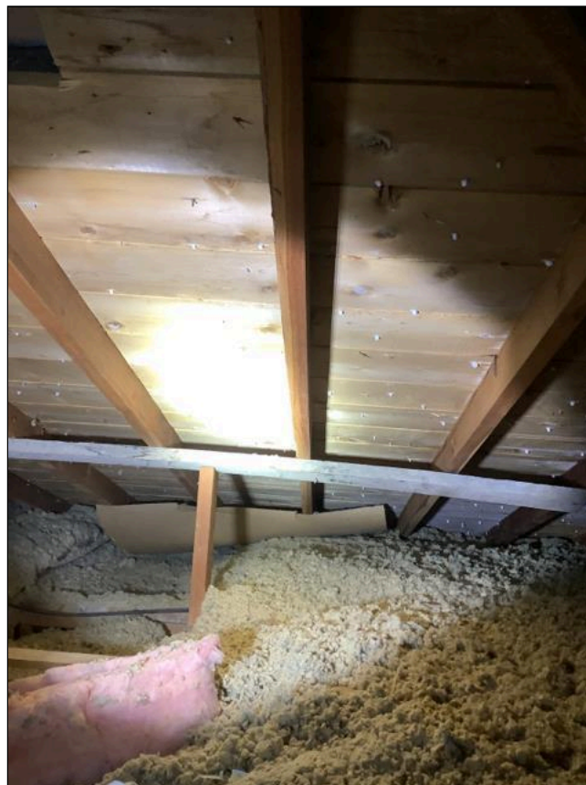
2.3 Item 2(Picture) Rafter - split, cross support bowed
