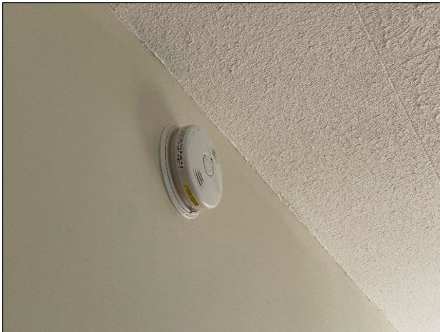
PHOTOGRAPH #24: Smoke Detector – Main Floor Living Room (Radioactive Materials)
