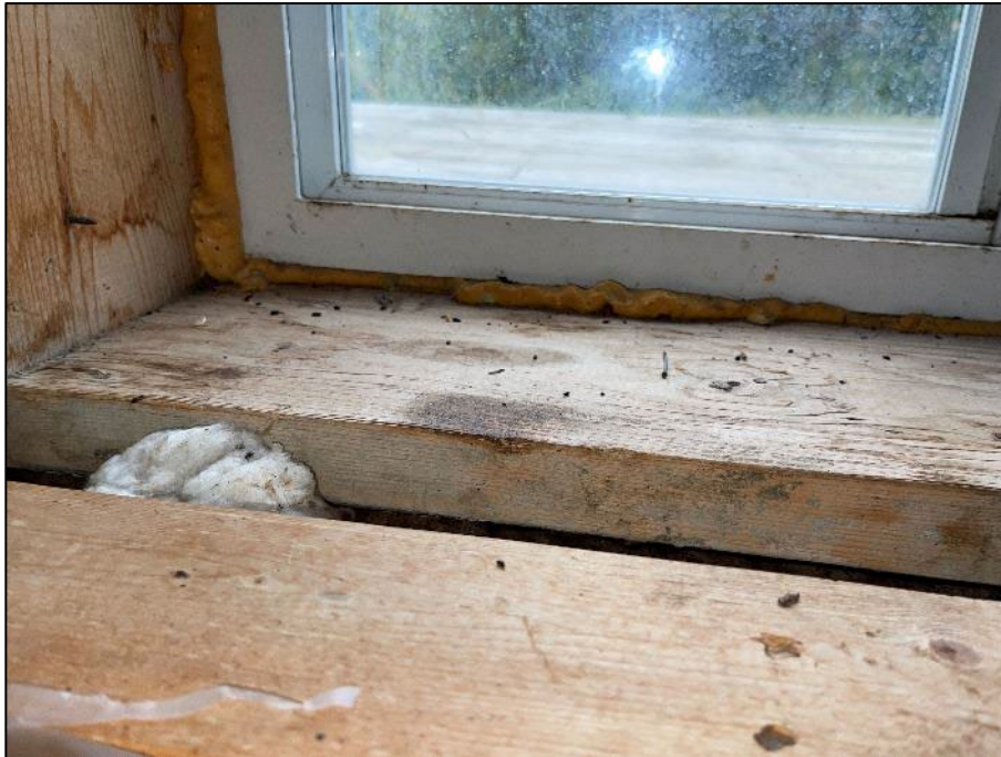
PHOTOGRAPH #25: Mouse Droppings Present in Basement Laundry Room (Biological Hazard)
