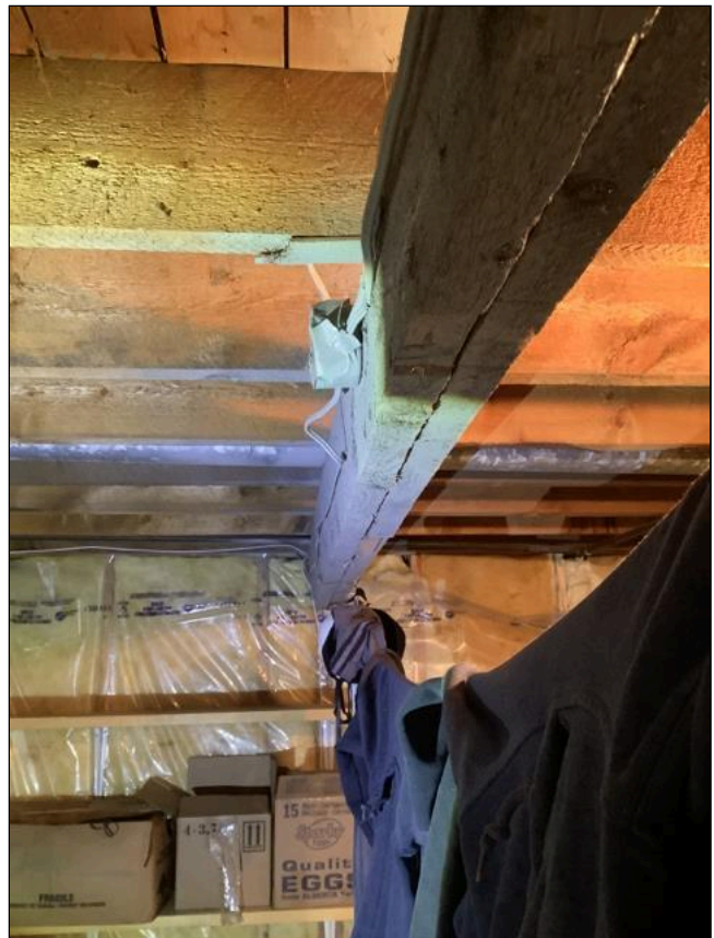
7.9 Item 20(Picture) Joists and Beams - slanted, crooked, notched out, bowed, split
