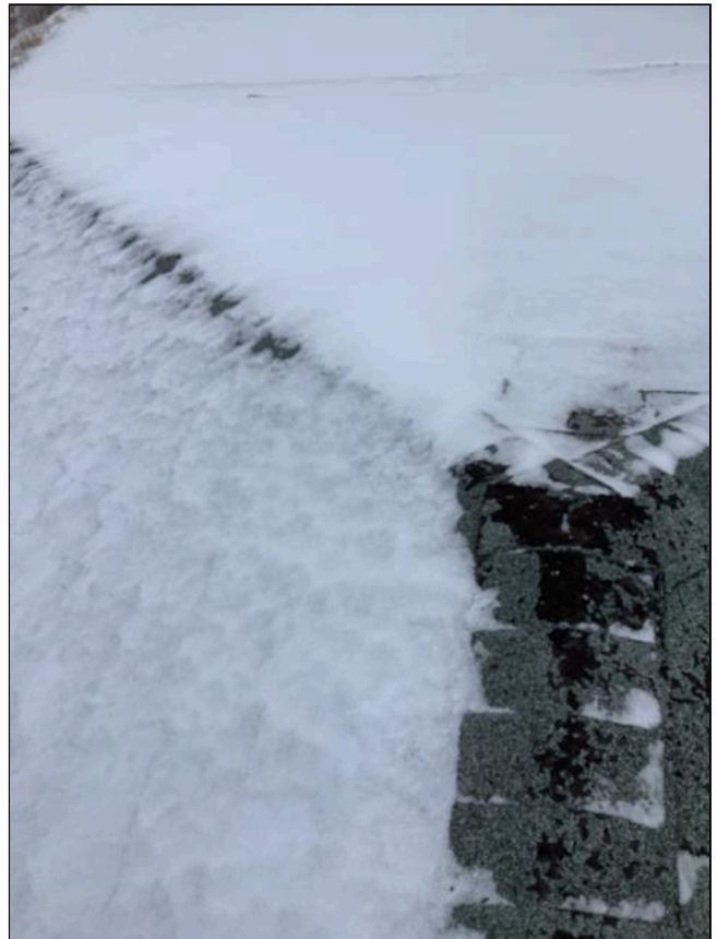
1.0 Item 6(Picture) Roof - shingles are aged and will require replacement
