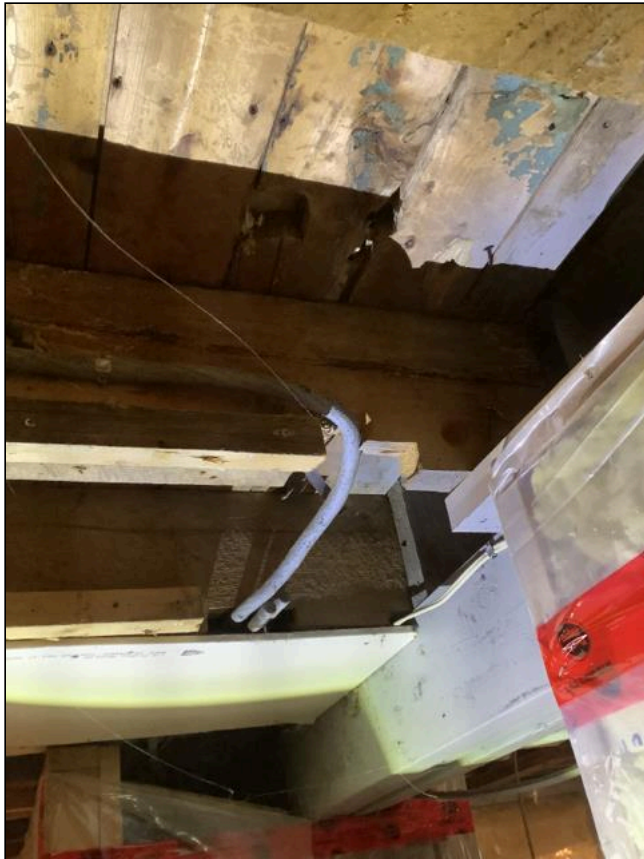
7.9 Item 25(Picture) Joists and Beams - slanted, crooked, notched out, bowed, split
