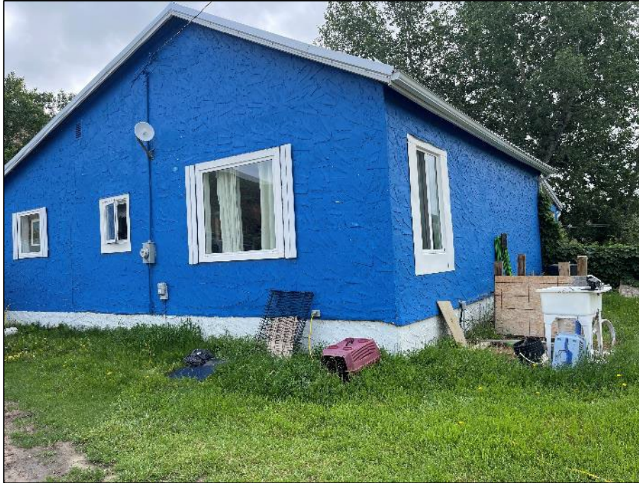
PHOTOGRAPH #15: Stucco - Exterior NW Corner (2% Chrysotile)
