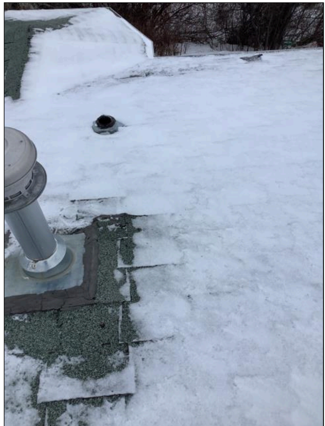
1.0 Item 4(Picture) Roof - shingles are aged and will require replacement
