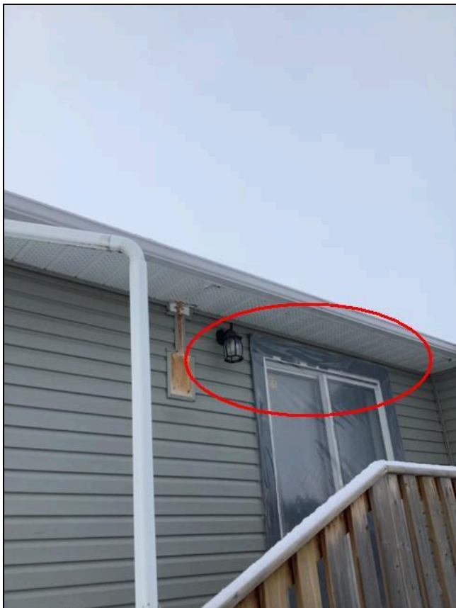
3.1 Item 9(Picture) Exterior Siding - bowed
