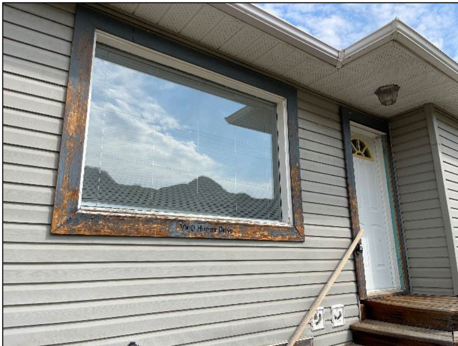
PHOTOGRAPH #22: White Paint – Exterior Trim (Lead Based)
