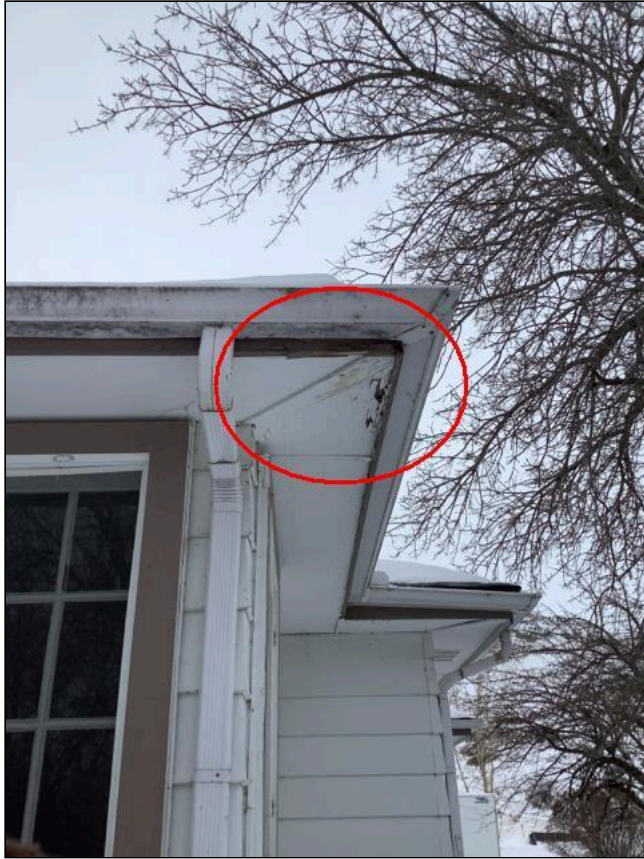
3.1 Item 1(Picture) Exterior - signs of moisture damage
