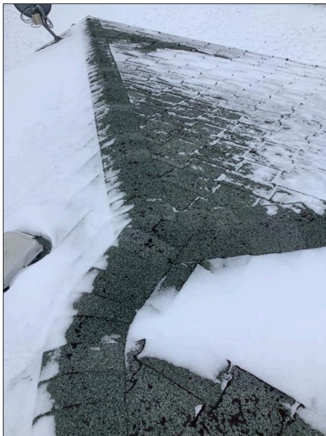
1.0 Item 8(Picture) Roof - shingles are aged and will require replacement
