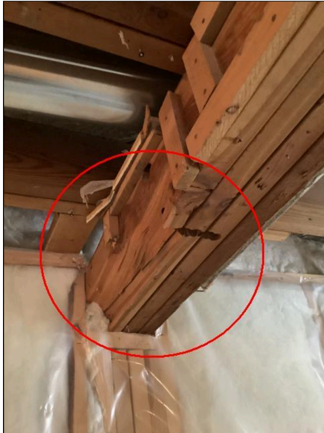
7.9 Item 1(Picture) Beam - end is broken
