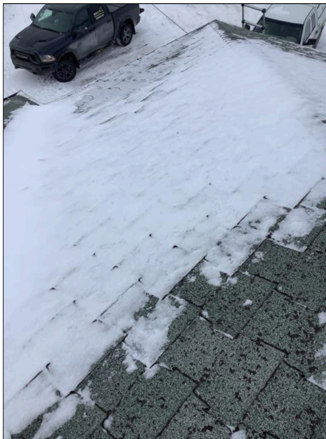
1.0 Item 10(Picture) Roof - shingles are aged and will require replacement
