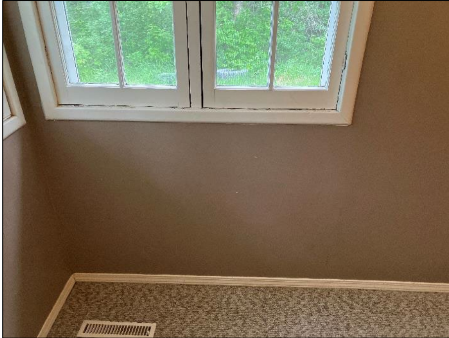
PHOTOGRAPH #5: Drywall Joint Compound – Floor 1 Ext NW Bedroom (Assume Positive)
