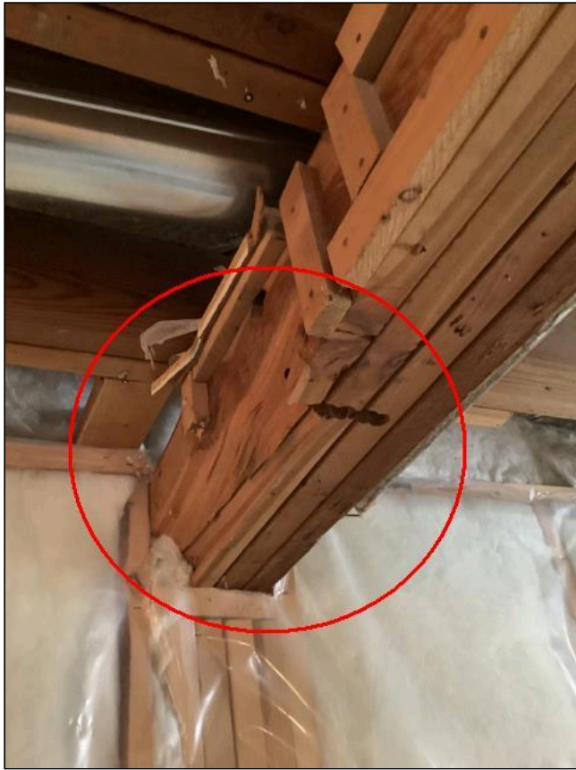
7.9 Item 1(Picture) Beam - end is broken
