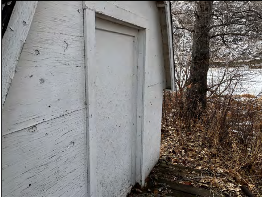
PHOTOGRAPH #21: Paint - Shed White (3400 ppm Lead)
