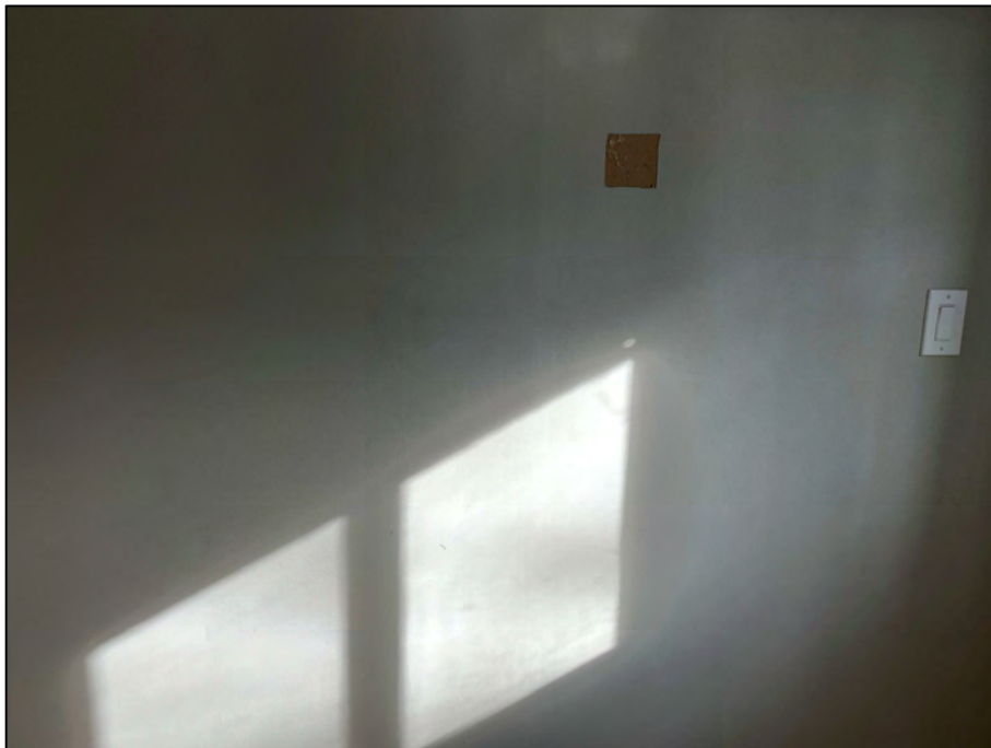
PHOTOGRAPH #18: Paint - Storage Room Beige (570 ppm Lead)
