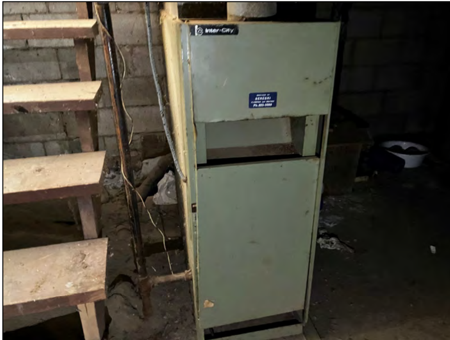
PHOTOGRAPH #26: Furnace Unit Within Basement
