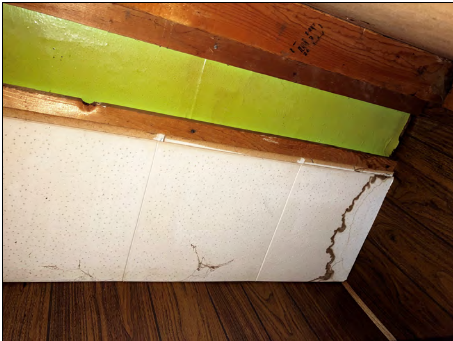
PHOTOGRAPH #22: Paint - Foyer Green (980 ppm Lead )
