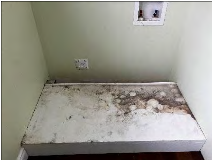
PHOTOGRAPH #28: Organic Growth Observed in Laundry Room
