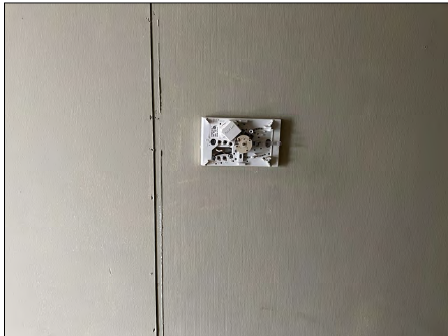
PHOTOGRAPH #8: Non-Mercury Containing Thermostat
