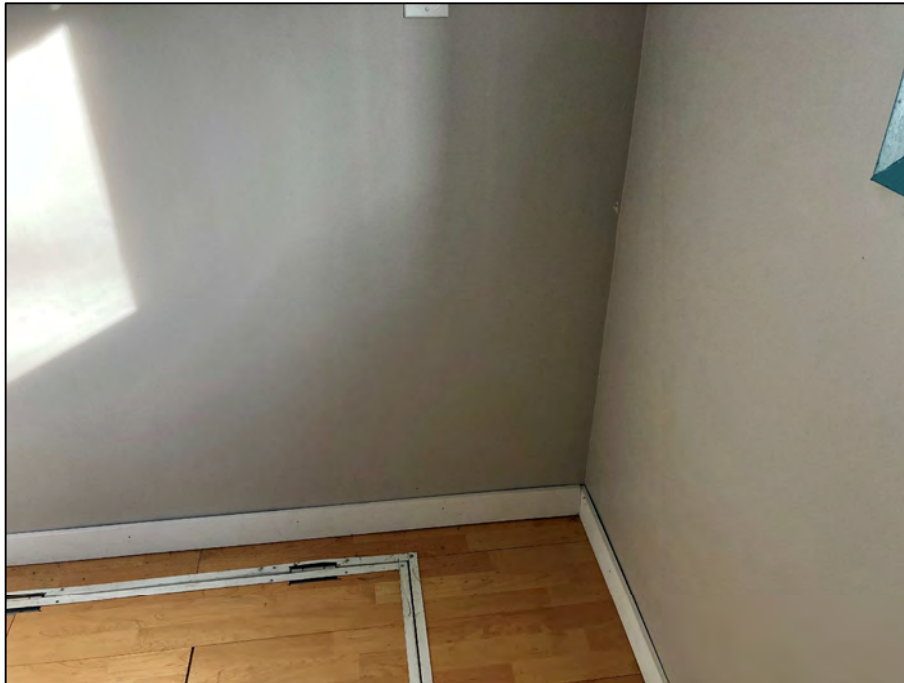
PHOTOGRAPH #5: Drywall Joint Compound - Level 1 Storage Room Exterior (2% Chrysotile)
