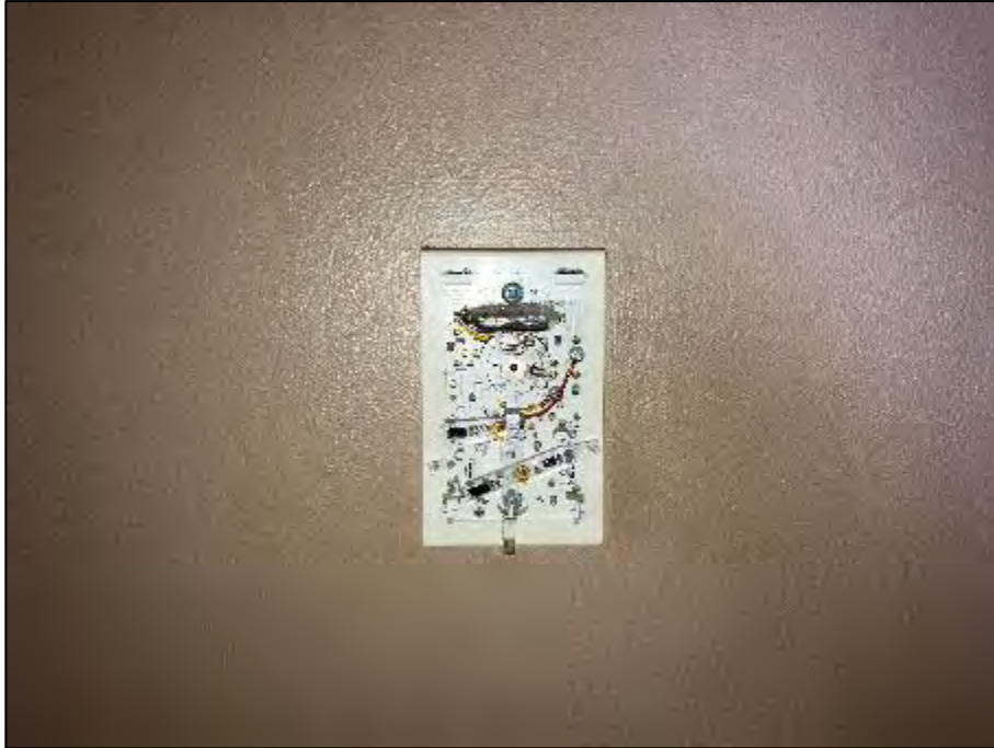
PHOTOGRAPH #36: Thermostat (Mercury)
