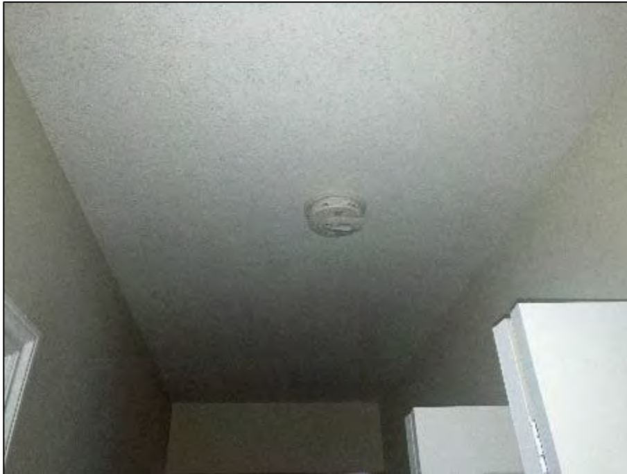
PHOTOGRAPH #27: Smoke Detector in Hallway
