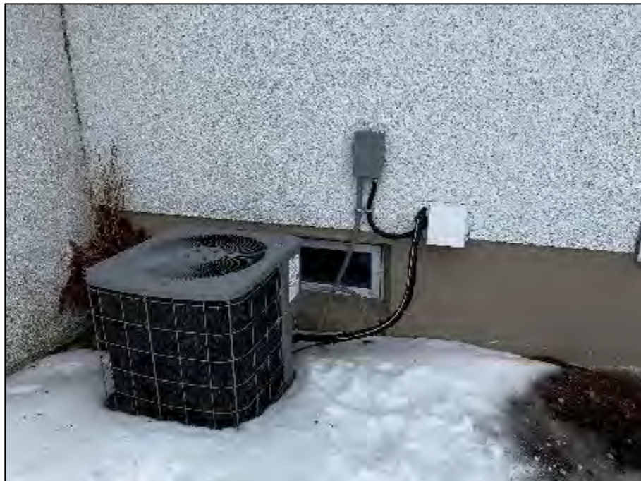
PHOTOGRAPH #35: Air Conditioning Unit on Property
