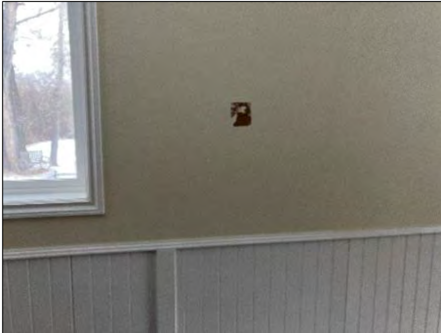
PHOTOGRAPH #21: Paint - Level 1 Dining Room Yellow (<80 ppm Lead)
