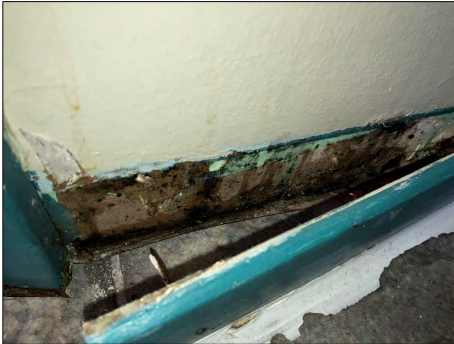
PHOTOGRAPH #28: Organic Growth Behind Bathroom Baseboard
