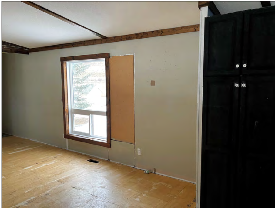
PHOTOGRAPH #7: Paint - Kitchen Green (<80 ppm Lead)
