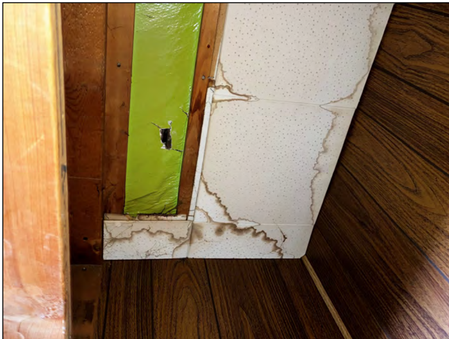
PHOTOGRAPH #29: Water Damaged Ceiling Tile in Foyer
