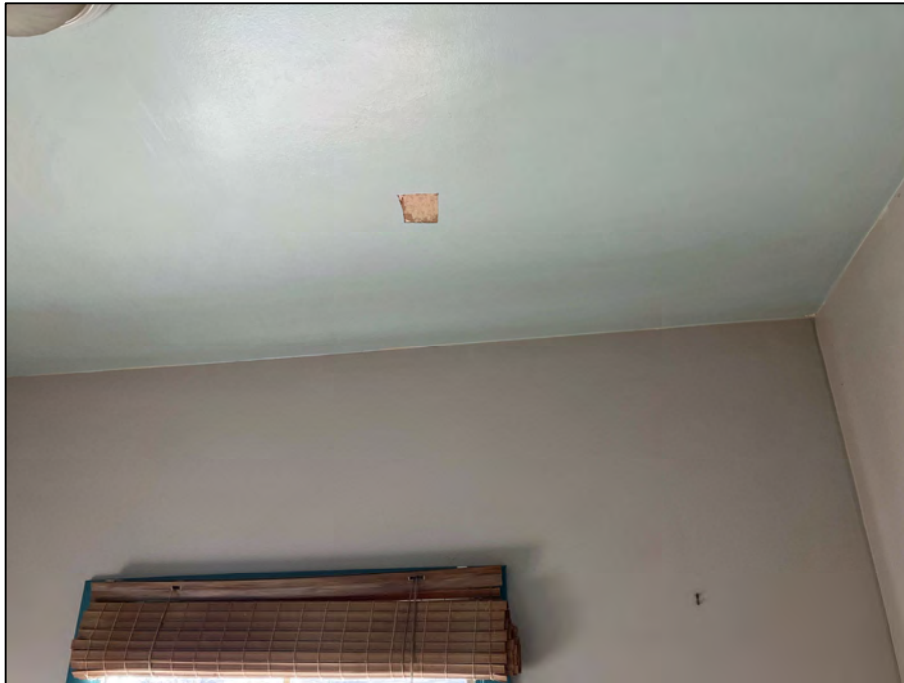
PHOTOGRAPH #19: Paint - Storage Room Green (640 ppm Lead)
