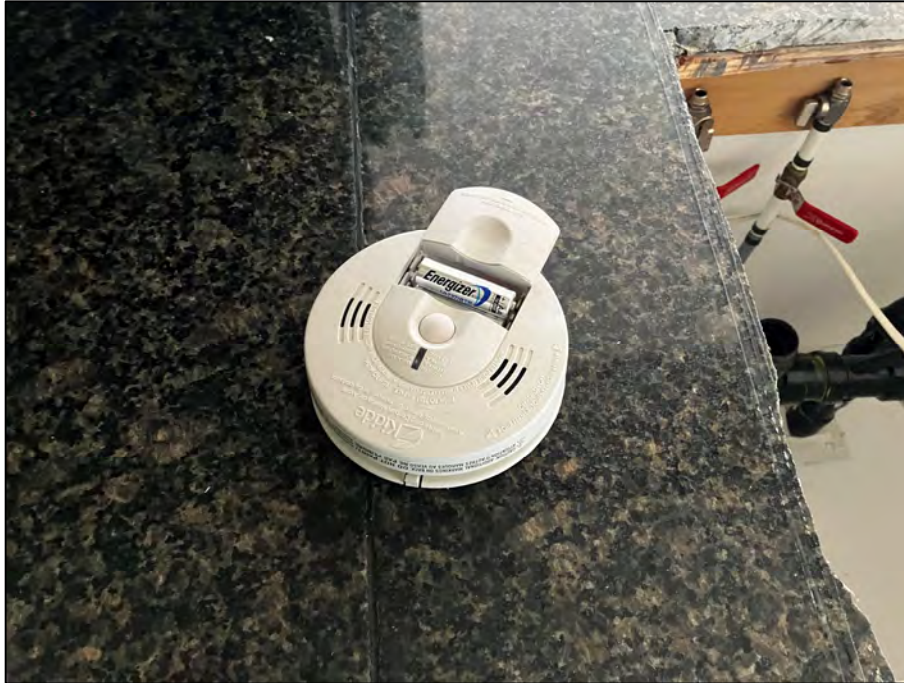
PHOTOGRAPH #9: Smoke Detector in Kitchen
