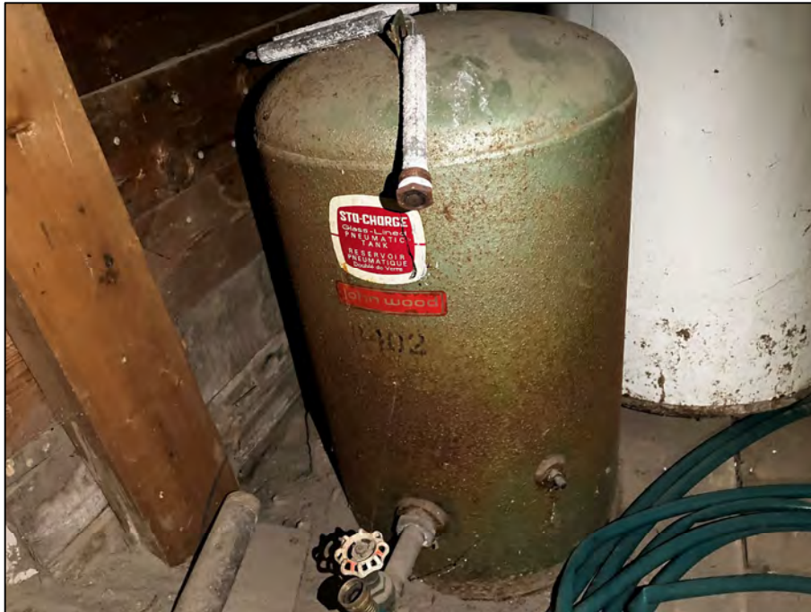
PHOTOGRAPH #24: Pneumatics Storage Tank in Basement
