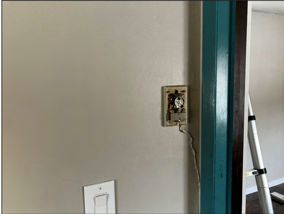
PHOTOGRAPH #30: Mercury Thermostat
