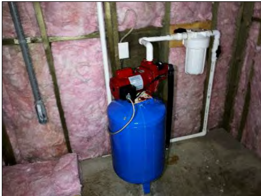
PHOTOGRAPH #26: Basement Sump Pump
