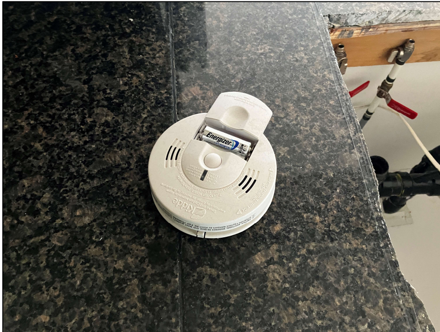
PHOTOGRAPH #9: Smoke Detector in Kitchen
