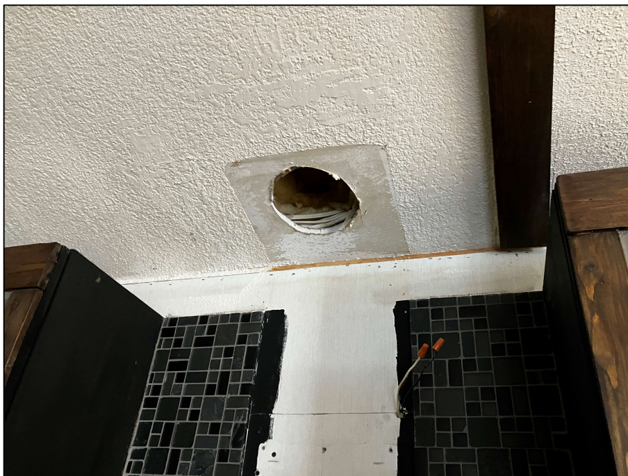
PHOTOGRAPH #17: Kitchen Ceiling Penetration into Attic Space
