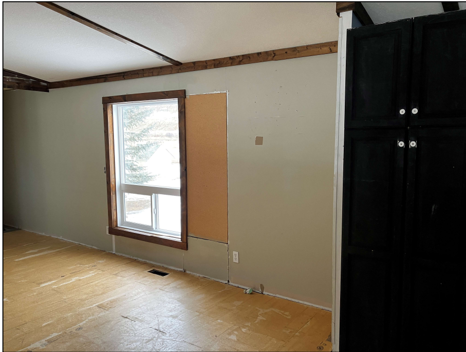
PHOTOGRAPH #7: Paint - Kitchen Green (<80 ppm Lead)
