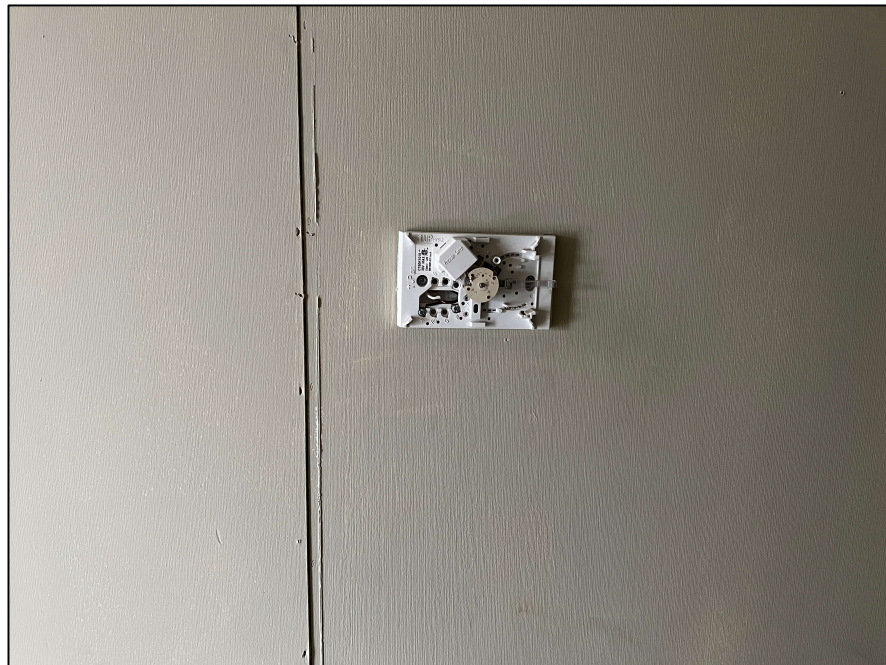
PHOTOGRAPH #8: Non-Mercury Containing Thermostat
