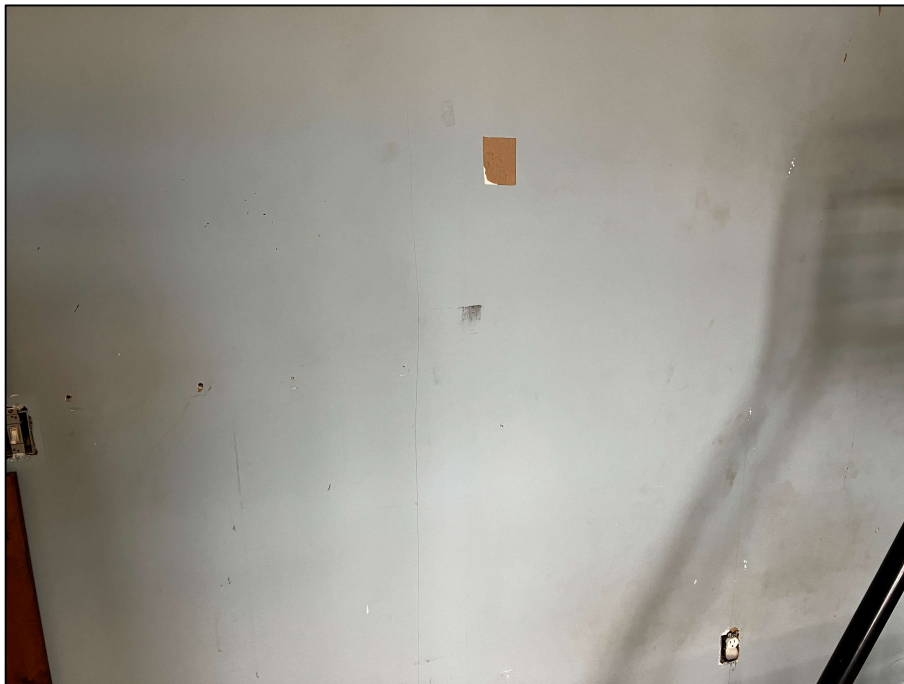
PHOTOGRAPH #6: Paint - N Bedroom Pale Blue (<80 ppm Lead)
