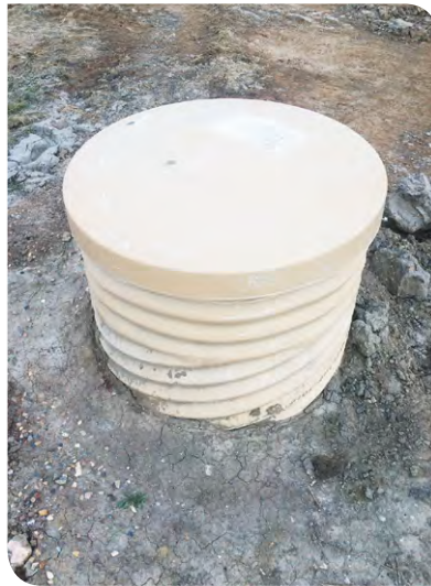
Figure 3-11, Bored Well Cover
