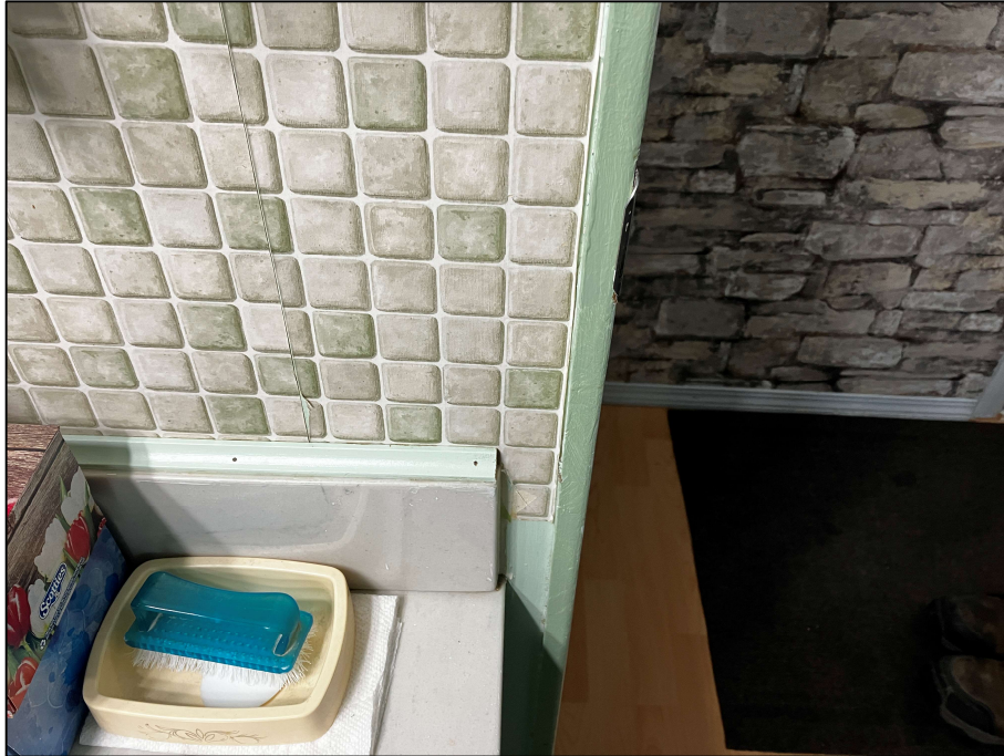
PHOTOGRAPH #13: Wallpaper - Level 1 Bathroom (None Detected)
