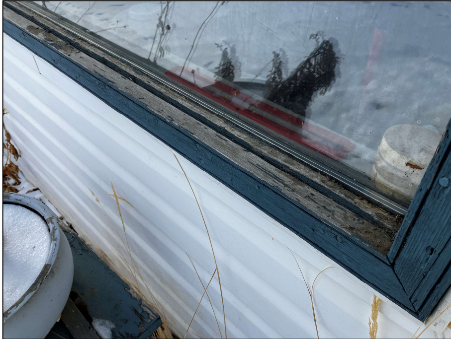
PHOTOGRAPH #25: Paint - Exterior Window Turquoise (<80 ppm Lead)
