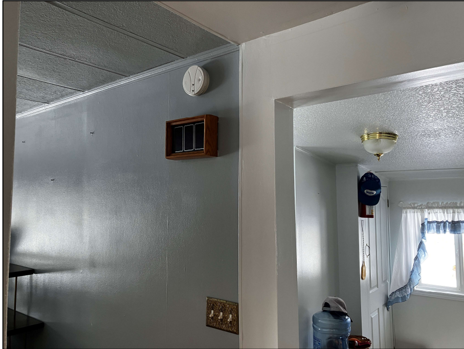
PHOTOGRAPH #30: Smoke Detector in Hallway Near Kitchen
