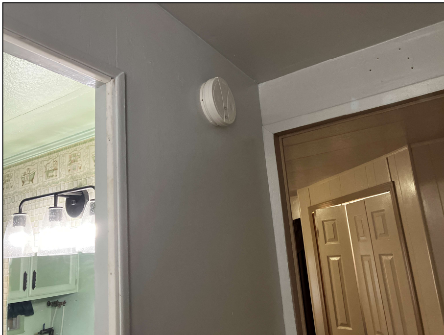
PHOTOGRAPH #31: Smoke Detector in Hallway Near Bedroom
