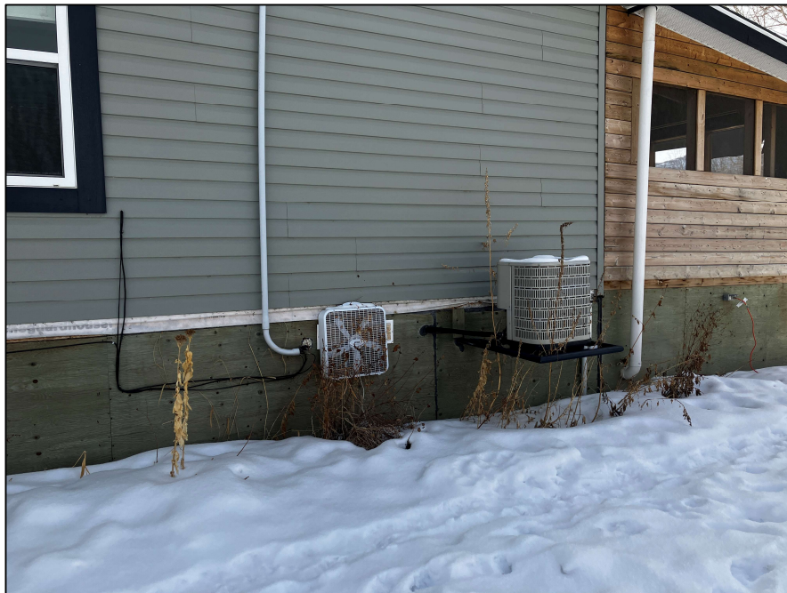
PHOTOGRAPH #8: Air Conditioning Unit on the Exterior of the Home
