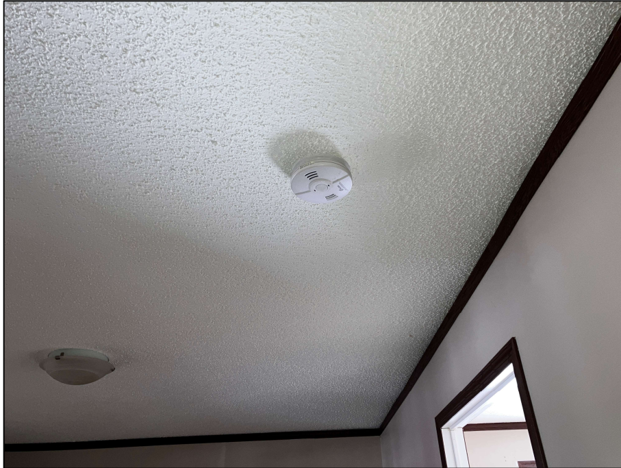
PHOTOGRAPH #7: Smoke Detector in Bedroom
