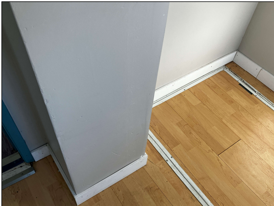
PHOTOGRAPH #4: Drywall Joint Compound - Level 1 Storage Room Interior (Assume Positive)
