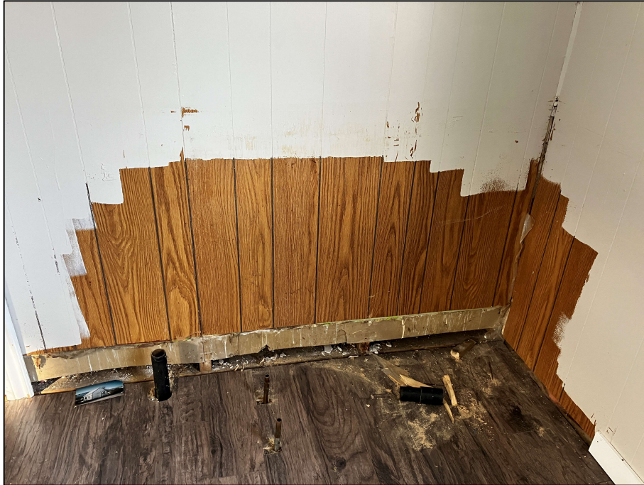
PHOTOGRAPH #1: Drywall Joint Compound - Level 1 Main Room Interior (Assume Positive)
