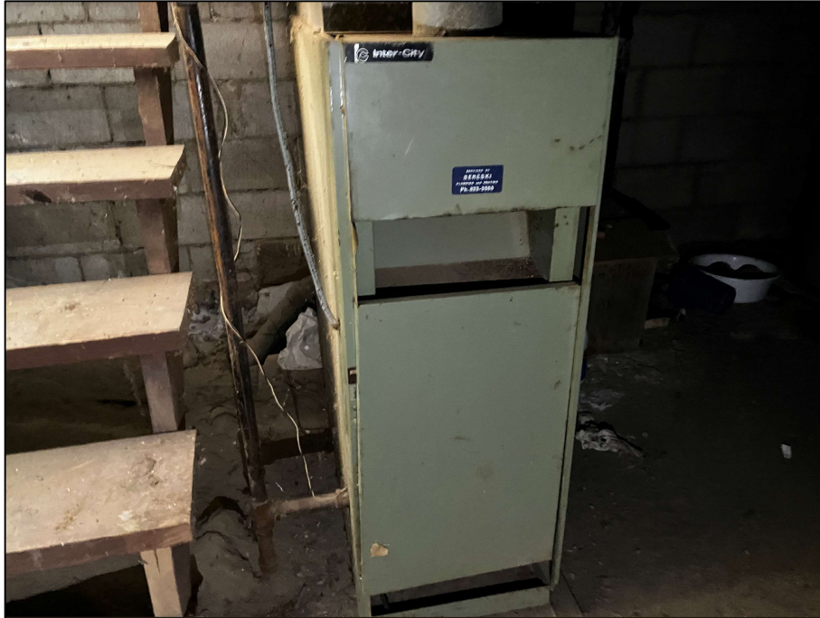
PHOTOGRAPH #26: Furnace Unit Within Basement
