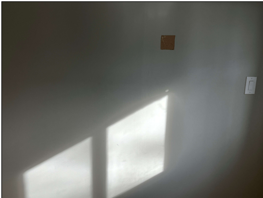
PHOTOGRAPH #18: Paint - Storage Room Beige (570 ppm Lead)
