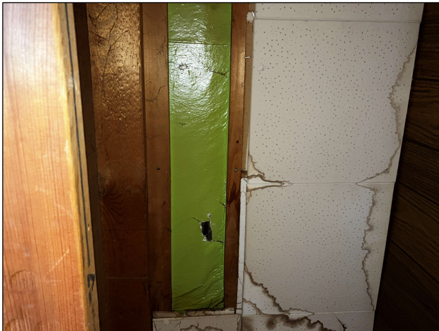
PHOTOGRAPH #6: Drywall Joint Compound - Level 1 Foyer Ceiling (Assume Positive)
