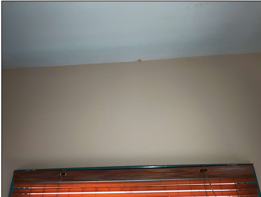
PHOTOGRAPH #7: Drywall Joint Compound - Level 1 Bathroom Ceiling (2% Chrysotile)
