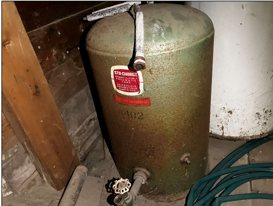
PHOTOGRAPH #24: Pneumatics Storage Tank in Basement
