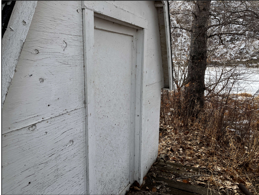
PHOTOGRAPH #21: Paint - Shed White (3400 ppm Lead)
