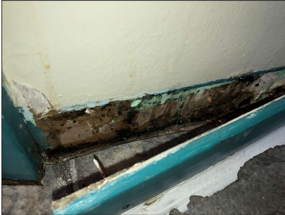
PHOTOGRAPH #28: Organic Growth Behind Bathroom Baseboard
