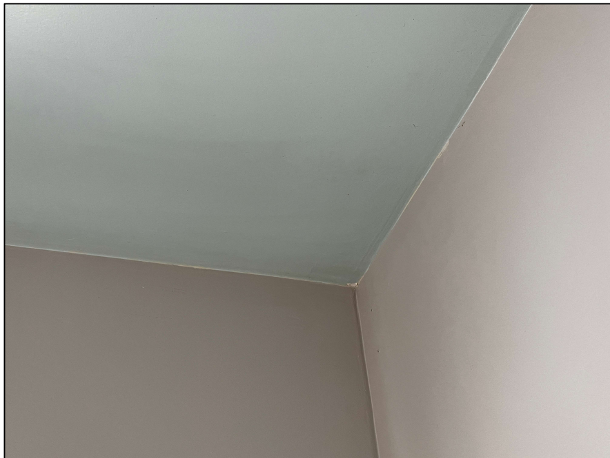
PHOTOGRAPH #8: Drywall Joint Compound - Level 1 Storage Room Ceiling (2% Chrysotile)
