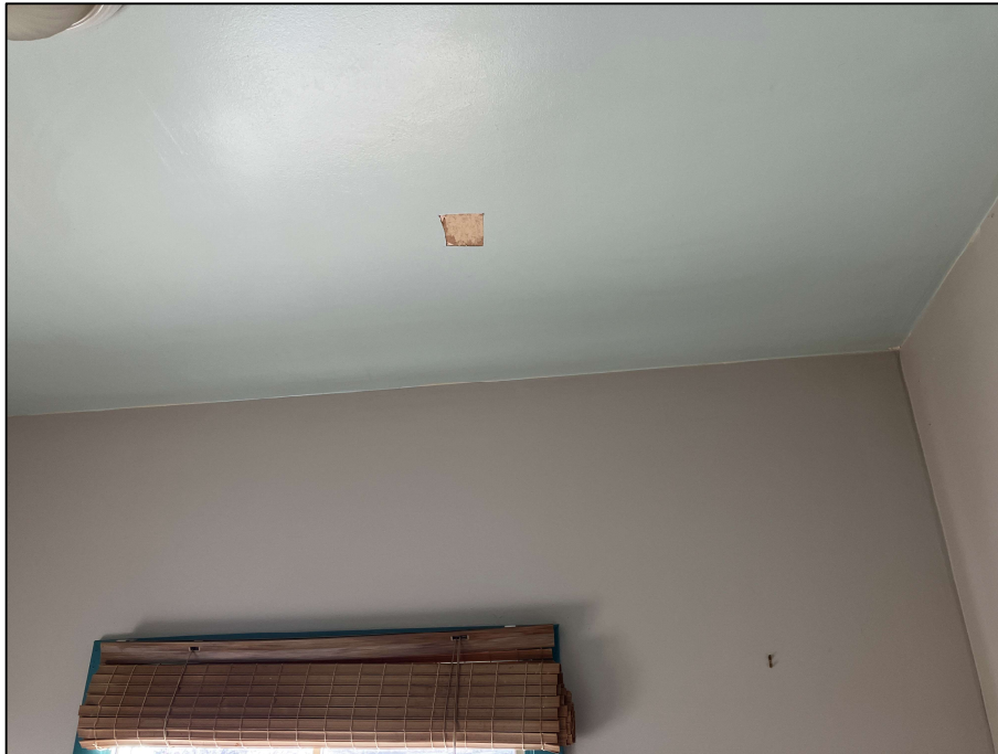
PHOTOGRAPH #19: Paint - Storage Room Green (640 ppm Lead)
