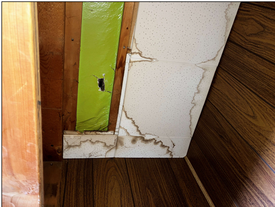
PHOTOGRAPH #29: Water Damaged Ceiling Tile in Foyer
